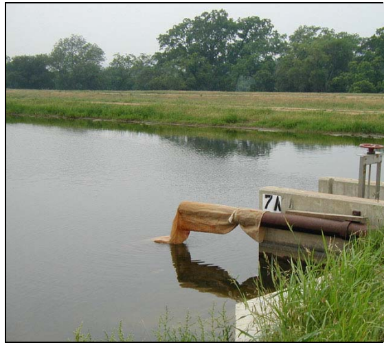
Filtering “sock” on pond water supply line.
