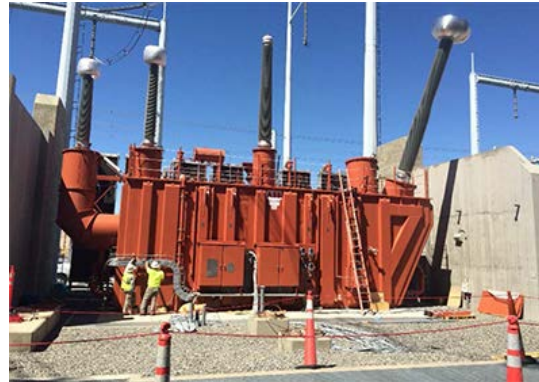
Celilo Converter Station Transformer
