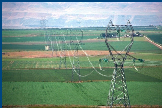
High Voltage Transmission
