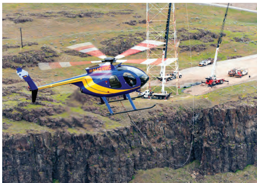
A helicopter removes conductor on the Harvalum–Big Eddy line as part of BPA's 500-kV Big Eddy–Knight project. Crews must remove the conductor to prepare for the construction of one of the towers supporting the Big Eddy–Knight line as it crosses the Columbia River.
