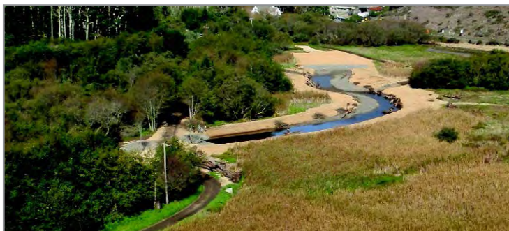
Photos of the Redwood Creek channel alignment and off-channel pond complex, including construction of 5502 feet of new channel, an off-channel point within the flood plain, and the removal of a levee road.
