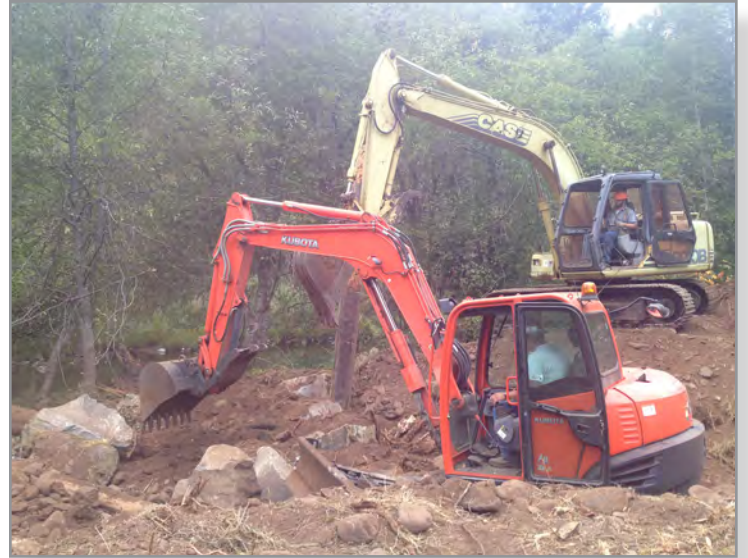
At work in their watershed: local contractors carefully excavate for a buried bank log jam. Photo: Cow Creek Umpqua Tribe
