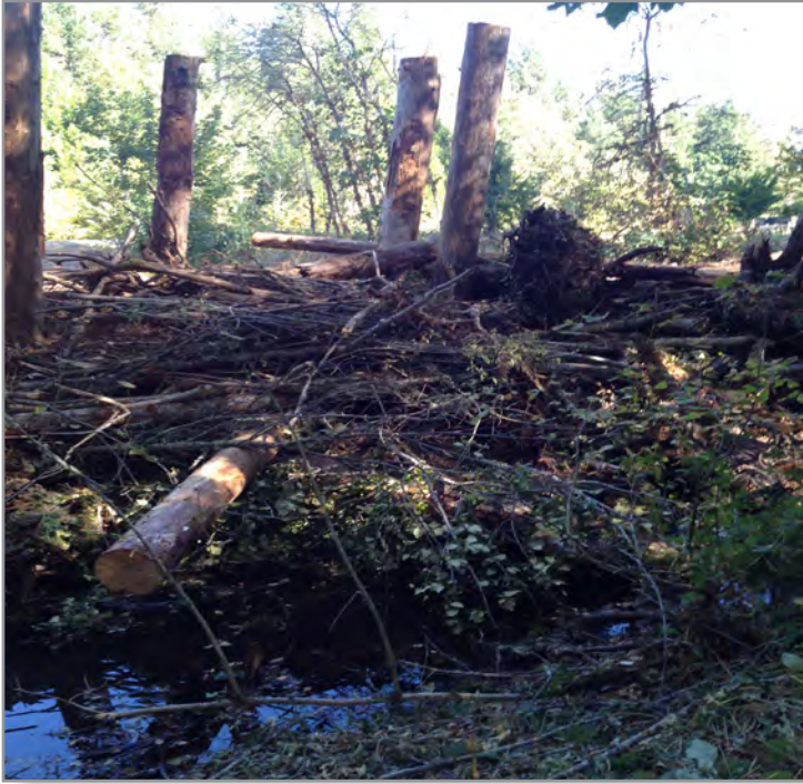
Completed buried bank jam on Elk Creek. Photo: Cow Creek Umpqua Tribe
