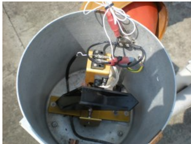
Figure 2. Precipitation Gauge Tipping Mechanism and Wiring.
