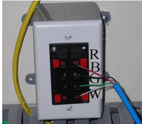
Figure 3. Wall station connecting sensor to data logger
