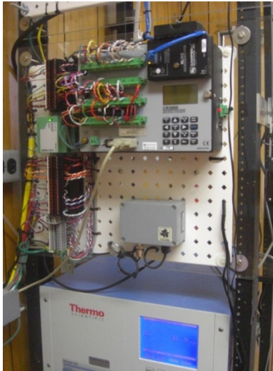
Figure 3 DAS System: Rack Mounted Data logger Backplane
