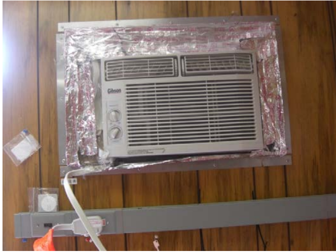
Figure 35. Typical CASTNET Air Conditioner (Note that unit is plugged into outlet directly below. This outlet is switched on and off by the temperature control system.)
