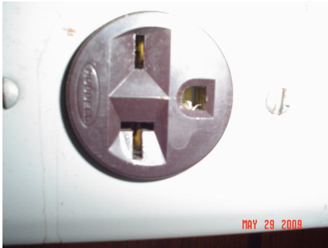
Figure 37. 220VAC Air-Conditioner Power Outlet
