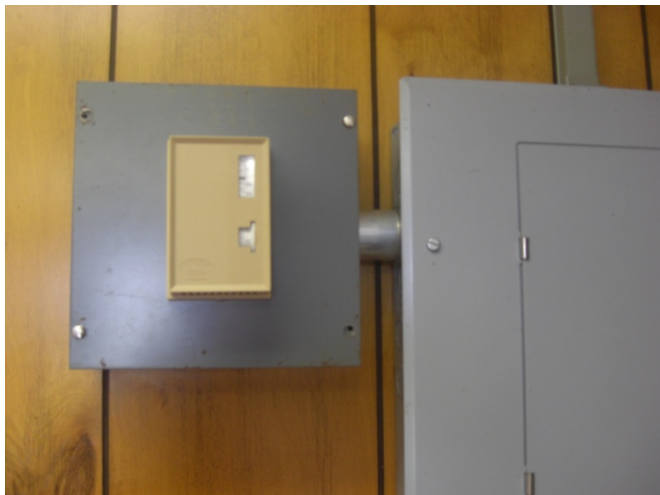
Figure 38. Thermostat Mounted Electrical Box
