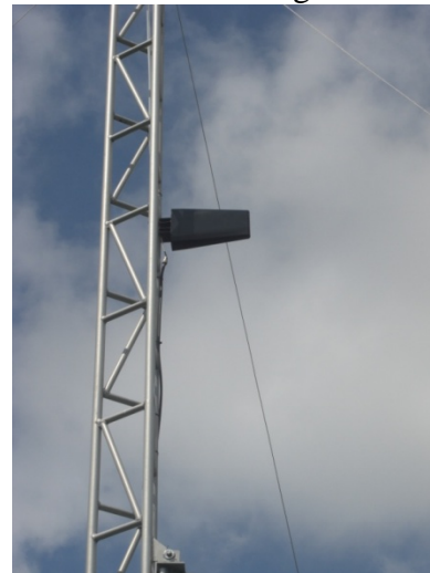
Figure 6. DAS System: Yagi Cellular Antenna Mounted on Folding Tower
