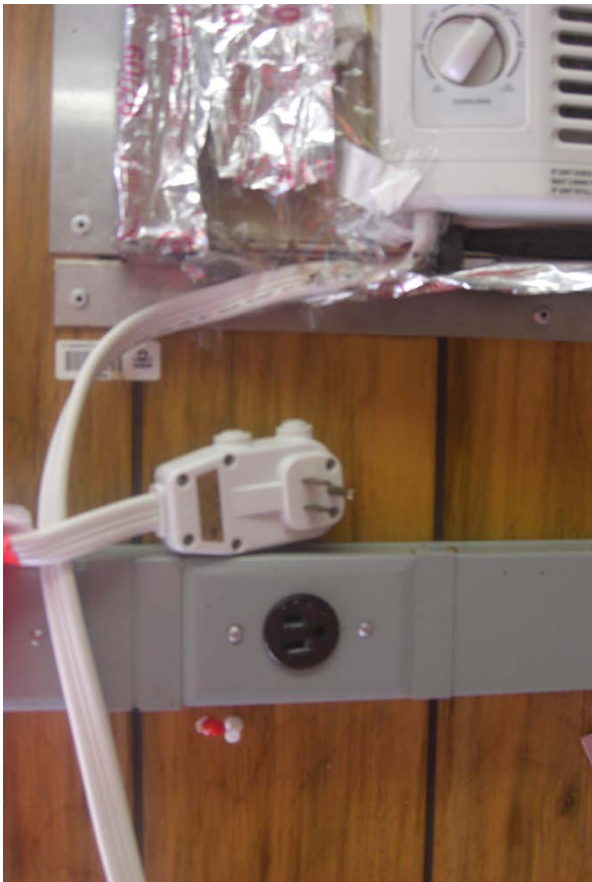
Figure 36. 120VAC Power Outlet switched by temperature control system
