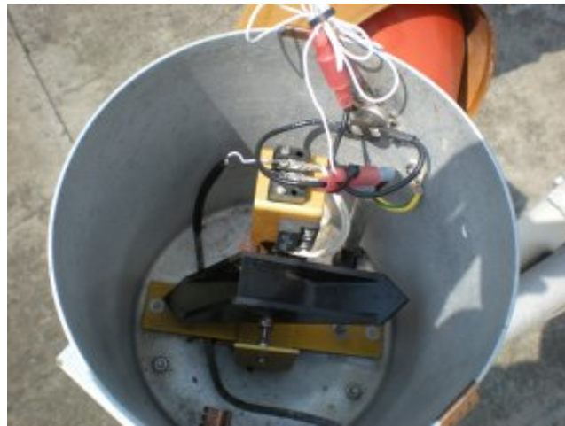
Figure 13. Precipitation Gauge Tipping Mechanism and Wiring.
