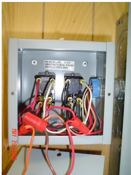
Figure 39. Cover Removed from Thermostat Electrical Box (To show temperature control relays (wired for 220VAC))
