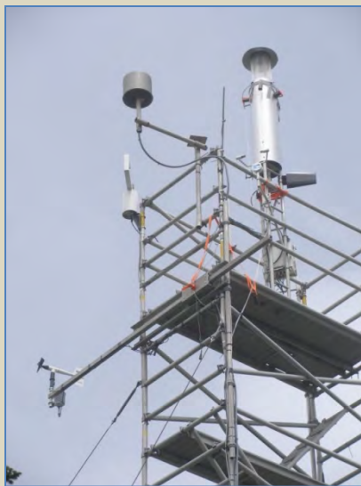
Figure 2e Cloud Water Collector
