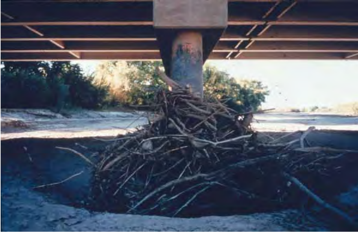
Figure 9.5. Scour at a Coastal Bridge Pier
