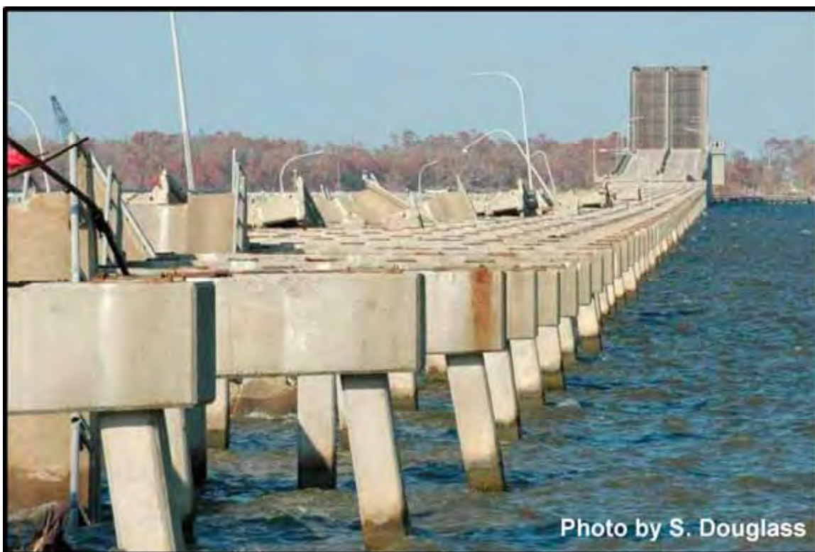
Figure 2.5. US Highway 90 bridge across Biloxi Bay, Mississippi, after Hurricane Katrina. (photo looking northeast from Biloxi 9/21/05).
