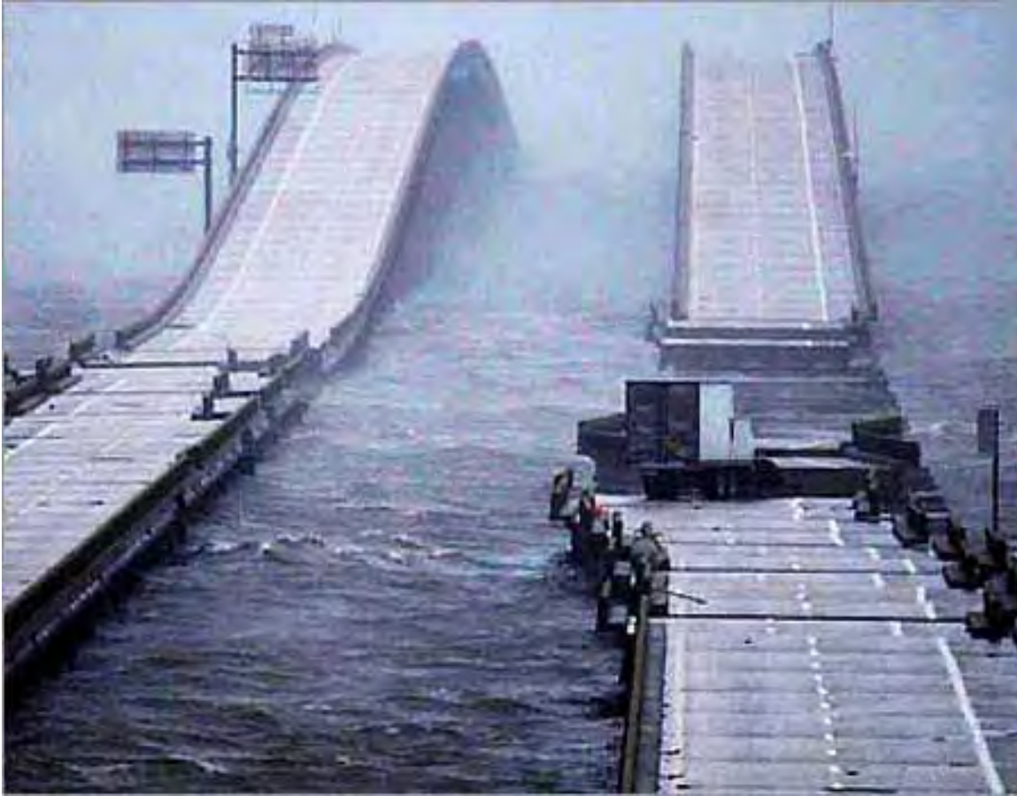
Figure 9.13. Interstate-10 bridge across Escambia Bay, Florida, after Hurricane Ivan. Photo looking east from Pensacola at dawn September 16, 2004. (Pensacola News Journal photo)
