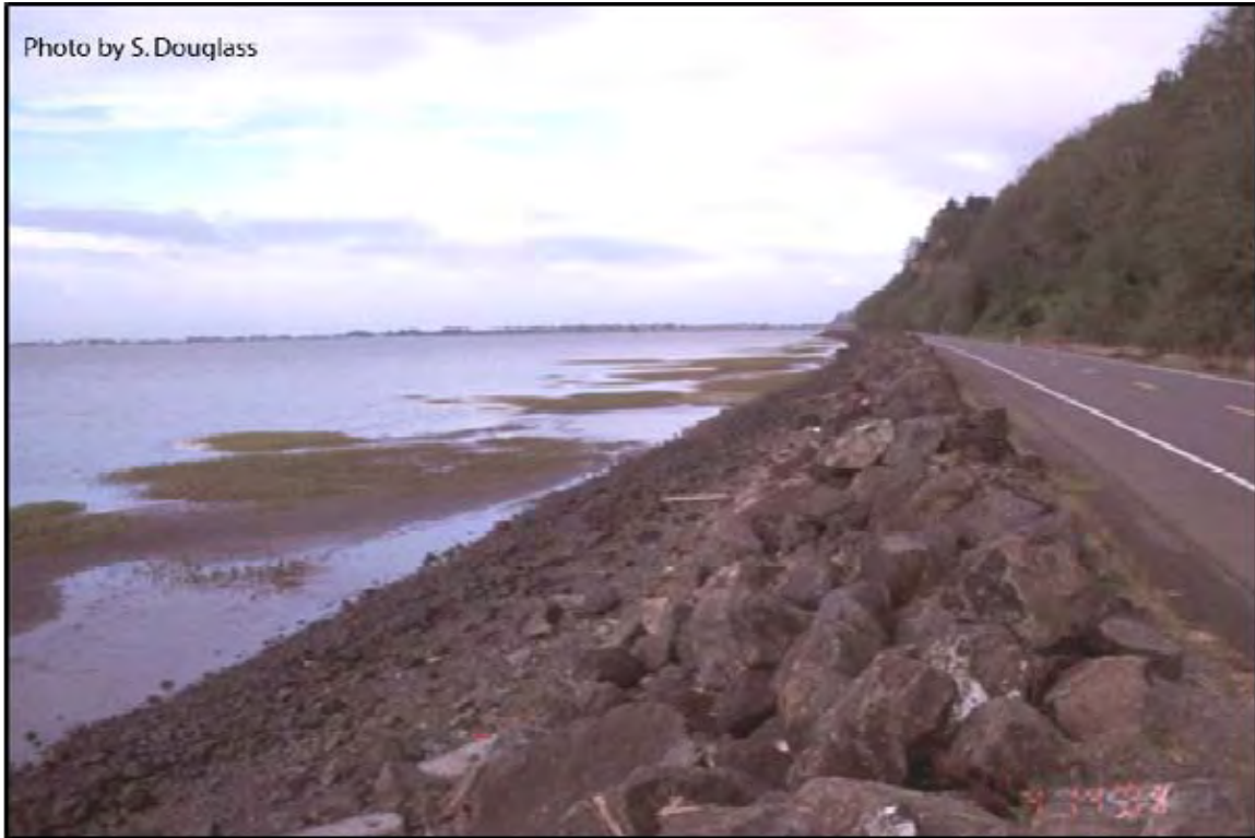
Figure 6.10. Revetment protecting a highway along a bay shoreline. Washington State Route 105, Willapa Bay, Washington (2003)
