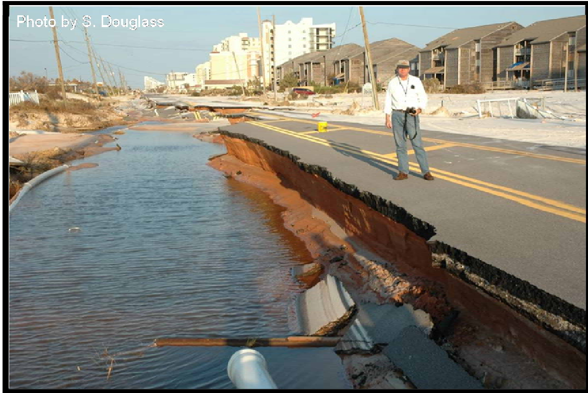
Figure 8.2. Example of pavement damage due to storm surge. Florida 292 on Perdido Key, Florida after Hurricane Ivan (Sept. 2004)
