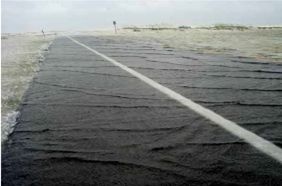
Figure 8.7. Weir-flow damage beginning. (Florida 399, Fort Pickens Road, Gulf Islands National Seashore; July 2005; FHWA photo).
