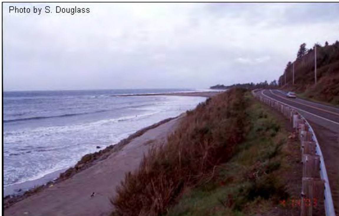
Figure 7.2. A highway initially built inland now threatened by long-term shoreline erosion. Cape Shoalwater area of Washington State Road 105 (2003)
