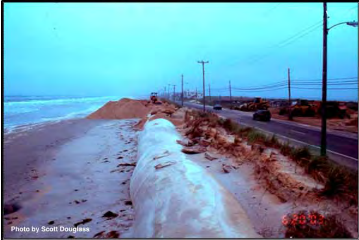
Figure 7.3. A local road threatened by long-term shoreline recession. Ocean Drive, Whale Beach area of Cape May County Road 619, Ludlam Island, New Jersey (2003)
