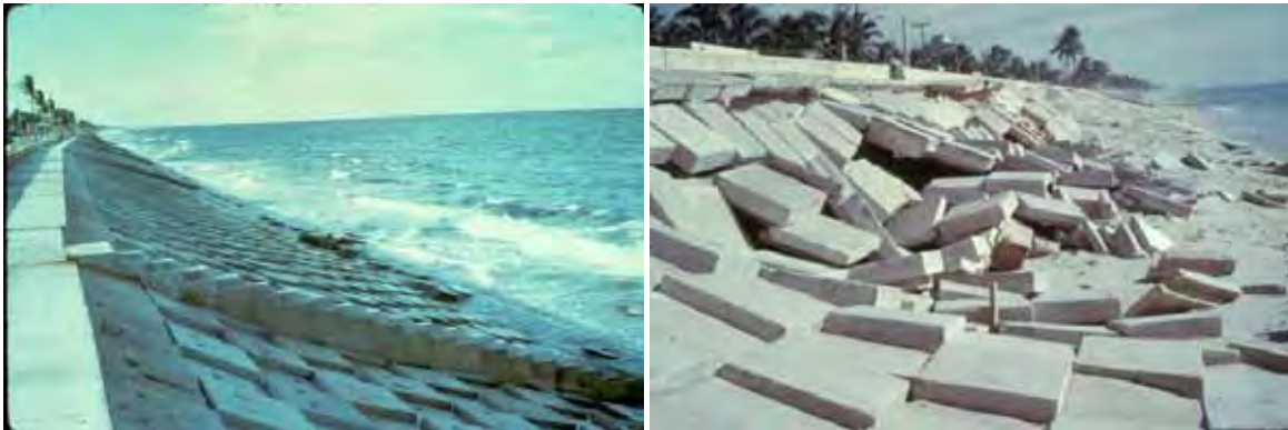
Figure 6.18. Example of rigid concrete-block revetment failure (Florida Highway A1A, Delray Beach, circa 1972; University of Florida and USACE archive photos)
