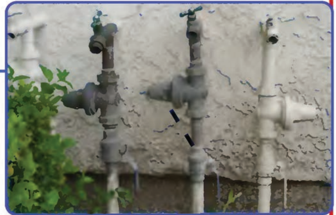
The master valve to a condominium or apartment may be more difficult to locate because several may be grouped together.
