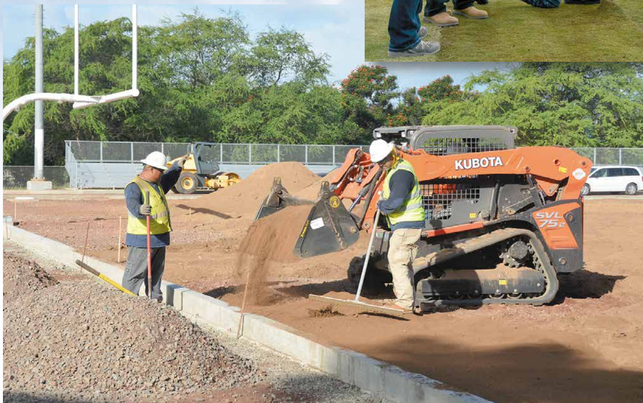
Navy's contractor, Cape Environmental Management Inc., began scraping vegetation and weeds and placing new topsoil on Radford High School's football field the week of Feb. 8. Approximately 800 tons of topsoil will be placed on the field prior to laying 80,000 sq. ft. of sod.
