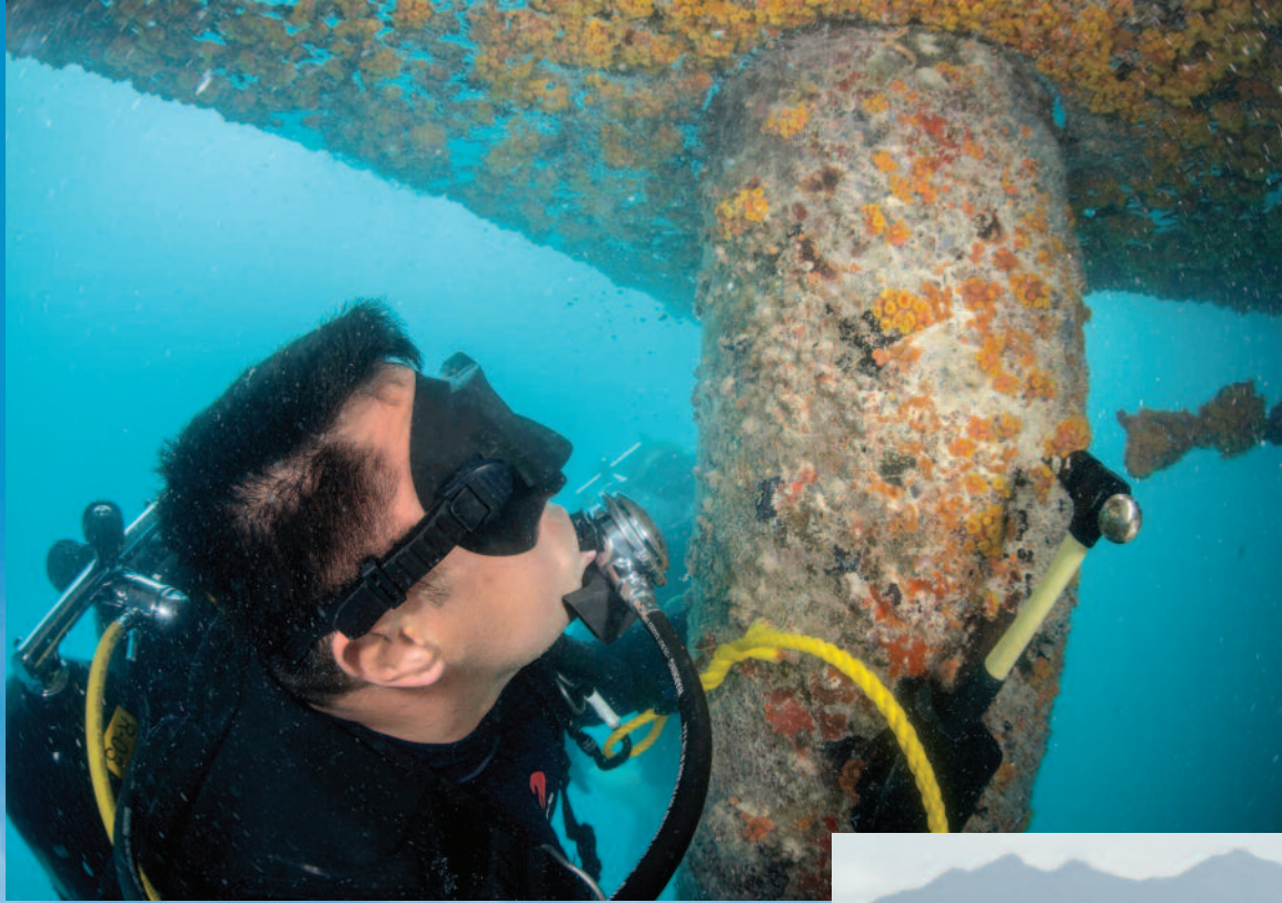
Builder 1st Class Donald Wedekind, Seabee diver from Underwater Construction Team Two, Port Hueneme, Calif., checks the density of piles during a survey on a deep draft wharf at U.S. Navy Support Facility Diego Garcia. During the survey Jan. 19, Seabees from Underwater Construction Team Two, Port Hueneme, and Navy divers from Mobile Diving and Salvage Unit One, Pearl Harbor are checking fenders and piles on the wharf to ensure they are structurally sound.
