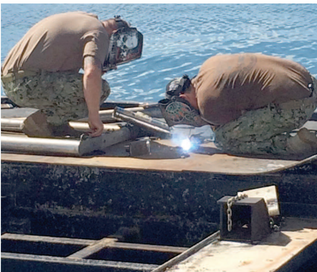
(Left) Seabees weld the dock to the USS Arizona Memorial as they complete repairs. The structure was damaged as the USNS Mercy departed JBPHH on May 27.
