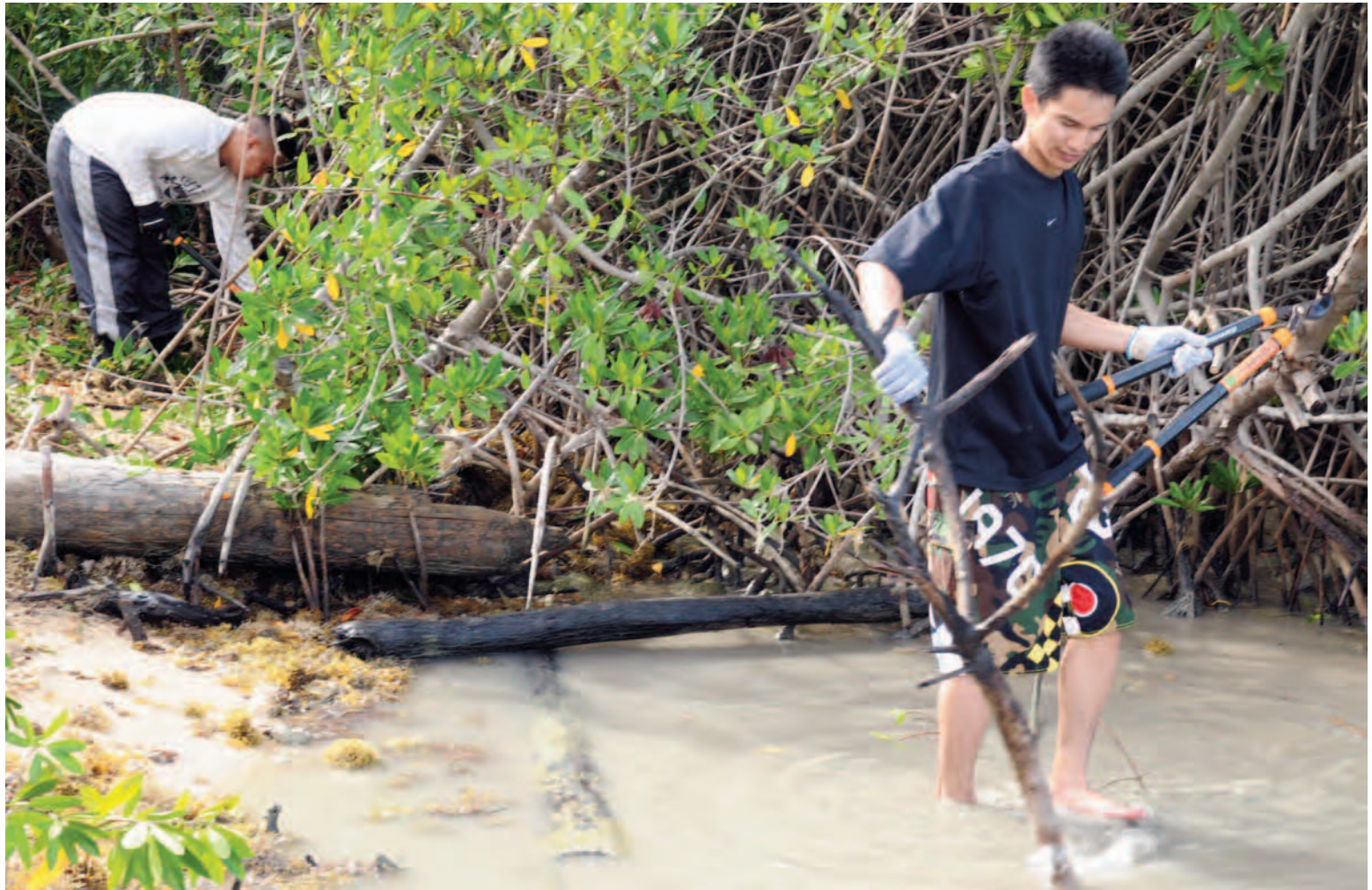
Personnel assigned to Joint Base Pearl Harbor-Hickam (JBPHH) and the 647th Civil Engineering Squadron clear red mangrove off the shoreline of Hickam Beach at JBPHH on Sept. 28. Personnel assigned to JBPHH, 647 CES and Commander, Navy Region Hawaii participated in the cleanup event for National Public Lands Day 2010.
