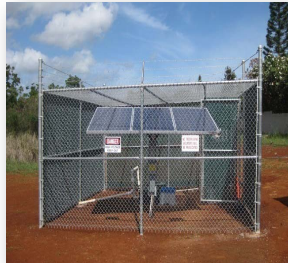
Control unit for successful remediation of fuel at Hickam Petroleum Pipeline Site
