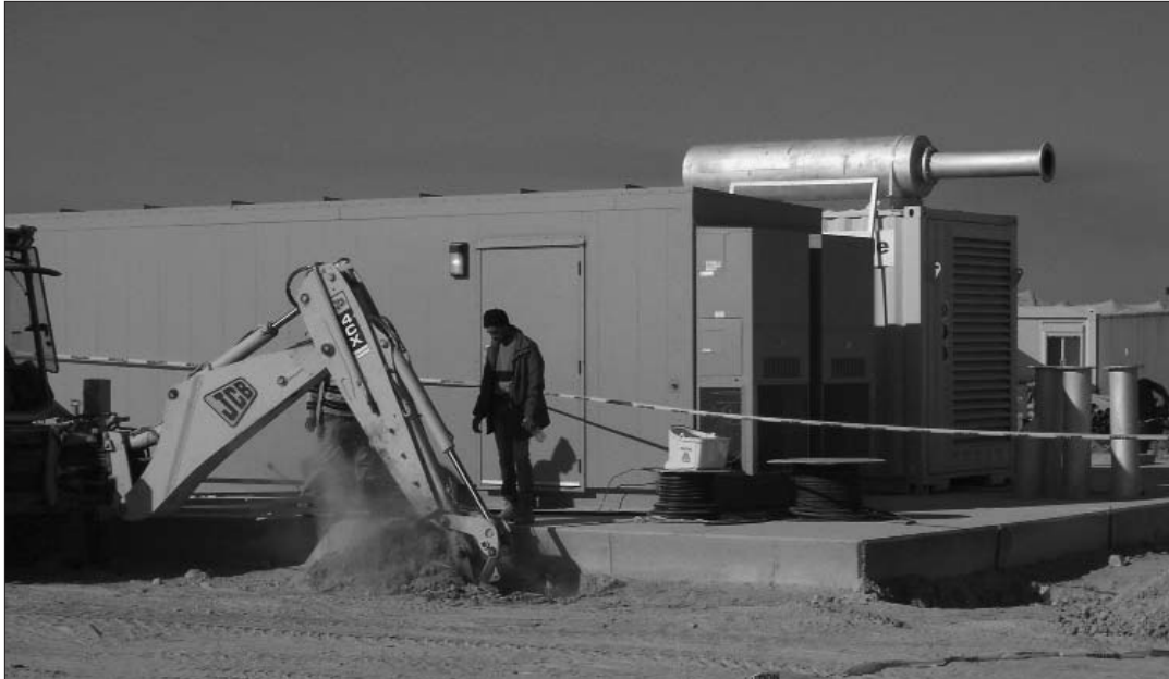
A worker watches the digging for the grounding ring outside one of the four 30-ft transportable shelters that make up the Tech Control Facility at Contingency Operating Base (COB) Speicher, Iraq. Photograph by Cory Hanes
