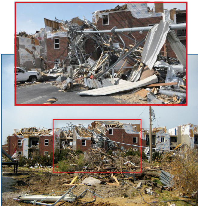
Figure 4: Collapse of a large communications tower onto a building in Joplin, MO (2011 Tornado)
