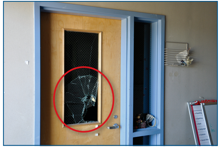
Figure 3: Broken vision panel at an elementary school corridor in Tuscaloosa, AL (2011 Tornado)
