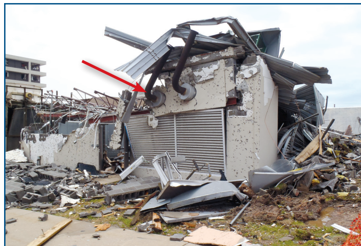
Figure 13: The steel deck/steel joist roof structure and unreinforced CMU walls of this Joplin, MO, building collapsed onto the emergency generator (2011 Tornado)
