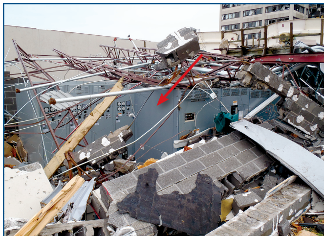
Figure 12: This Joplin, MO, building housing the switchgear (red arrow) and emergency generator (Figure 13) collapsed (2011 Tornado)
