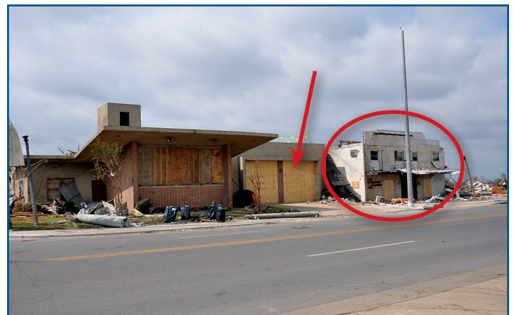
Figure 7: Fire station with a cast-in-place concrete roof deck in Tuscaloosa, AL. The apparatus bay doors (red arrow) collapsed and the adjacent building (red circle) was damaged (2011 Tornado).
