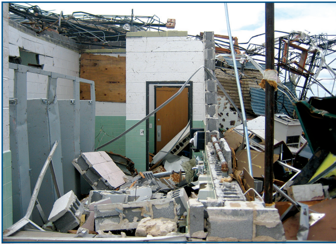
Figure 2: Collapsed concrete masonry unit (CMU) walls at a Joplin, MO, school restroom (2011 Tornado)
