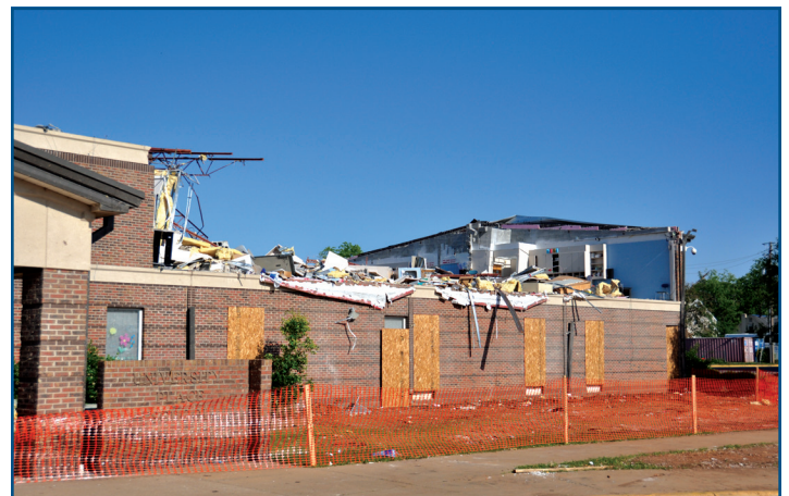
Figure 8: Collapse of the second-floor roof structure, interior walls, and exterior walls of a school in Tuscaloosa, AL (2011 Tornado)
