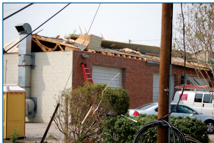
Figure 1: A business damaged by roof damage and water intrusion from a weak tornado
