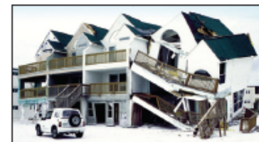
Figure 1. Failure of wood-frame walls used to support a coastal building, which was subjected to shallow flooding, small waves, and floating debris (Fort Walton Beach, FL, Hurricane Opa).
