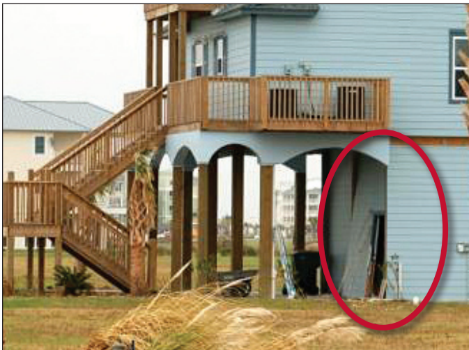
Figure 4. Coastal A-zone flood conditions are sufficient to cause failure of solid breakaway walls and garage doors (west Galveston Island, TX, Hurricane Ike).
