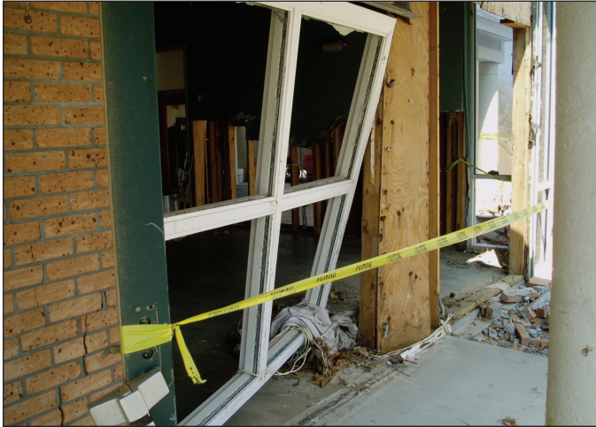
Figure 2. Failure of wood-frame wall, brick veneer, and windows as a result of 4' of stillwater flooding and small waves (Bay St. Louis, MS, Hurricane Katrina).
