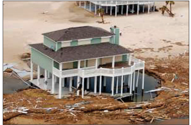
Figure 7. Extreme local scour around a Gulf-front pile foundation (Bolivar Peninsula, TX, Hurricane Ike).
