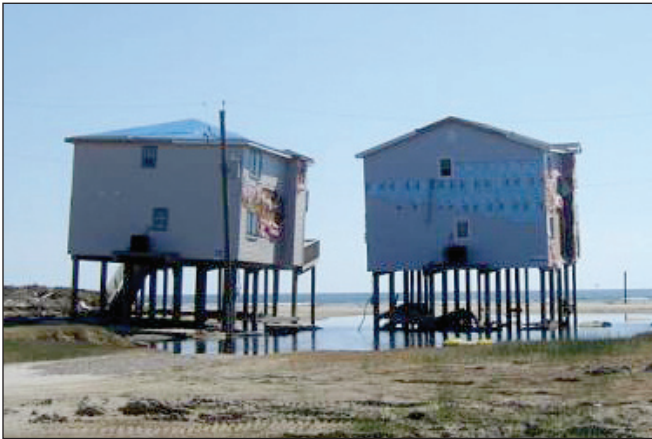
Figure 8. Differential settlement of buildings thought to be a result of inadequate foundation embedment coupled with erosion, scour, and/or soil liquefaction (Surfside Beach, TX, Hurricane Ike).
