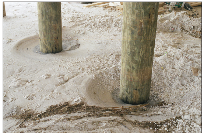
Figure 4. Local scour around foundation piles (Pensacola Beach, FL, Hurricane Ivan).
