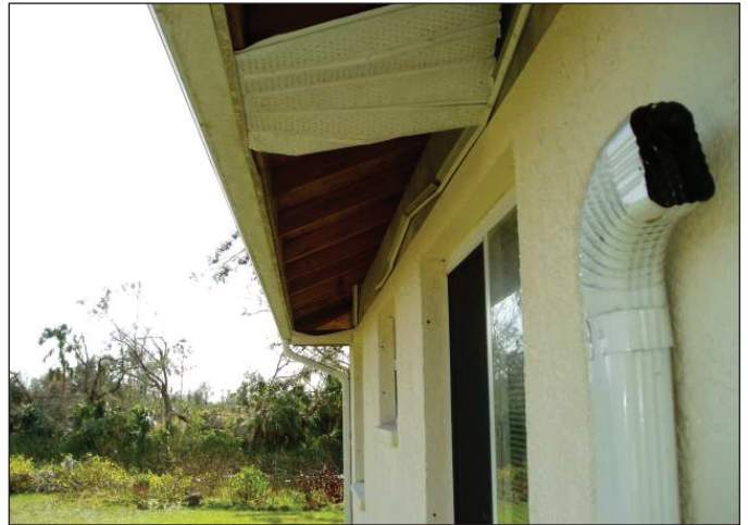
Figure 1. Missing soffit material.
