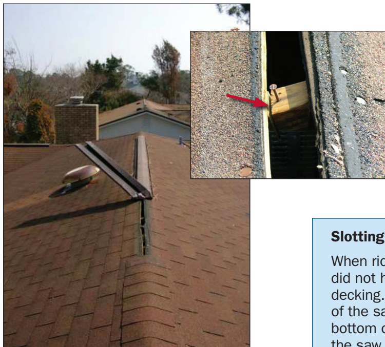
Figure 8. This metal ridge vent was attached with widely spaced roofing nails.
