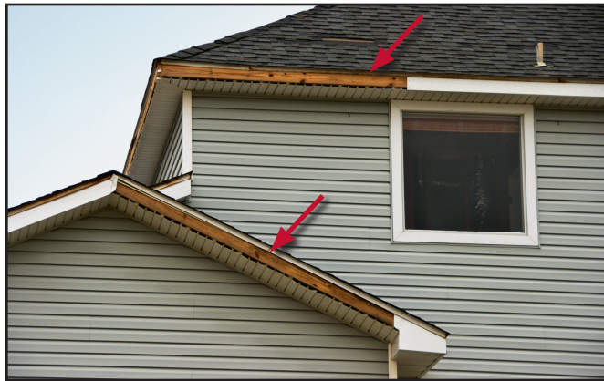
Figure 7. Loss of fascia cover exposes ends of vinyl soffit to direct entry of wind-driven rain.
