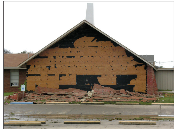
Figure 1. Failed brick veneer over plywood. Many of the ties are still attached to the substrate, but several of the tie fasteners pulled out of the substrate and the ties are embedded in the collapsed veneer. Estimated wind speed: 107 miles per hour (peak gust, Exposure C, at 33 feet).
