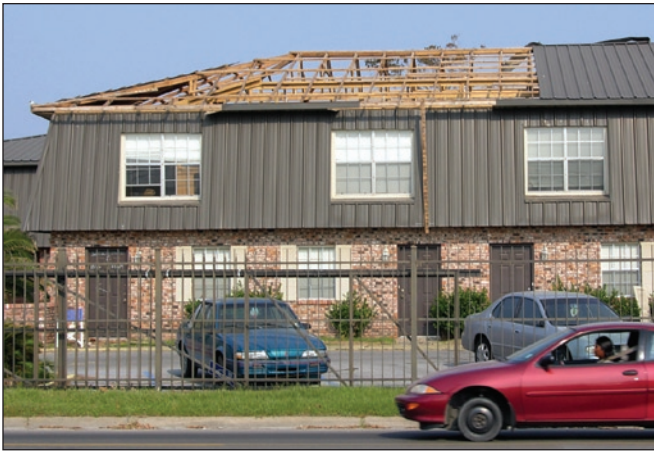
Figure 6. Blow-off of nailers caused these panels to progressively fail. The nailers were installed directly over the trusses. In an assembly such as this where there is no decking, there is no opportunity to incorporate an underlayment. With loss of the panels, rainwater was free to enter the building.
