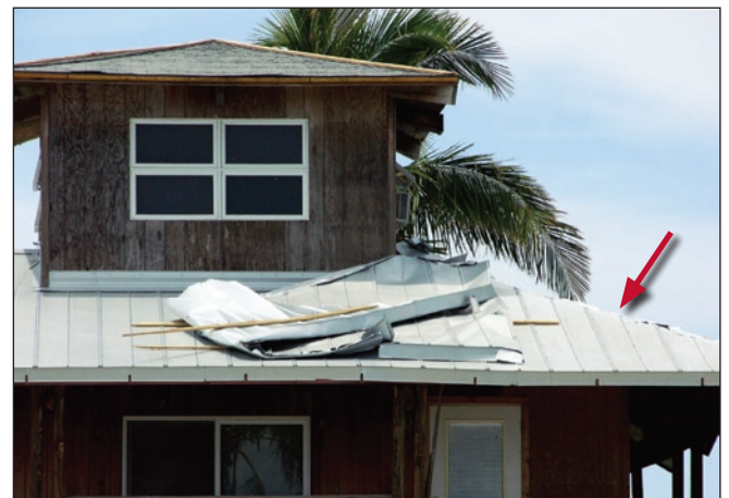
Figure 5. The panels blew off the upper roof and landed on the lower roof of this house. The upper asphalt shingle roof shown had been re-covered with 5V-Crimp panels that were screwed to nailers. The failure was caused by inadequate attachment of the nailers (which had widely-spaced nails) to the sheathing. Note that the hip flashing on the lower roof blew off.
