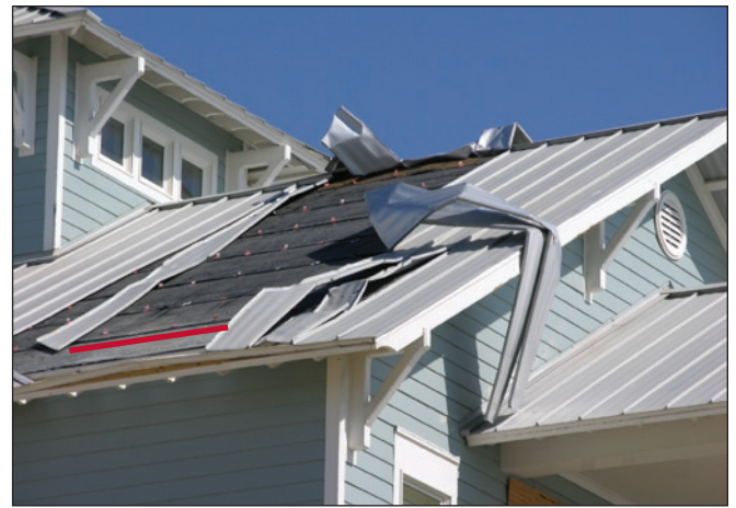
Figure 1. This architectural panel system has concealed clips. The panels unlatched from the clips. The first row of clips (just above the red line) was several inches from the end of the panels. The first row of clips should have been closer to the eave.
