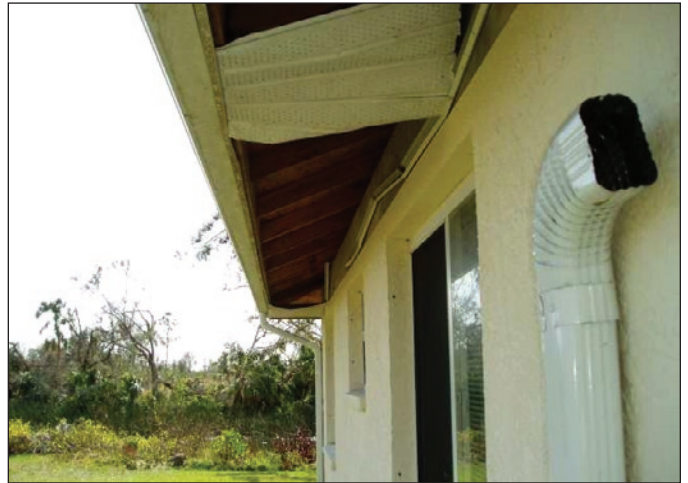
Figure 1. Missing soffit material.
