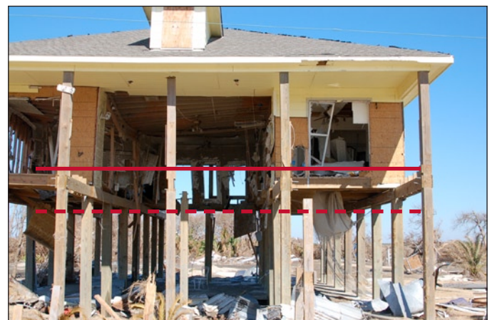
Figure 2. Bolivar Peninsula, TX, V-zone house constructed with the lowest floor (bottom of floor beam) at the BFE (dashed line). The estimated wave crest level during Ike (solid line) was 3 to 4' above the BFE at this location.
