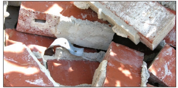
Figure 4. This tie remained embedded in the mortar joint while the smooth-shank nail pulled out from the stud.
