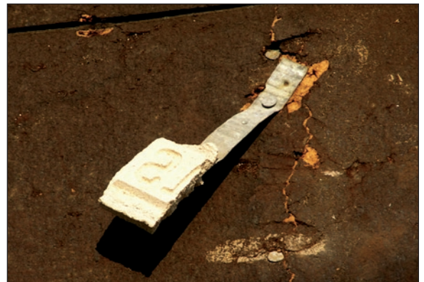
Figure 6. This tie was embedded in the mortar, but the bond was poor.
