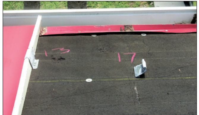
Figure 4. These eave clips were too far from the panel ends. The clip at the left was 13" from the edge of the deck. The other clip was 17" from the edge. It would have been prudent to install double clips along the eave.
