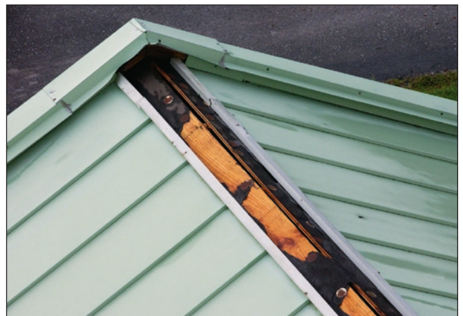
Figure 9. The ridge flashing fasteners were placed too far apart. A significant amount of water leakage can occur when ridge flashings are blown away.
