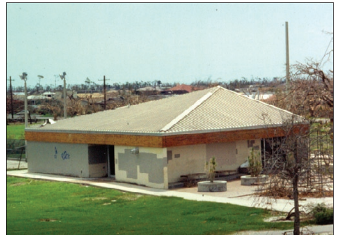
Figure 2. This structural standing seam roof system survived Hurricane Andrew (Florida, 1992), but some hip flashings were blown off. The estimated wind speed was 170 mph (peak gust, Exposure C at 33 feet).
