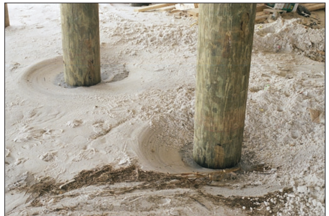
Figure 4. Local scour around foundation piles (Pensacola Beach, FL, Hurricane Ivan).
