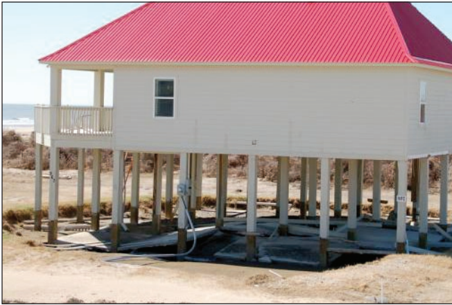
Figure 6. Local scour around a 3rd row house's pile foundation (Bolivar Peninsula, TX, Hurricane Ike).
