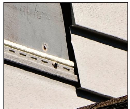
Figure 5. The siding panel was not properly locked into the panel below.
