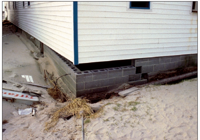
Figure 3. Failure of A-zone type foundation in coastal area, not subject to V-zone conditions (Topsail Island, NC, Hurricane Fran).
