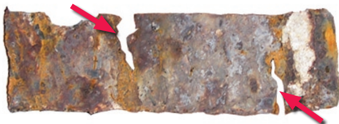
Figure 3. Significant tie corrosion caused the brick at a fire station to fail, even though the building is not near the coast. Note that metal is missing for half of width of the tie at two locations (red arrows). The left end of the tie was still embedded into a concrete masonry unit back-up wall. The right end is where the tie failed in tension, thus leaving a portion of the tie embedded in the collapsed brick.
