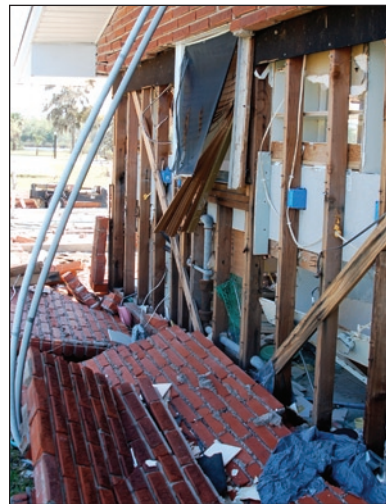
Figure 5. Damage to brick veneer walls due to shallow flooding, floating debris, and small waves. The damaged home was on a sheltered bay shoreline (Baytown, TX, Hurricane Ike).
