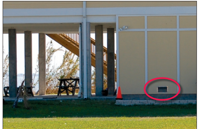
Figure 5. Flood opening in a below-BFE enclosure wall.
