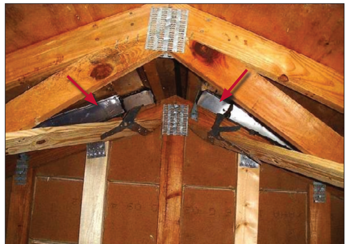
Figure 12. Metal plugs (red arrows) in gable rake vents.
