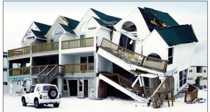
Figure 1. Failure of wood-frame walls used to support a coastal building, which was subjected to shallow flooding, small waves, and floating debris (Fort Walton Beach, FL, Hurricane Opal).
