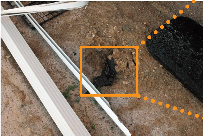
Fractured ABS stabilizer plates may have contributed to the failure of the support system.
