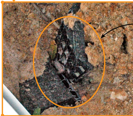
Fractured ABS stabilizer plate
