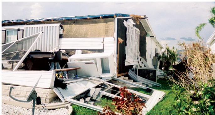
Damage to new manufactured home resulting from improper attachment of a screened enclosure.
