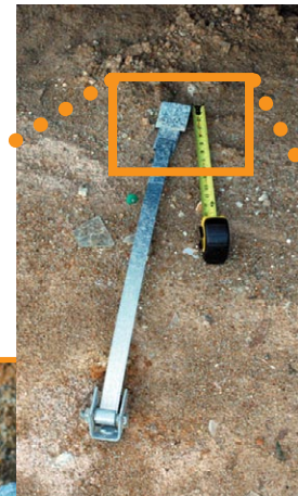
Wall ties that secured the home to ground anchors were torn from the home.
