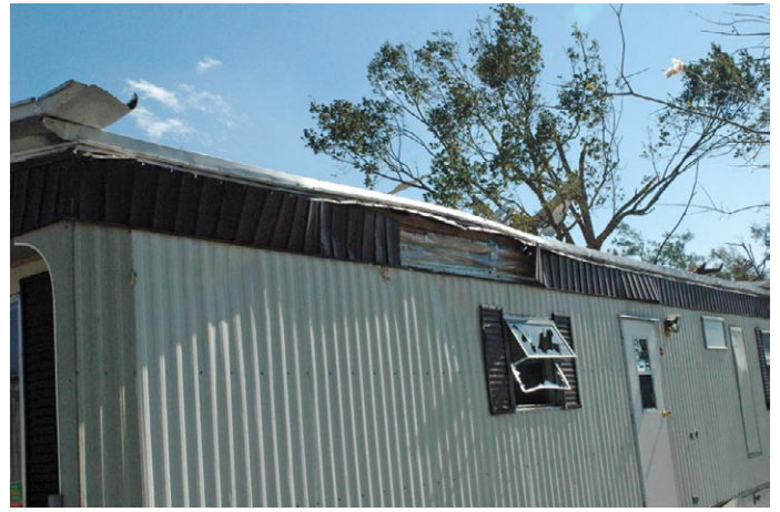
Portions of the roof and wall sheathing of this older manufactured home were lost. Flying debris broke unprotected glass in the doors and windows.
