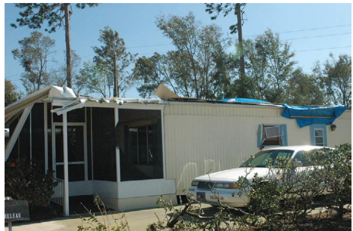
The roof of this older manufactured home was blown off by high winds.
