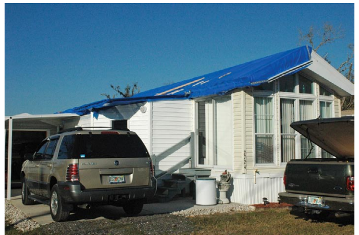
Loss of roofing likely originated where the roof of the addition was fastened to the home's roof.
