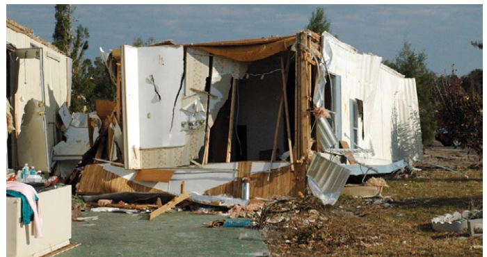
This manufactured home rolled off its foundation after anchors used to secure it pulled out of the ground. Only six anchors (three per side) secured the 30-foot-long section of home. Twelve anchors would have been appropriate. The home lifted off its foundation and rolled approximately 70 feet before coming to a rest on its roof.
