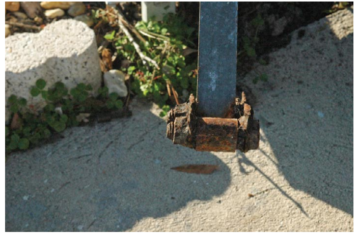
This ground anchor failed just below the anchor head where corrosion had weakened the anchor shaft. Like many older-style anchors and straps, the anchors and straps were not galvanized and were susceptible to corrosion.
