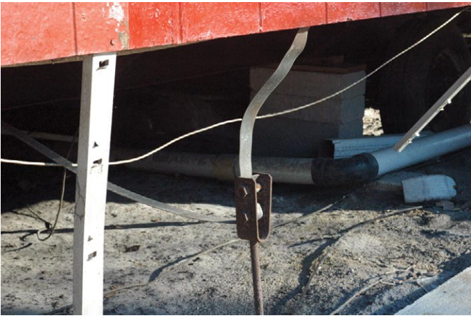
The ground anchor above pulled out of the ground 8 inches. Either improper anchors were selected or too few were installed. The anchor spacing at this home was approximately 12 feet.
