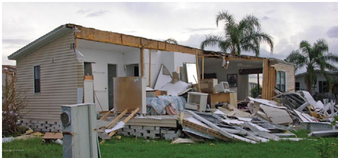
Wind damage to a new manufactured home.
