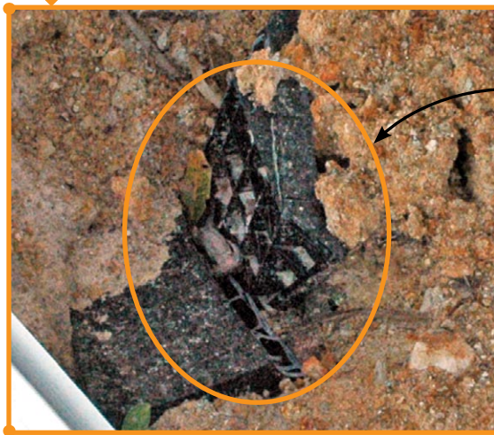
Fractured ABS stabilizer plate
