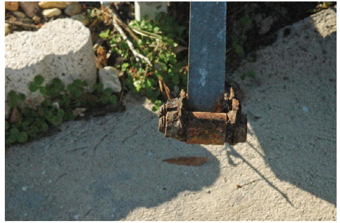
This ground anchor failed just below the anchor head where corrosion had weakened the anchor shaft. Like many older-style anchors and straps, the anchors and straps were not galvanized and were susceptible to corrosion.
