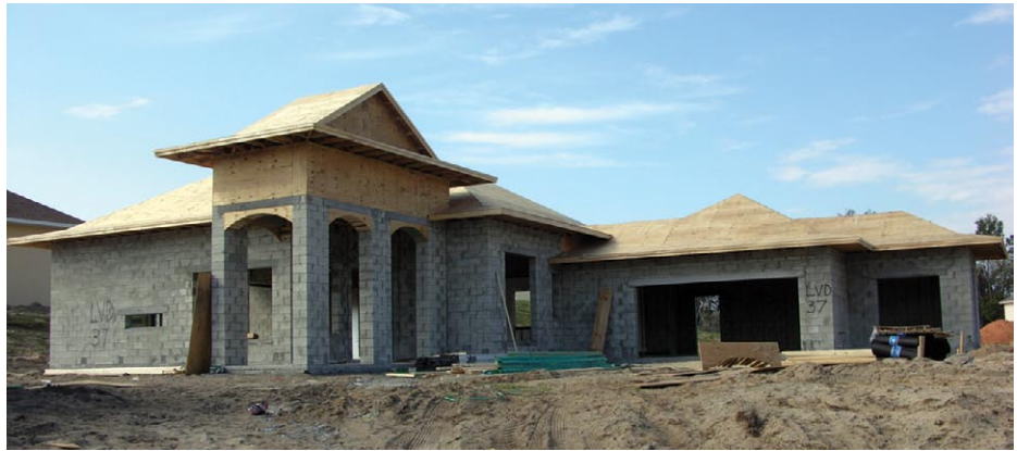
CMU was used for the exterior walls at this house under construction (New Smyrna Beach, FL).
