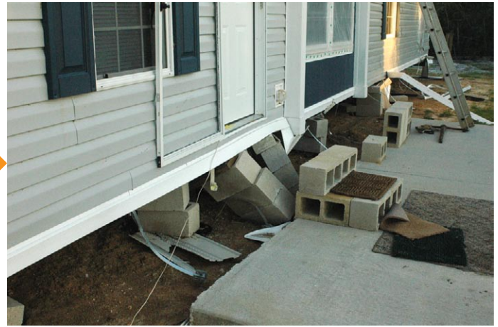
After falling from its supports, the home moved approximately 3 feet.
