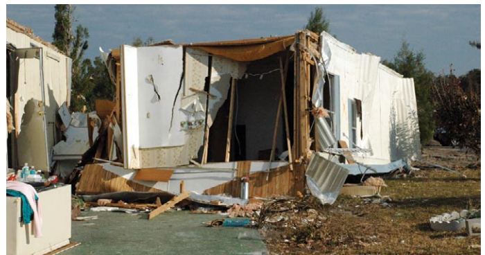
This manufactured home rolled off its foundation after anchors used to secure it pulled out of the ground. Only six anchors (three per side) secured the 30-foot-long section of home. Twelve anchors would have been appropriate. The home lifted off its foundation and rolled approximately 70 feet before coming to a rest on its roof.
