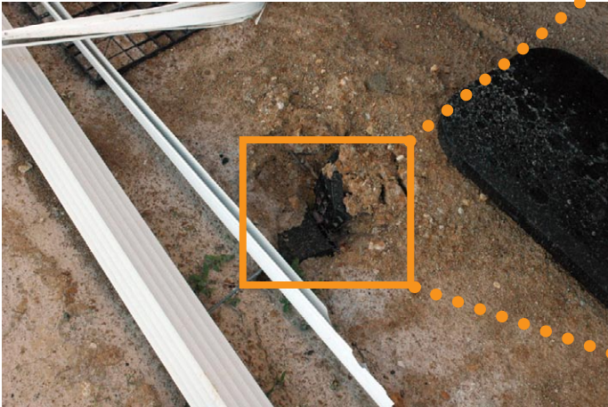
Fractured ABS stabilizer plates may have contributed to the failure of the support system.
