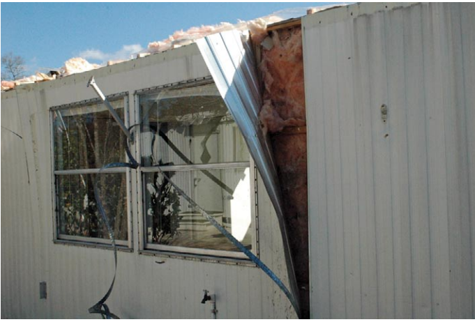
The entire roof structure of this older manufactured home was lost and wall panels were lifted from the home.
