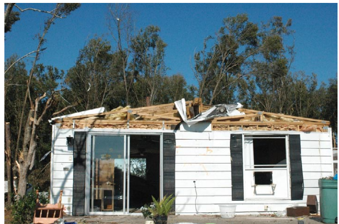
This home, constructed between 1976 and 1994, was severely damaged by one of the February 2007 tornadoes.
