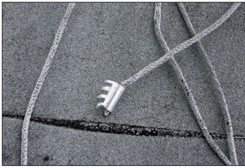
Figure 7. A failed prong-type splice connector. If conductors become detached from the roof, they are likely to pull from pronged splice connectors.
