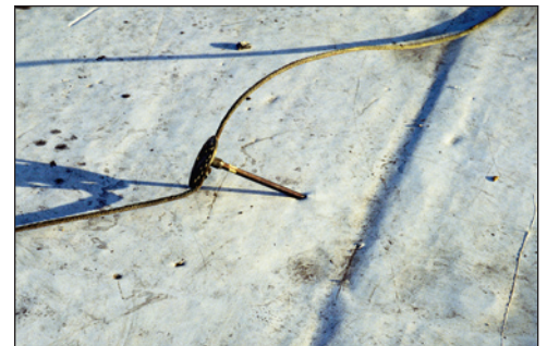
Figure 1. This displaced air terminal punctured the membrane in several locations.
