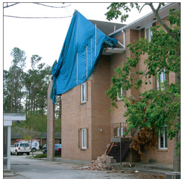
Figure 2. The upper portion of the brick veneer at this apartment building collapsed. Pedestrian and vehicular traffic in the vicinity of the damaged wall were vulnerable to injury and damage if remaining portions of the wall were to collapse during subsequent storms.
