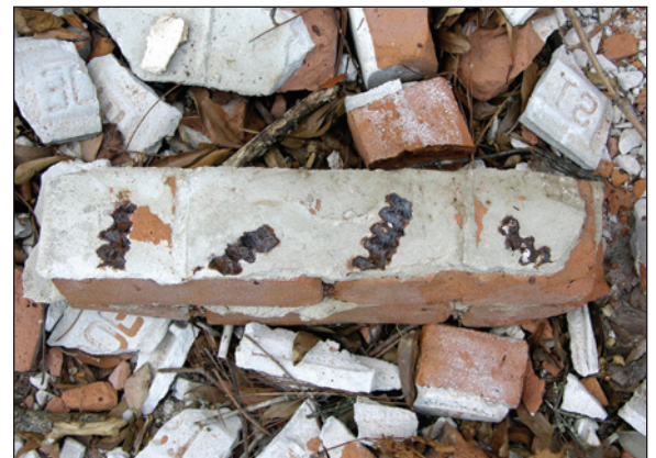
Figure 6. There were several ties in this portion of the wall, but they failed due to severe corrosion.
