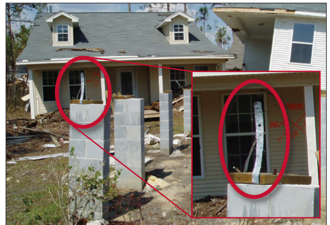
Figure 8. Post-Katrina investigations showed that many buildings were attached to foundation piers with light gauge metal straps. These straps failed in many instances. A stronger (preferably bolted) connection is recommended when attaching Coastal A Zone buildings to their foundations.
