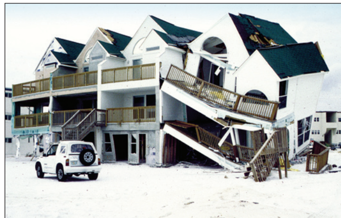
Figure 1. Failure of wood-frame walls used to support a coastal building, which was subjected to shallow flooding, small waves, and floating debris (Hurricane Opal).
