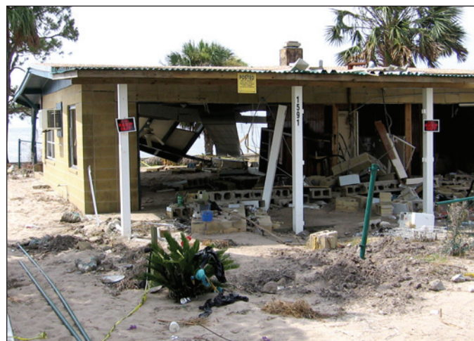
Figure 2. Masonry walls destroyed by 3 feet of stillwater flooding and small waves (Hurricane Dennis).
