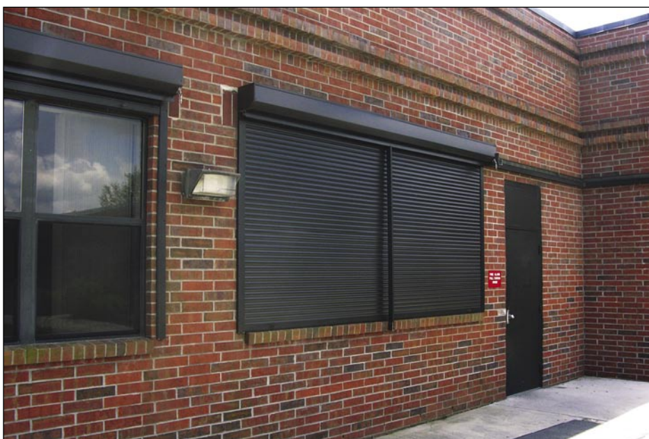
Figure 6-24. Shutters installed at openings at Liberty Elementary School shelter area (Port Charlotte)
