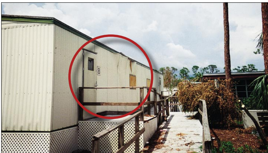
Figure 6-16. Damaged portable classroom unit at an elementary school (Charlotte Harbor)
