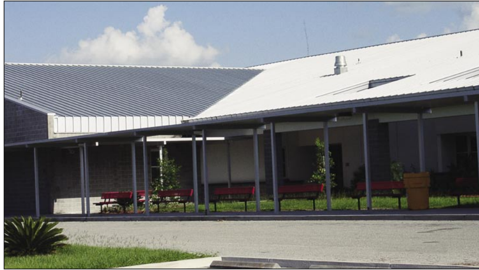
Figure 6-19. Middle school with minimal roof covering damage (Arcadia)
