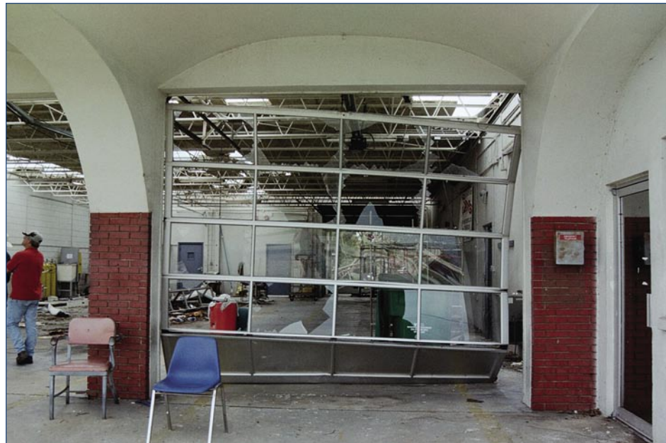
Figure 6-5. View of damaged garage door and interior of Port Charlotte Fire Station No. 1; note missing roof deck panels over apparatus bay.
