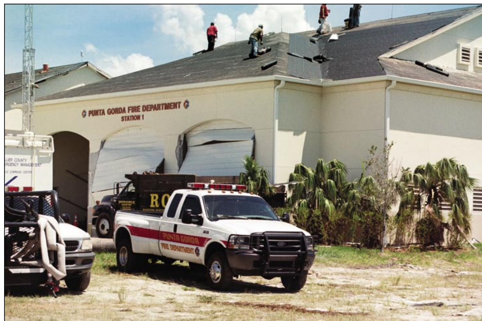
Figure 6-6. Overview of Punta Gorda Fire Station No. 1. The tile roof had been removed and a new roof was being installed. Note the damaged doors.
