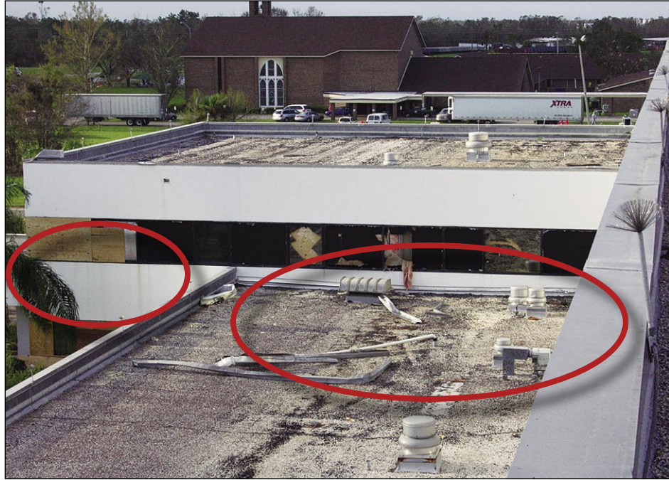
Figure 6-8. Aggregate damaged the windows to ICU rooms at a hospital (Arcadia)
