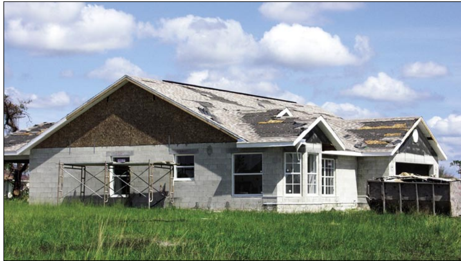
Figure 3-14. Asphalt shingle roof covering damage on a new one-story house. In some areas, the underlayment was also blown away (Deep Creek).
