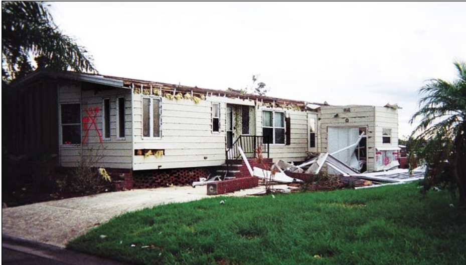
Figure 3-45. Example of typical damage to roof covering, roof sheathing, and exterior siding of a manufactured home as a result of the failure of an attached carport structure (Port Charlotte)
