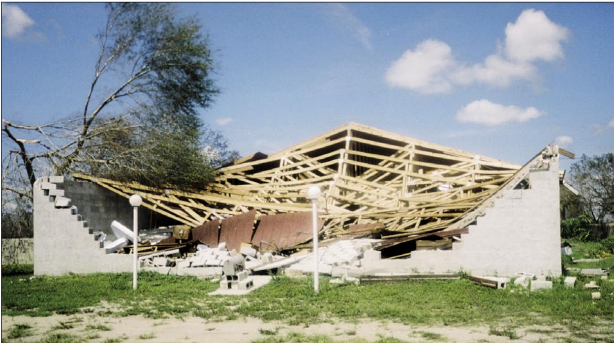
Figure 3-9. Example of wood truss roof failure due to sheathing loss and lack of bracing at gable end on a pre-2001 FBC unreinforced masonry building (north of Arcadia)
