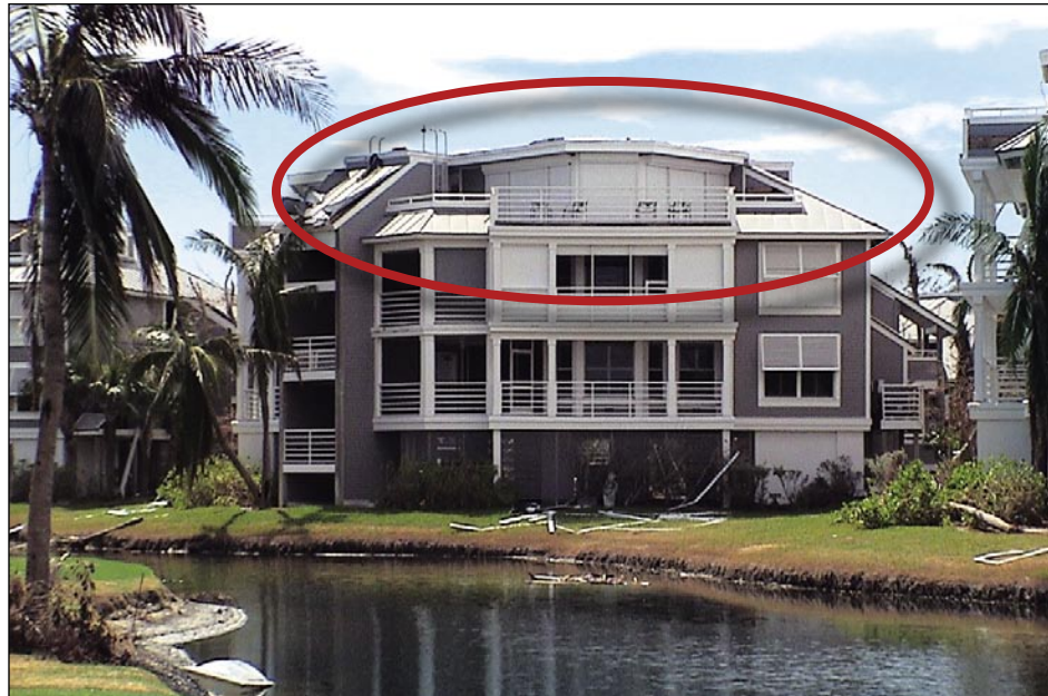
Figure 3-4. Nearby undamaged wood-frame building similar to that shown in Figure 3-3 protected with shutters (Captiva Island)
