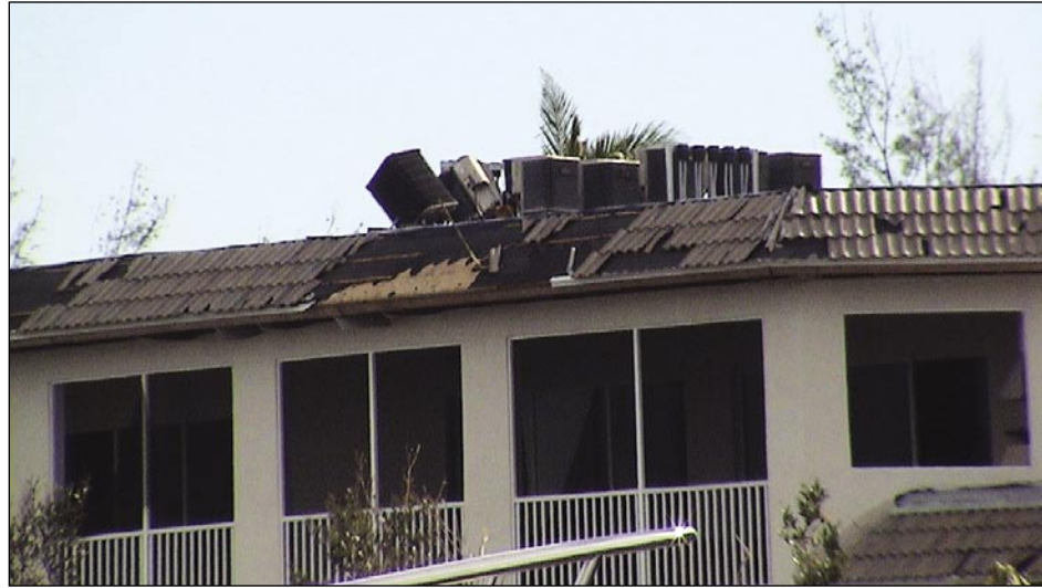
Figure 3-29. Dislocation of rooftop equipment (Pine Island)
