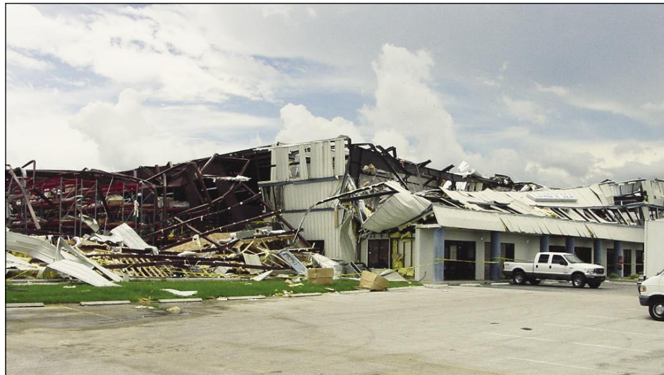
Figure 3-12. Pre-engineered metal building with progressive failure and severe panel loss (Arcadia)
