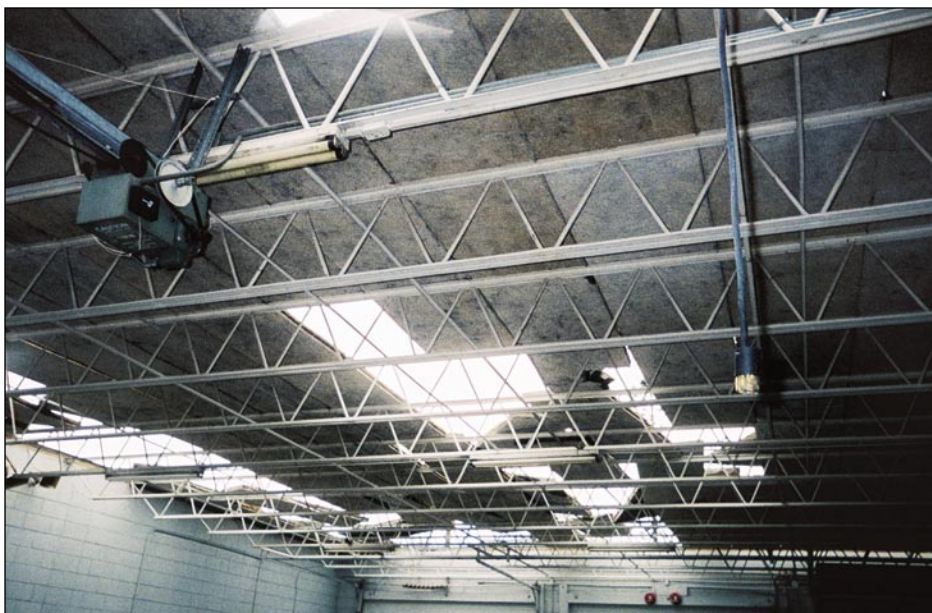
Figure 3-56. Cementitious wood-fiber roof deck panels at this older fire station were not adequately secured to resist uplift (Port Charlotte).
