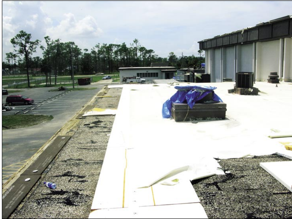
Figure 3-59. Example of roof covering damage at a school. This was a mechanically attached single-ply membrane over a previous aggregate surfaced built-up roof (Port Charlotte).
