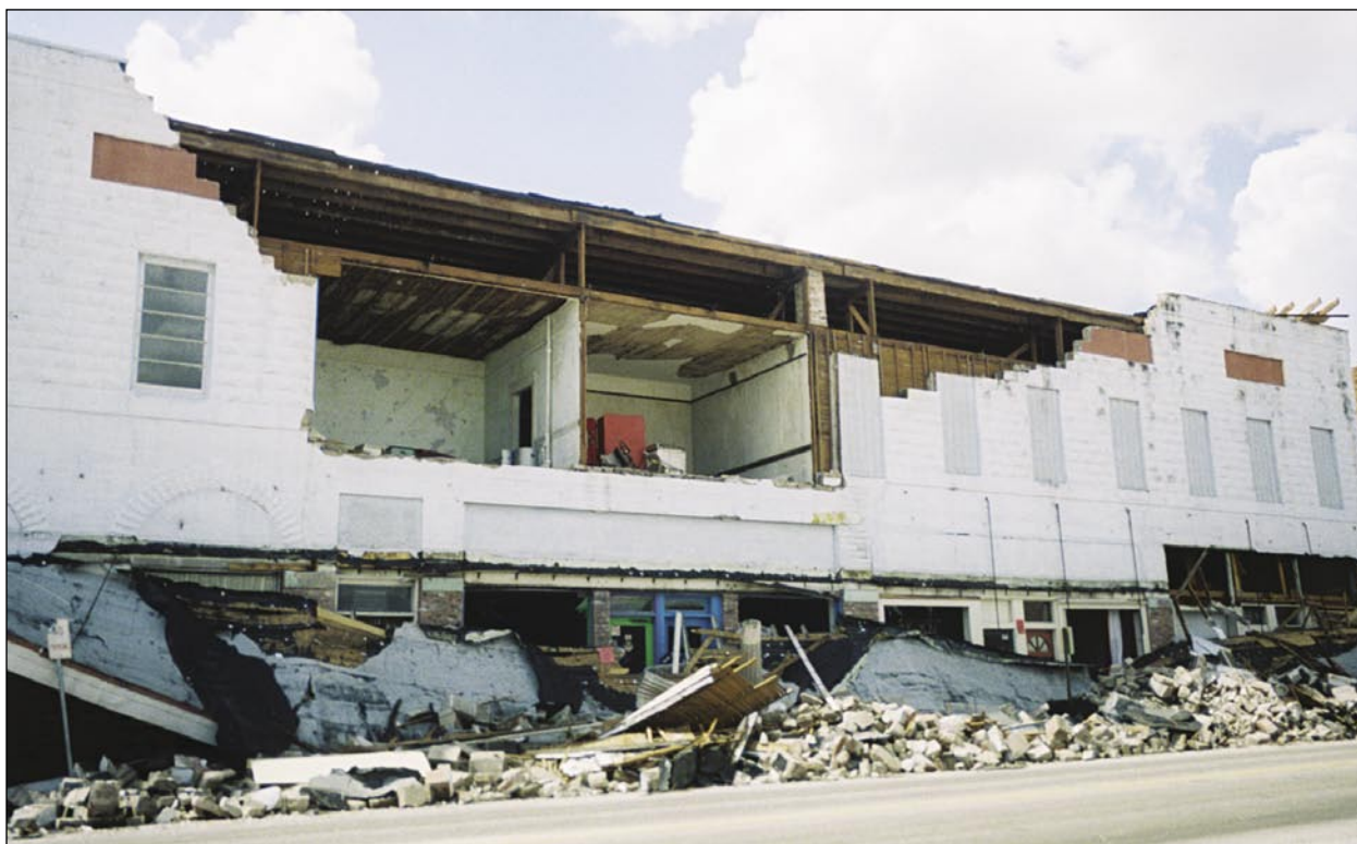
Figure 3-25. Example of unreinforced masonry wall and parapet collapse due to breaching of roof (on opposite side of building) (Wauchula)
