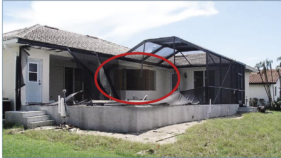
Figure 3-47. Example of damage to pool screen enclosure. Note broken window in center of photo from debris (Punta Gorda Isles).
