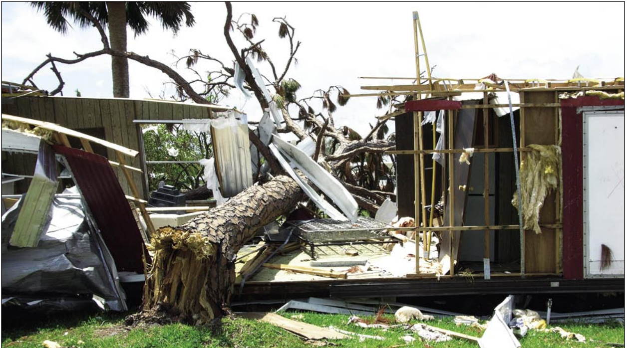
Figure 3-43. Damage to manufactured home from tree impact (Pine Island)
