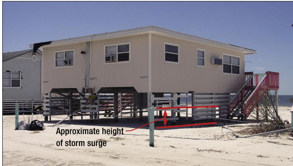
Figure 3-50. Oceanfront house constructed on piles sustained only minor damage as a result of storm surge (Fort Myers Beach)
