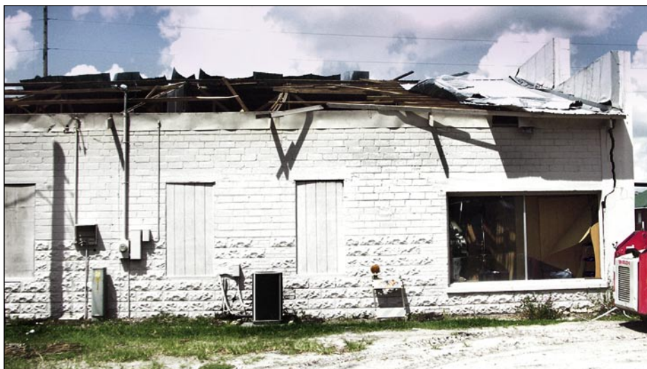
Figure 3-10. Roof sheathing and partial failure of wood roof structure on a masonry building. Note damage to inadequately reinforced masonry parapet at gable end wall (Wauchula).
