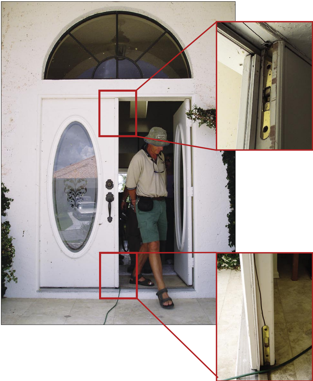
Figure 3-20. Double-entry door that failed under wind pressure. Upper inset shows close-up of crack in door frame at top latch. Lower inset shows crack in door emanating from bottom latch (Punta Gorda).
