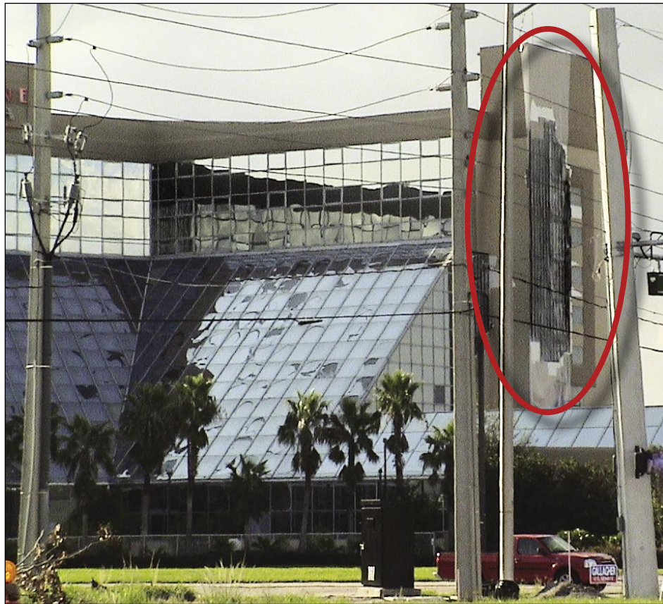
Figure 3-33. Damage to glass atrium of high-rise hotel. Note the loss of EIFS, which was the cause of the glass breakage (Orlando).
