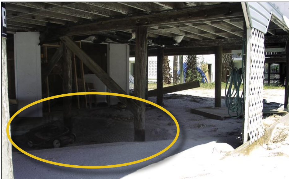
Figure 3-49. Minor scour around pile (Fort Myers Beach)
