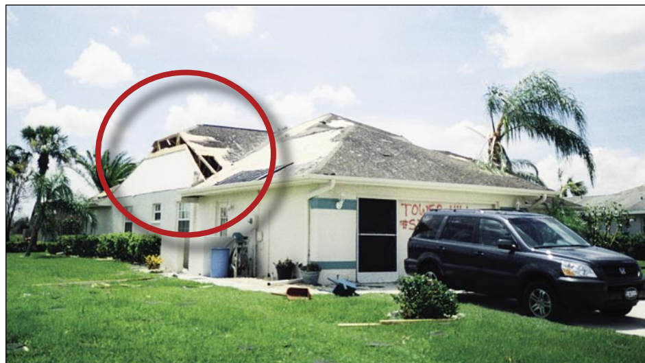
Figure 3-19 Partial gable end wall failure with loss of roof shingles (Deep Creek)
