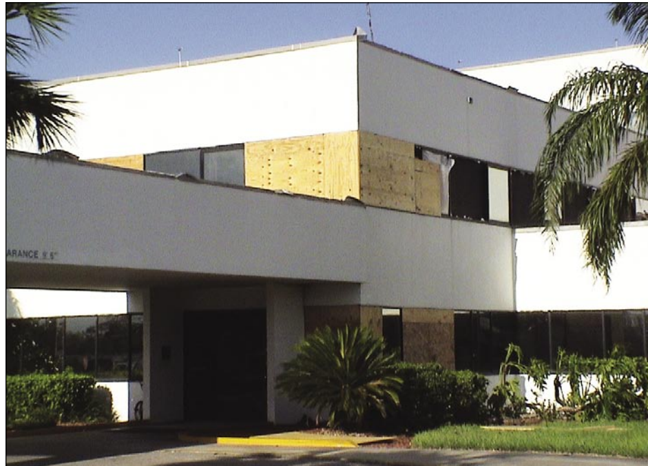
Figure 3-41. Aggregate from the built-up roofs broke windows at the intensive care unit of a hospital where 3-second peak gust wind speeds were estimated between 110 and 120 mph (Arcadia).
