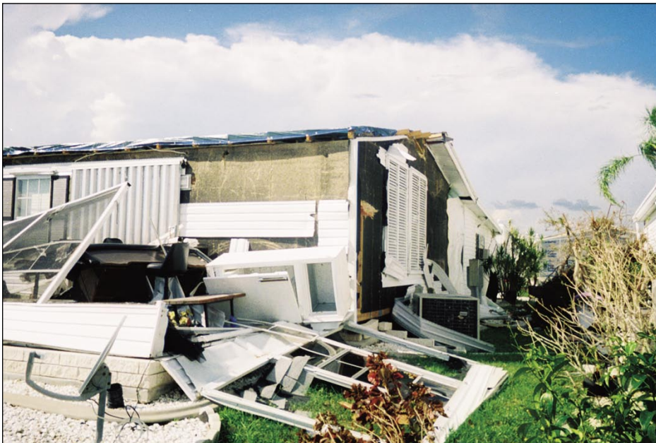
Figure 3-46. Example of damage to manufactured home roof covering, roof deck, and siding due to failure of screen enclosure attached to home (Port Charlotte)
