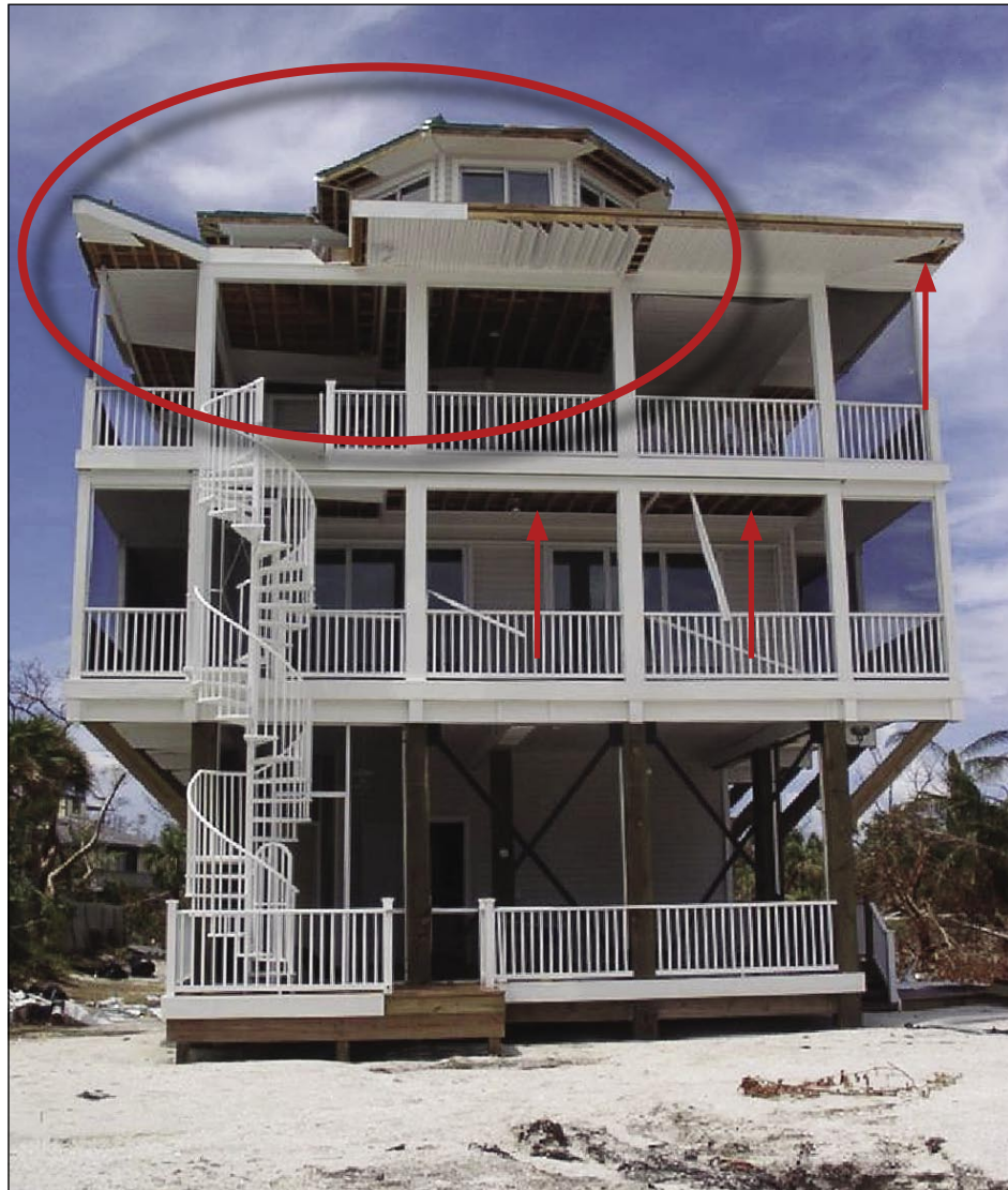
Figure 3-21. Typical elevated wood- frame house with extensive soffit damage (North Captiva Island)
