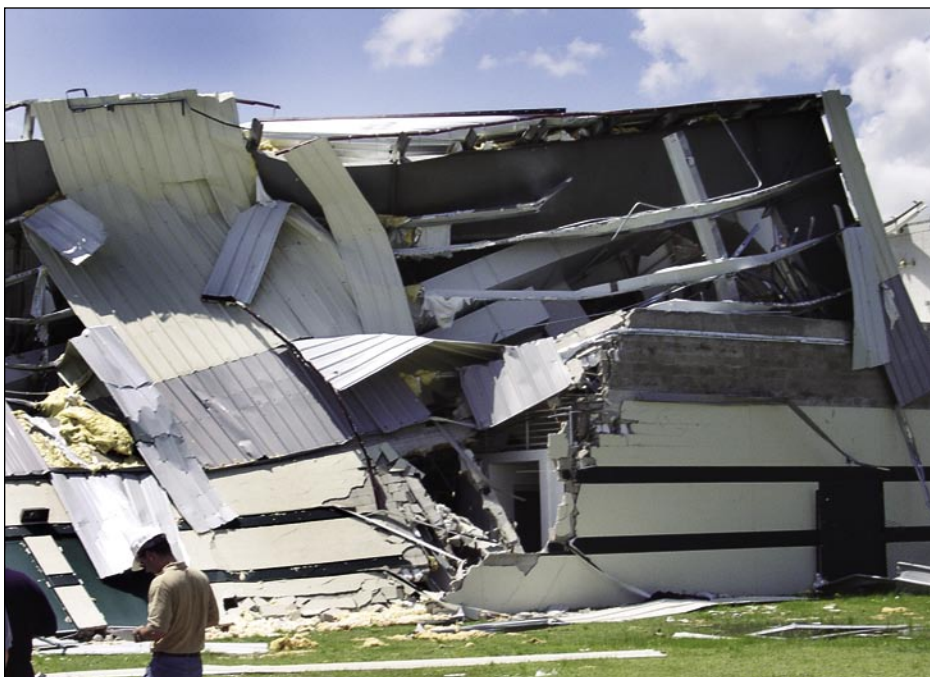
Figure 3-58. End wall damage to long span, pre-engineered metal building designed for use as a storm shelter (Turner Agri-Civic Center, Arcadia – see Section 6.5.1.1)
