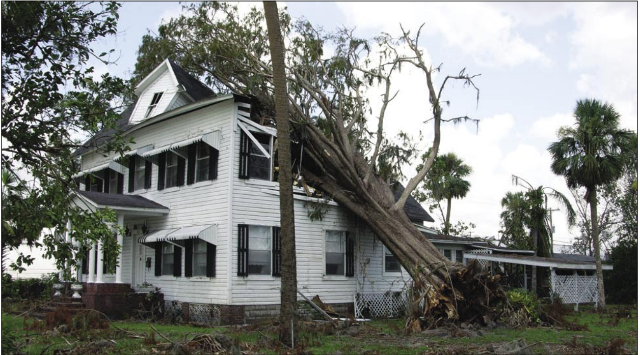
Figure 3-42. Damage to three-story home from tree impact (Wauchula)
