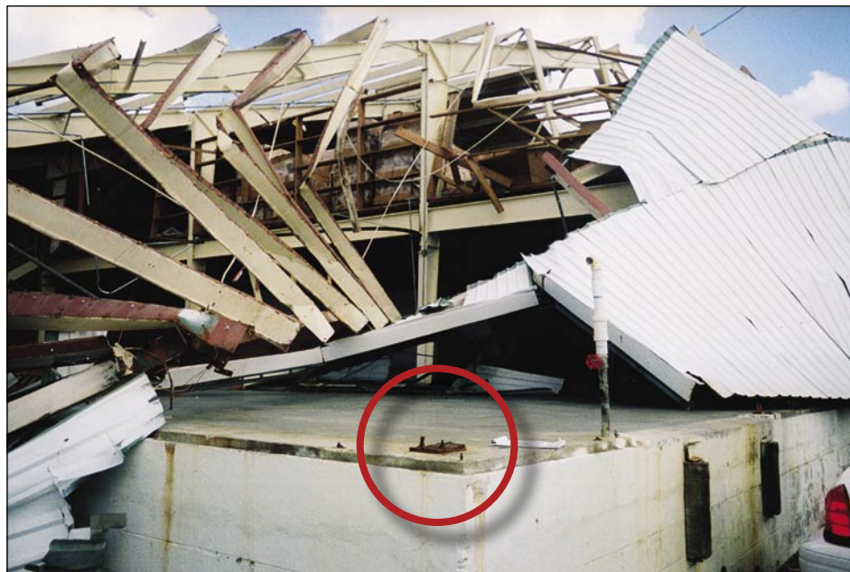
Figure 3-13. Roof framing failure and gable end wall collapse due to insufficient supports of pre-engineered metal building. Note corroded base plate with failed bolts for gable end wall column (Wauchula).
