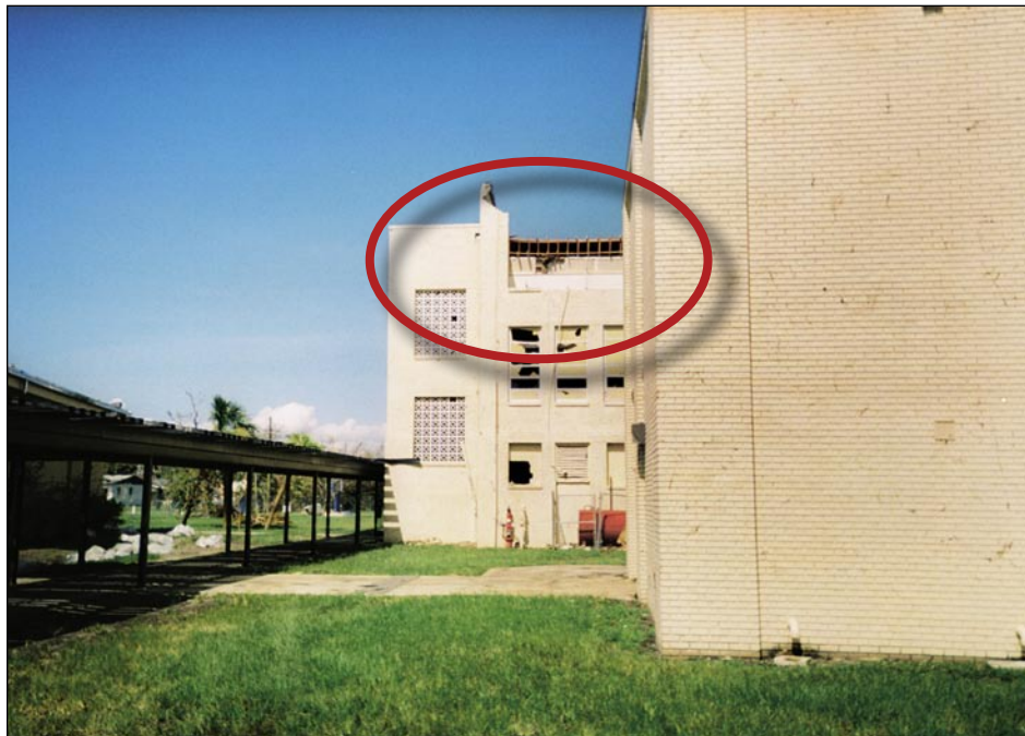
Figure 3-60. Example of URM parapet wall collapse and broken windows at an older school (Punta Gorda)
