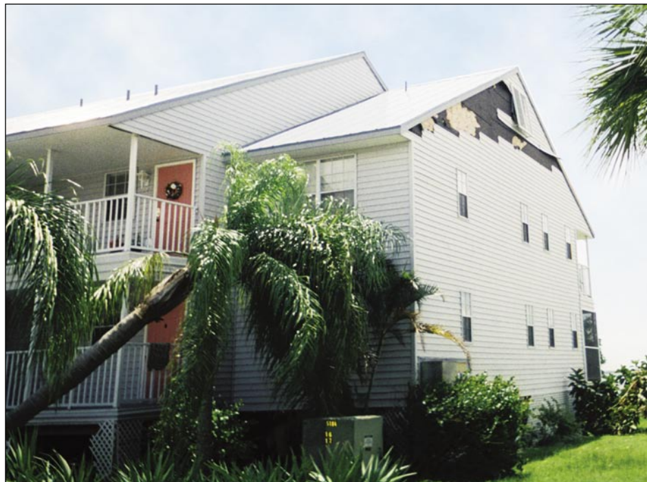
Figure 3-24. Vinyl siding wall covering on multi-family building with damage to gable end wall sheathing (Port Charlotte)
