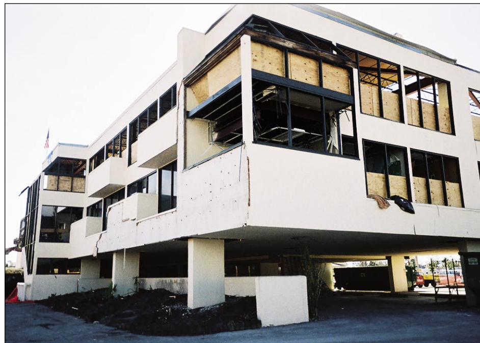
Figure 3-27. Structural steel frame building showing loss of roof decking and damage to EIFS wall coverings (Punta Gorda)
