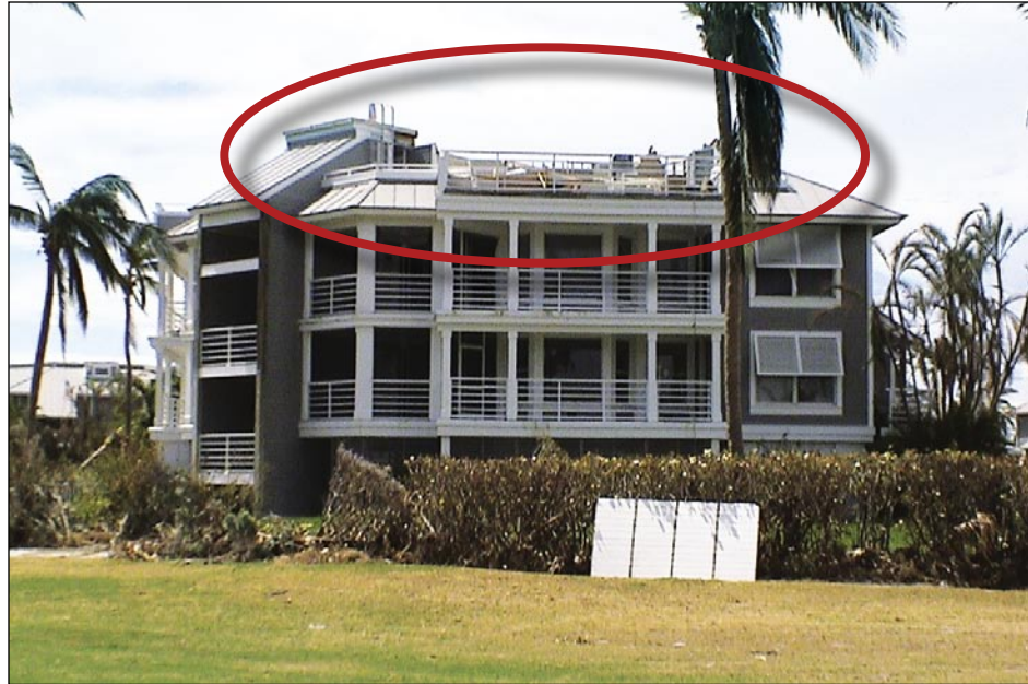
Figure 3-3. Loss of roof structure in a wood-frame building likely due to internal pressurization resulting from unprotected windows and doors (Captiva Island)
