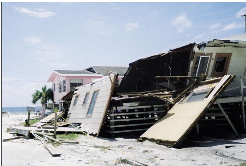
Figure 3-5. Wall failure on older multi-family wood-frame building due to lack of continuous load path. Internal pressurization may have also contributed to this failure (Fort Myers Beach).
