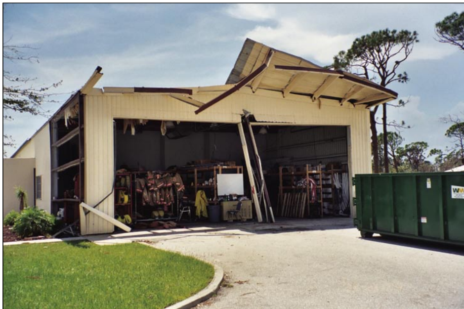
Figure 4-19. Main column at Fire Station No. 8 collapsed due to corrosion and metal siding failed (Port Charlotte)
