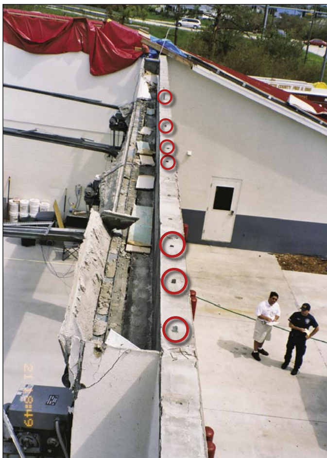
Figure 4-15. Roof truss hurricane anchor straps failed at the tie-beam at Fire Station No. 12 (Port Charlotte)
