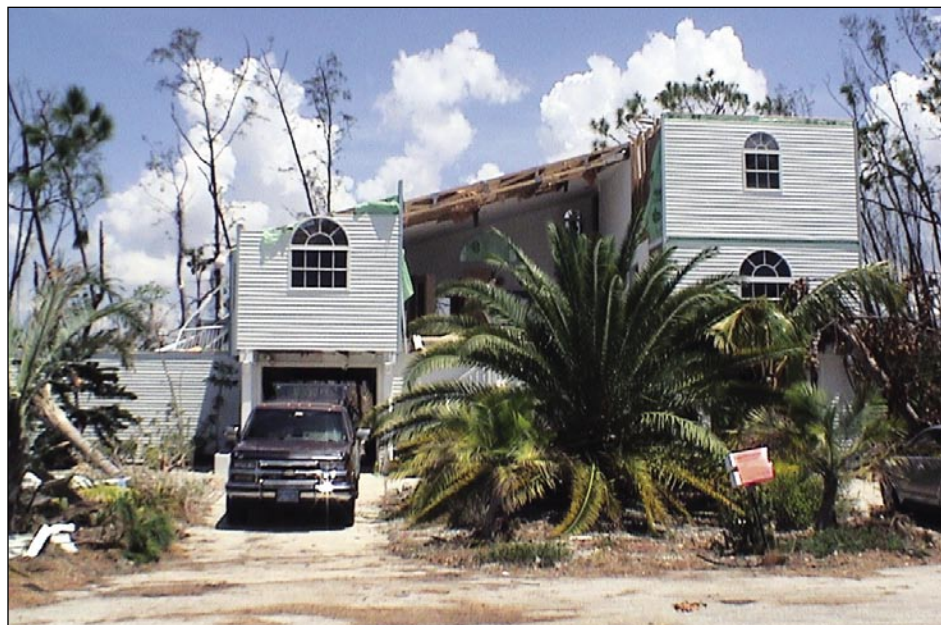
Figure 4-5. Failure of the roof over a cathedral ceiling from pressurization of the house when the window failed on the windward face (Pine Island)
