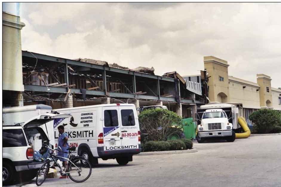
Figure 4-16. Older steel-frame structure performed well in spite of major damage to the roof decking and the exterior walls (Wauchula)
