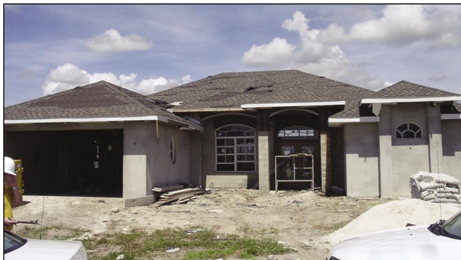
Figure 4-11. New concrete masonry residence built to 2001 FBC standards performed well structurally, although it did experience some asphalt shingle damage (Port Charlotte).
