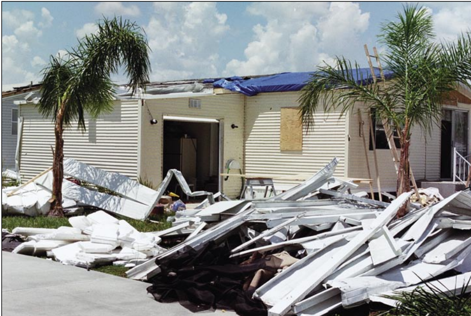
Figure 4-22. Damaged garage (Zolfo Springs)
