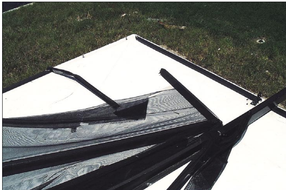
Figure 4-26. Consequence of corner post not directly tied down to the slab (Punta Gorda Isles)
