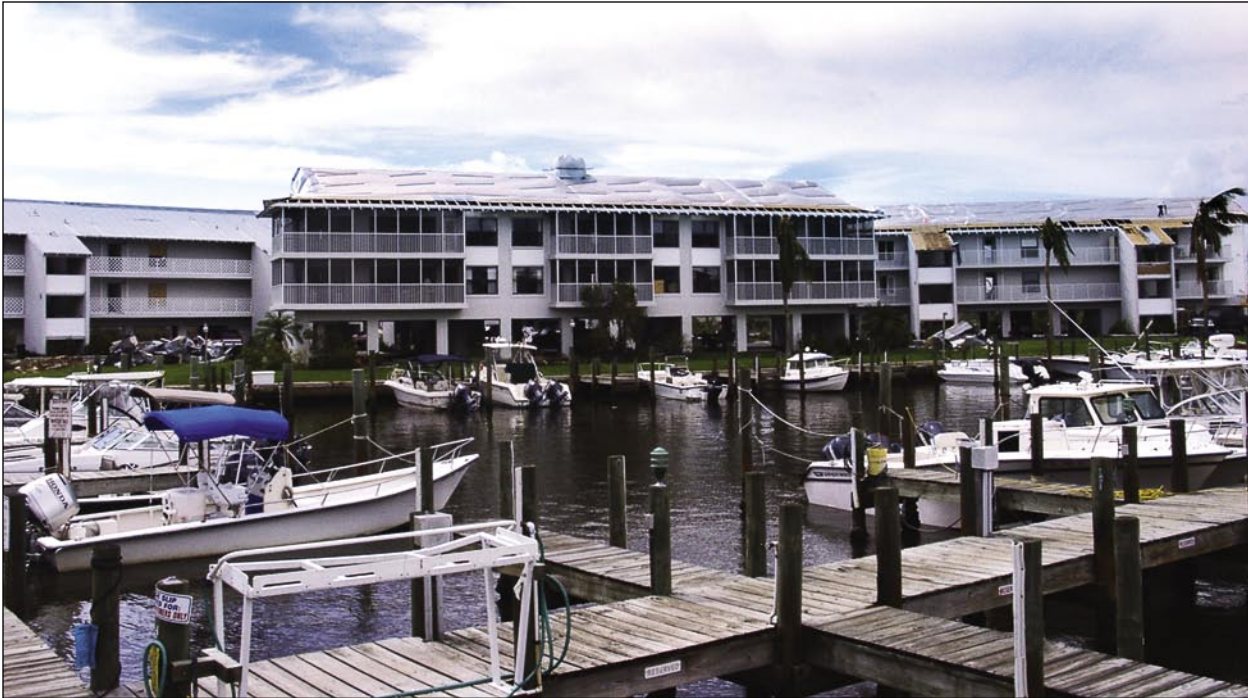
Figure 4-7. Multi-family residential building that performed well structurally, although it had severe roof covering and some sheathing failure at the overhangs, allowing water intrusion (Pine Island)
