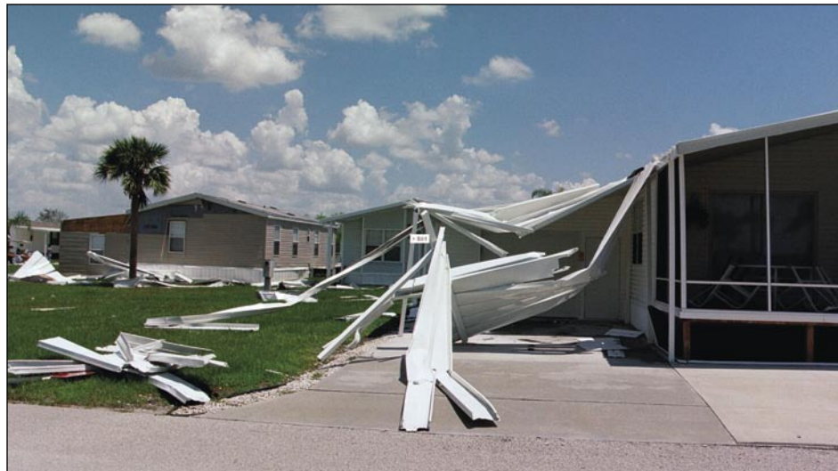
Figure 4-21. Damaged carport (Zolfo Springs)
