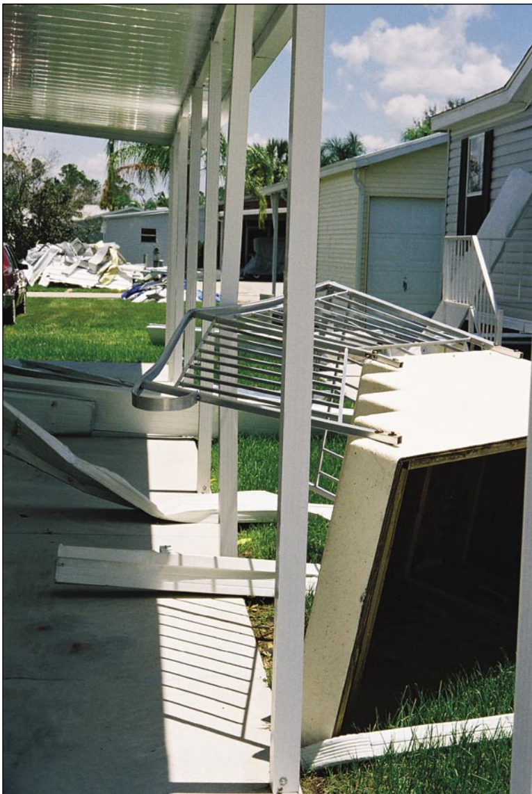
Figure 4-24. Stairway blown into a post of an aluminum carport accessory structure (Zolfo Springs)
