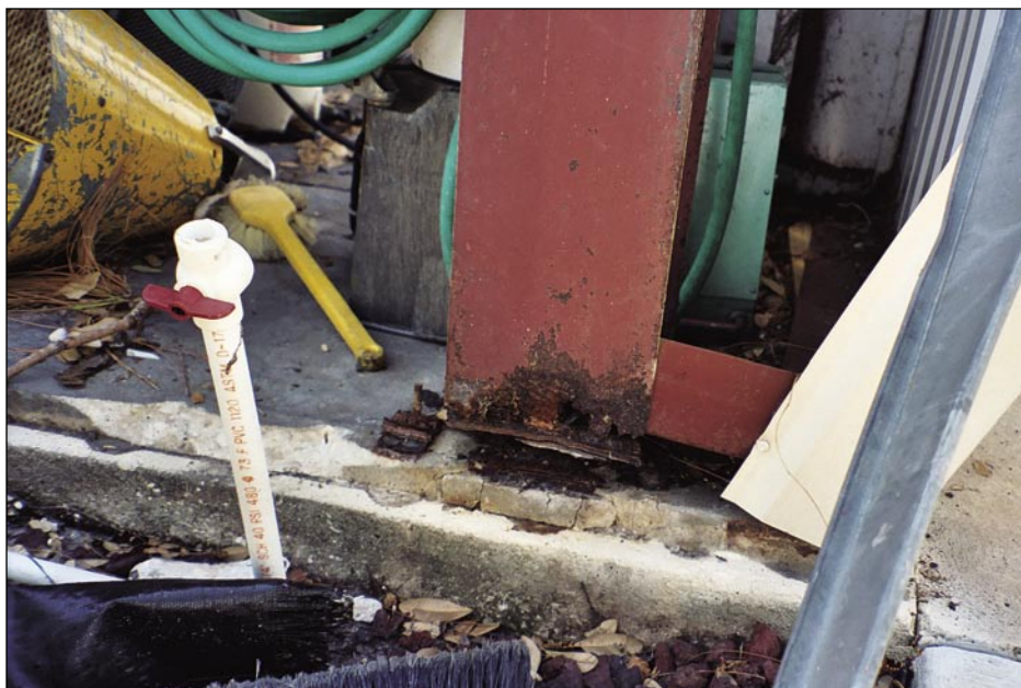
Figure 4-20. Significant amount of corrosion at Fire Station No. 8, which contributed to failure shown in Figure 4-19
