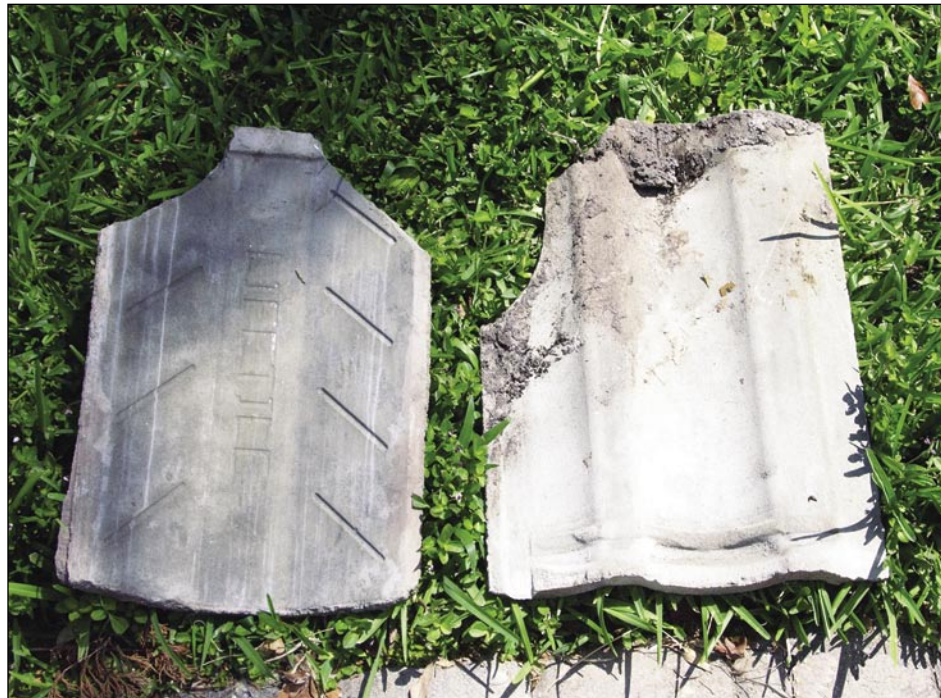
Figure 5-48. Tiles that flew through windows of an occupied residence (Deep Creek)
