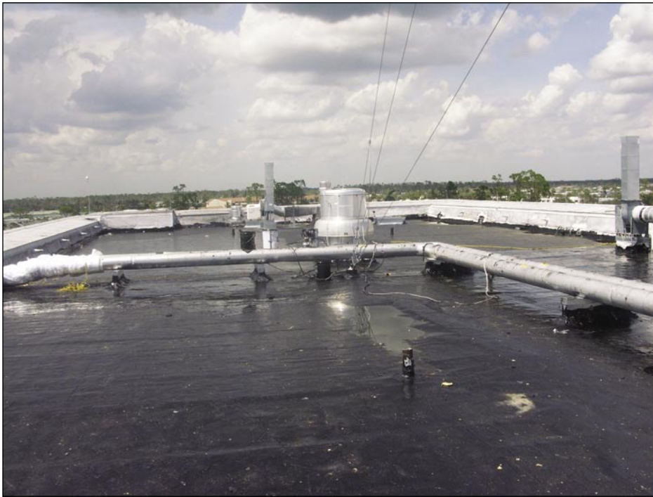
Figure 5-64. View of a portion of the fourth floor roof of a hospital after installation of an emergency roof (the black area). The deck was concrete (Port Charlotte).
