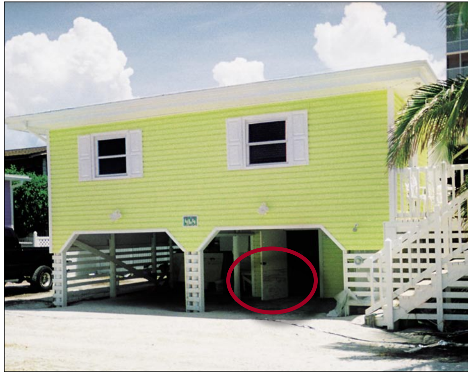
Figure 7-2. Older residence atop pile foundation that allowed floodwaters to pass safely underneath, resulting in only minor damage to enclosures and access stairways (Fort Myers Beach)
