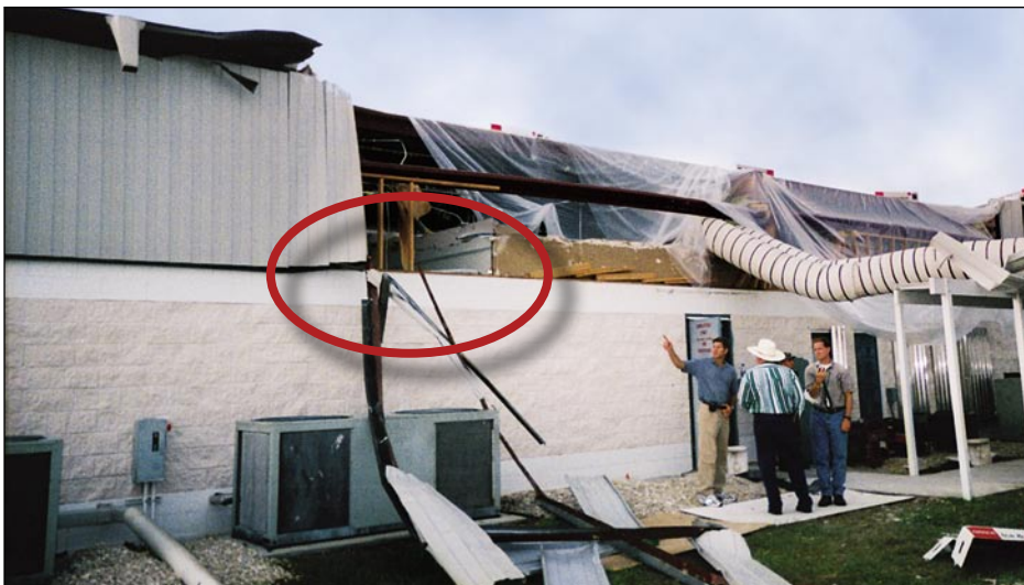
Figure 6-1. Exterior wall and roof damage at Charlotte County EOC
