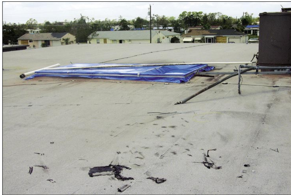
Figure 5-77. A large HVAC unit blew off this curb. Note the loose LPS conductors (this side of the curb). This school had significant damage to several pieces of rooftop equipment (Port Charlotte).
