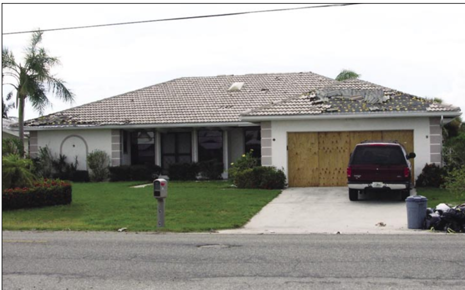
Figure 5-41. In addition to field tile blow-off, most of the hip tiles and several ridge tiles were also blown off this house (Punta Gorda Isles).
