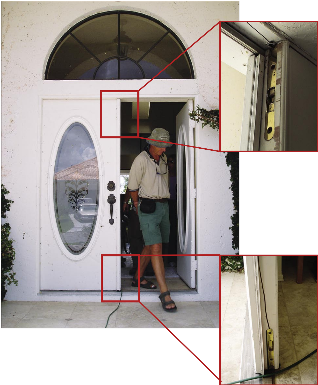
Figure 3-20. Double-entry door that failed under wind pressure. Upper inset shows close-up of crack in door frame at top latch. Lower inset shows crack in door emanating from bottom latch (Punta Gorda).
