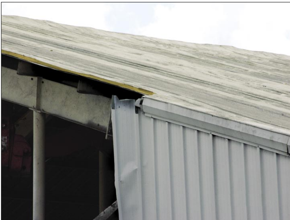
Figure 5-58. The metal wall panels and metal edge flashing on this building blew away, but the exposed fastener R-panels with an SPF covering did not progressively fail (Wauchula).
