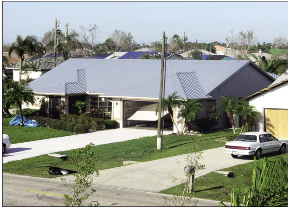
Figure 5-5. Garage door at the home in the center buckled and the rollers pulled out from their tracks; garage door at the home on the right also failed (Deep Creek).
