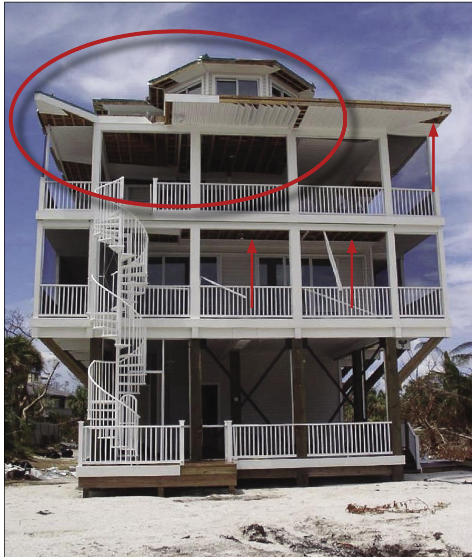
Figure 3-21. Typical elevated wood- frame house with extensive soffit damage (North Captiva Island)
