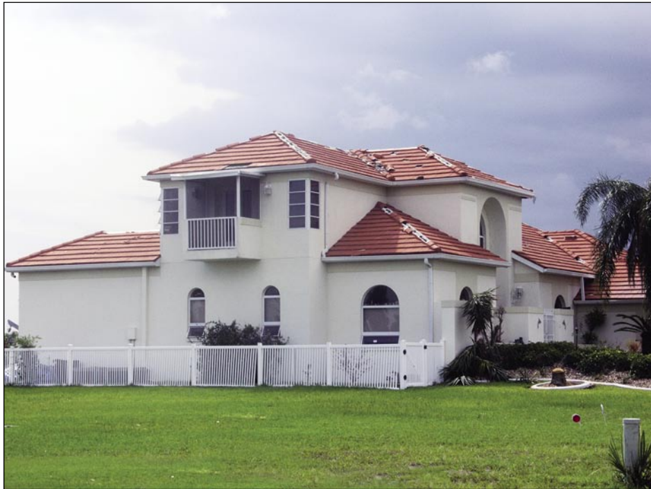
Figure 5-32. Most of the mortar-set hip and ridge tiles blew off this house (Port Charlotte).
