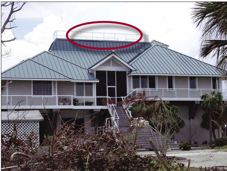
Figure 7-1. Residence constructed to the design requirements of the 2001 FBC performed well and only experienced some light trim damage (shown in the center of the photo) (North Captiva Island).
