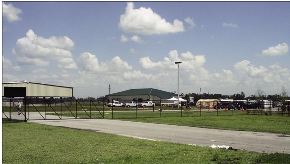
Figure 6-20. Pre-engineered metal buildings with minimal damage located near the Turner Agri-Civic Center (Arcadia)
