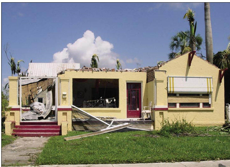
Figure 3-2. Failure of roof structure from pressurization of a pre-2001 FBC house when the window failed on windward face (Punta Gorda)
