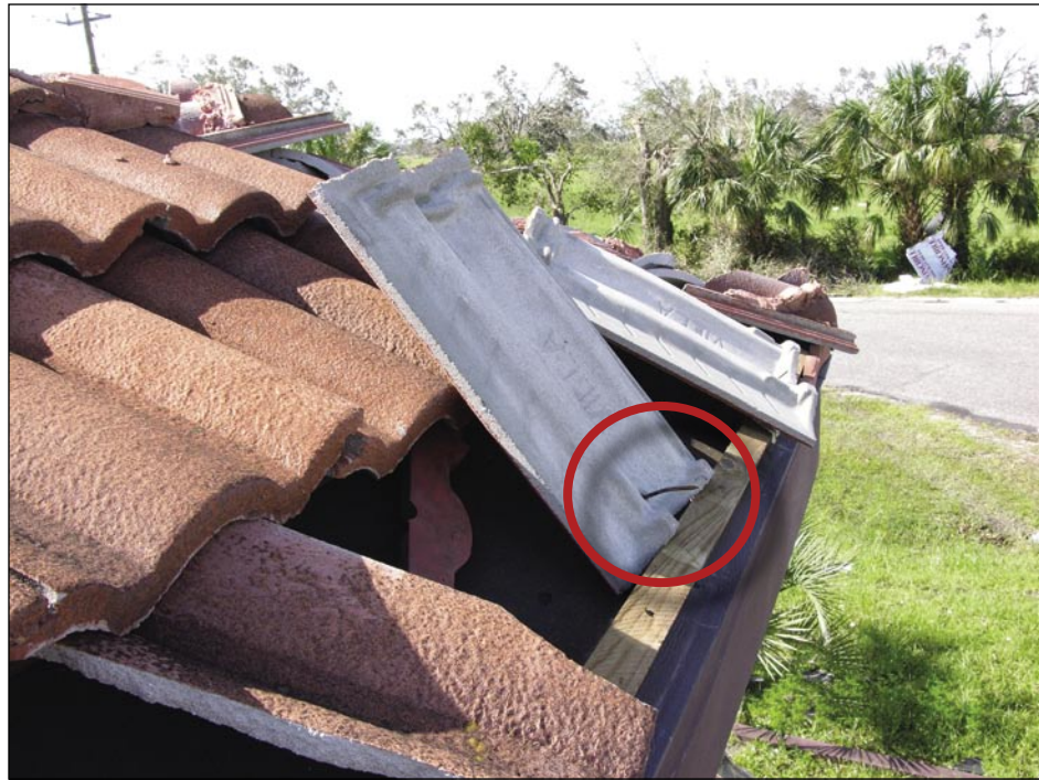
Figure 5-34. Each tile on this building was attached to battens with a single 3 1 / 8 -inch long smooth shank nail (Arcadia)
