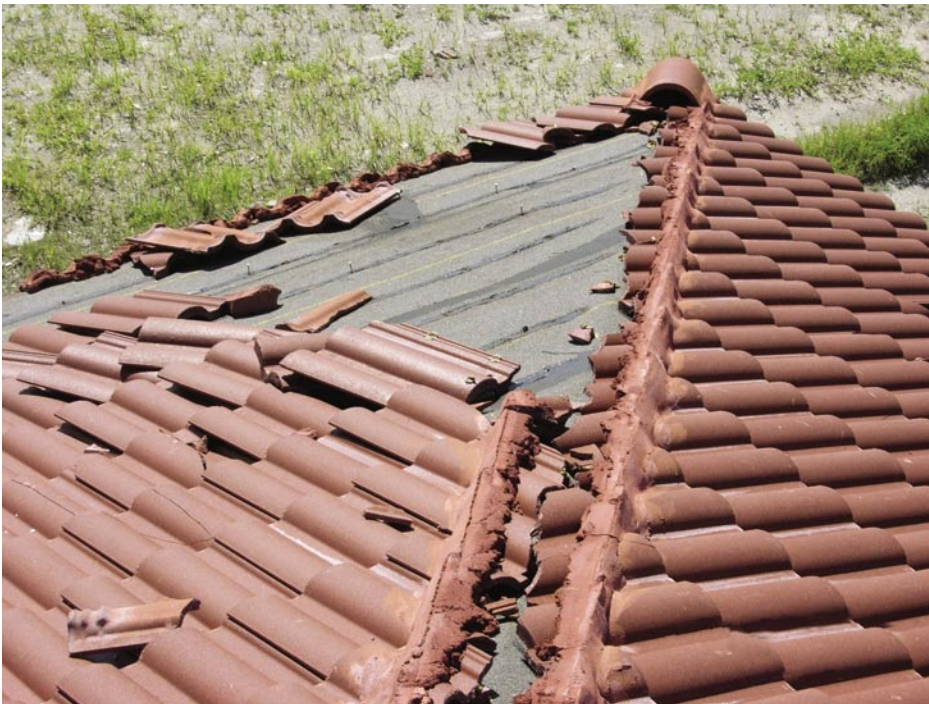
Figure 5-36. Loss of mortar-set hip tiles and several of the field tiles. Some of the screws remained in the deck, while others had been pulled out (Deep Creek).
