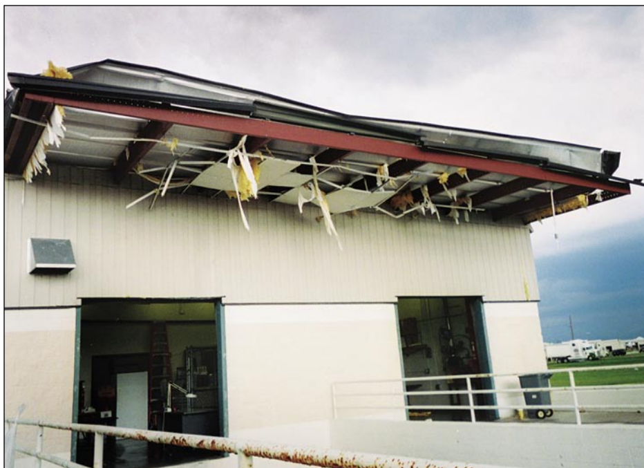
Figure 6-3. Failure of roof and soffit panels at rear awning (Charlotte County EOC)
