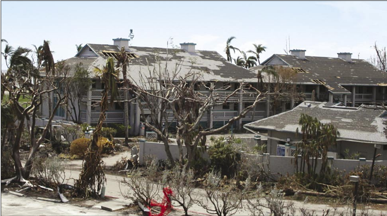
Figure 3-23. Roof covering loss. Note dark areas on roof are exposed underlayment (Captiva Island).
