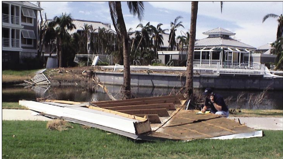
Figure 3-38. Large section of roof structure transported over 200 yards from its source (Captiva Island)
