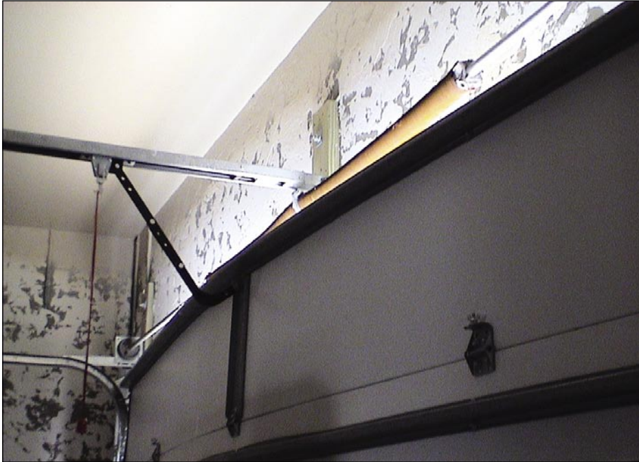
Figure 5-6. Garage door failed because the removable stiffener bar was not in place at the time of the hurricane (Punta Gorda Isles).
