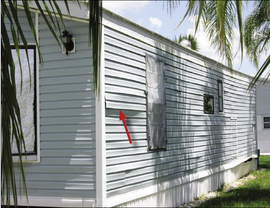
Figure 5-65. The vinyl siding panel with the red arrow is unlatched. The panel above and several others are also unlatched (Zolfo Springs).
