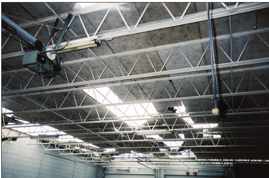
Figure 3-56. Cementitious wood-fiber roof deck panels at this older fire station were not adequately secured to resist uplift (Port Charlotte).
