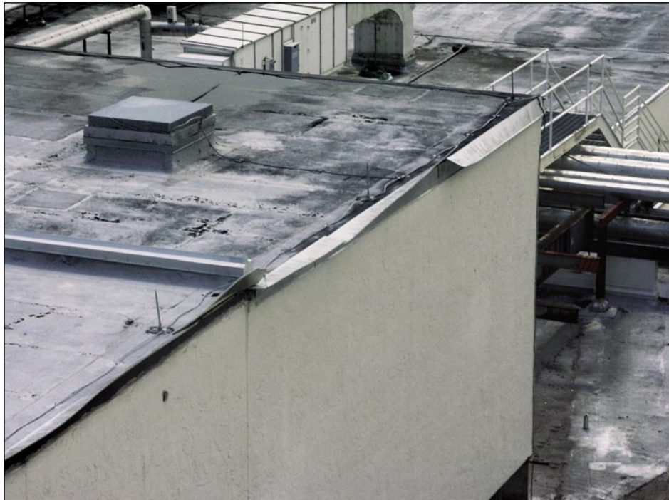
Figure 5-62. The edge flashing at this mineral surface cap sheet roof lifted (Port Charlotte).
