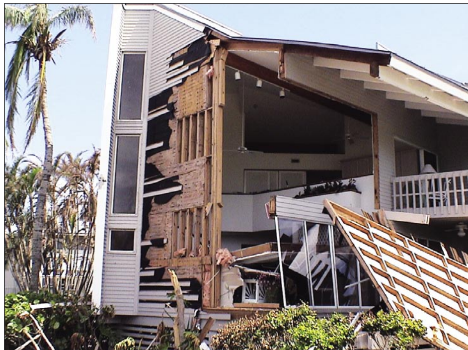
Figure 4-8. Wall failure on older (1980s vintage) multi-family wood-frame building due to lack of load path. Internal pressurization may have also contributed to this failure (Captiva Island).
