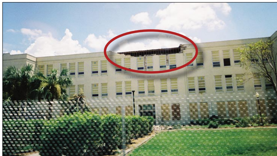
Figure 6-11. URM parapet damage to front façade of a high school (Punta Gorda)
