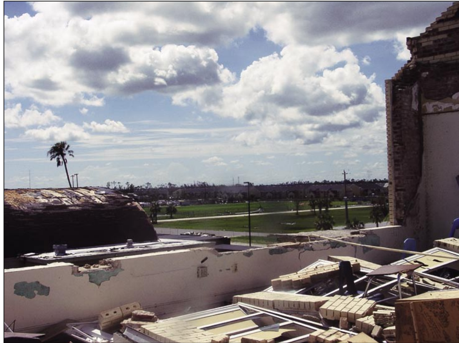
Figure 4-13. Unreinforced brick wall failure of a building built over 50 years ago (photo taken from the inside of a classroom, looking out) (Punta Gorda)
