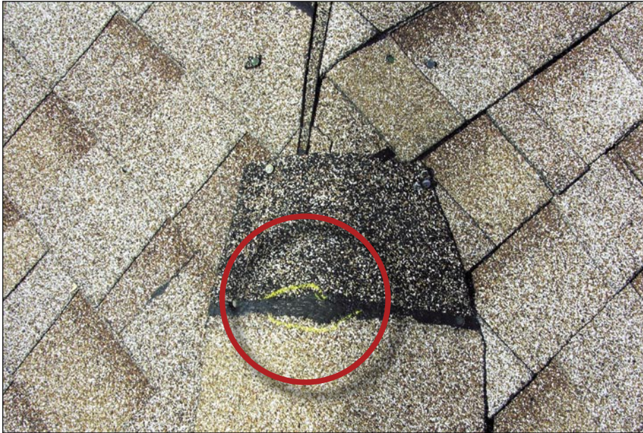
Figure 5-26. Only the portion of the self-seal adhesive that is indicated in yellow had bonded (within the red circle). No bonding occurred on the right side of the hip line (Deep Creek).
