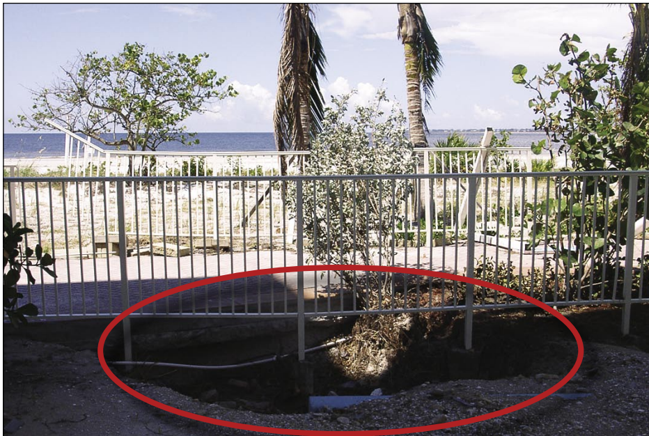
Figure 3-48. Minor scour of parking lot from overwash of storm surge (Fort Myers Beach)
