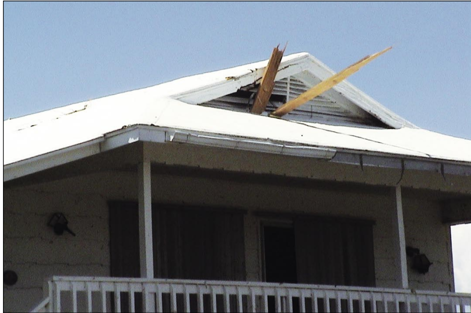
Figure 3-37. Impact of structural wood members in the gable end from a neighboring house (Pine Island)
