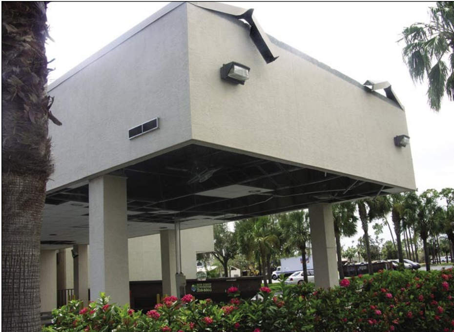
Figure 5-70. Loss of soffit at a bank drive-through. Note the coping damage (Port Charlotte).
