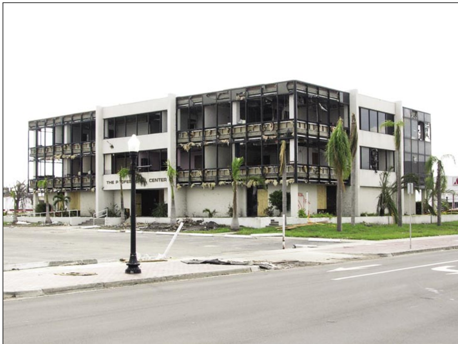
Figure 5-18. All of the glazing, including glass spandrel panels, was broken on the long side of the building (Punta Gorda).
