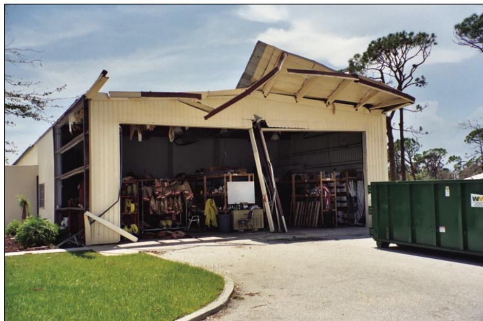
Figure 4-19. Main column at Fire Station No. 8 collapsed due to corrosion and metal siding failed (Port Charlotte)
