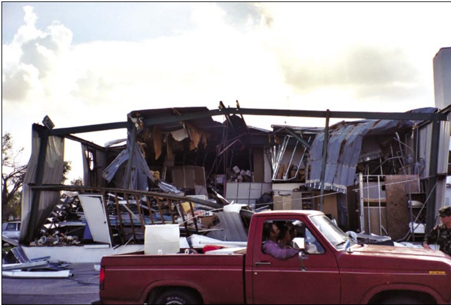
Figure 4-17. Completely destroyed pre-engineered metal building (Arcadia)
