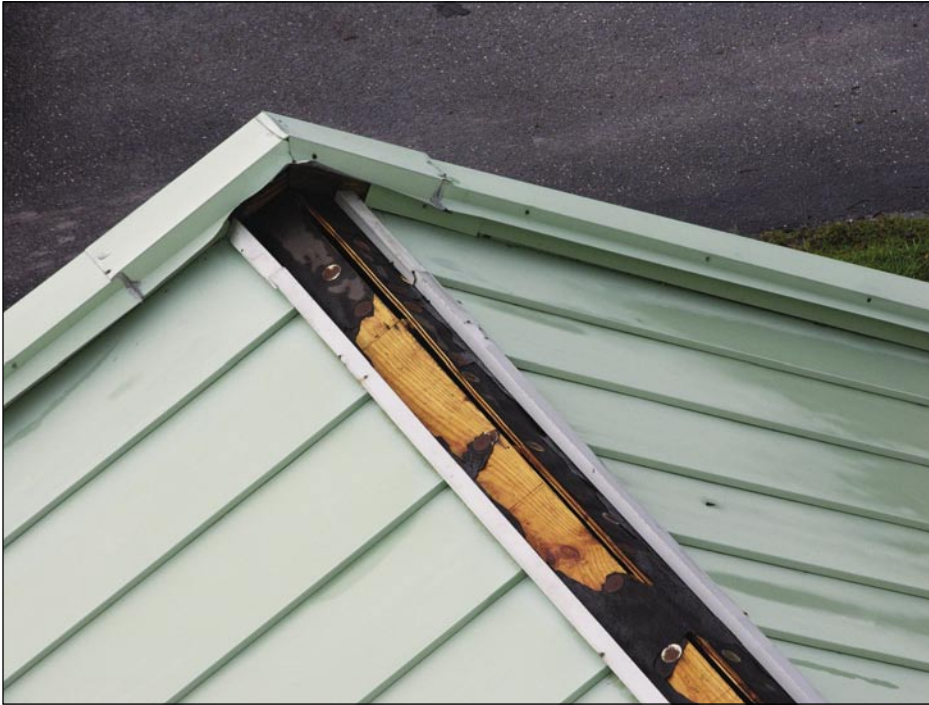
Figure 5-54. View of the canopy ridge at the building shown in Figure 5-52. The ridge flashing fasteners were placed too far apart. A significant amount of water leakage can occur when ridge flashings are blown away (Port Charlotte).
