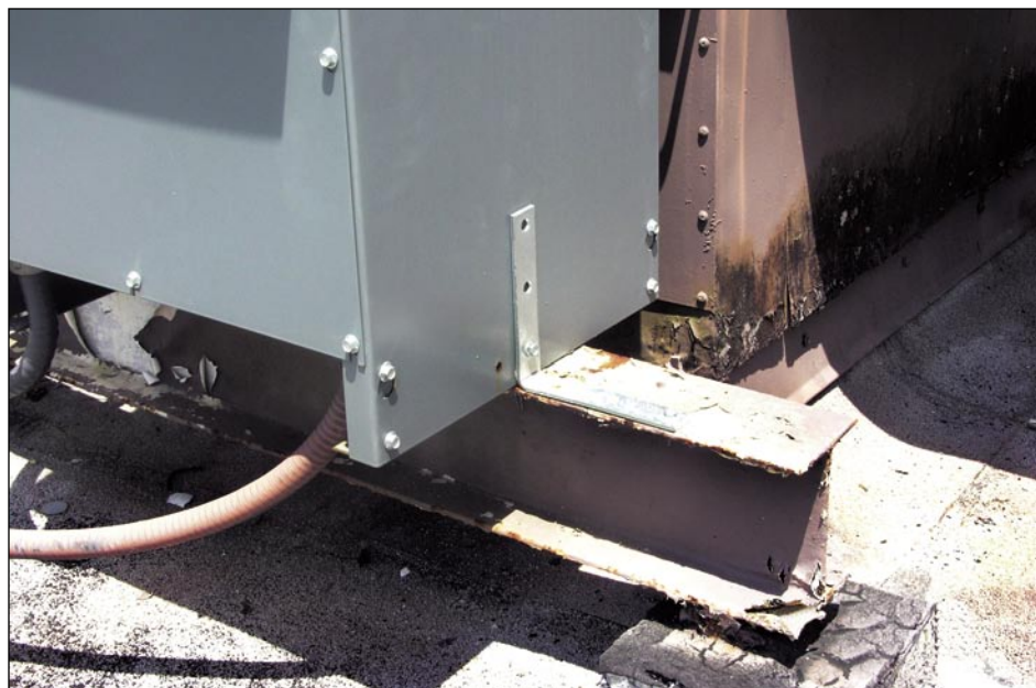
Figure 5-78. A thick angle bracket was used to anchor this unit. Although two screws attached the angle to the support beam, only one screw was used at the unit (Port Charlotte).
