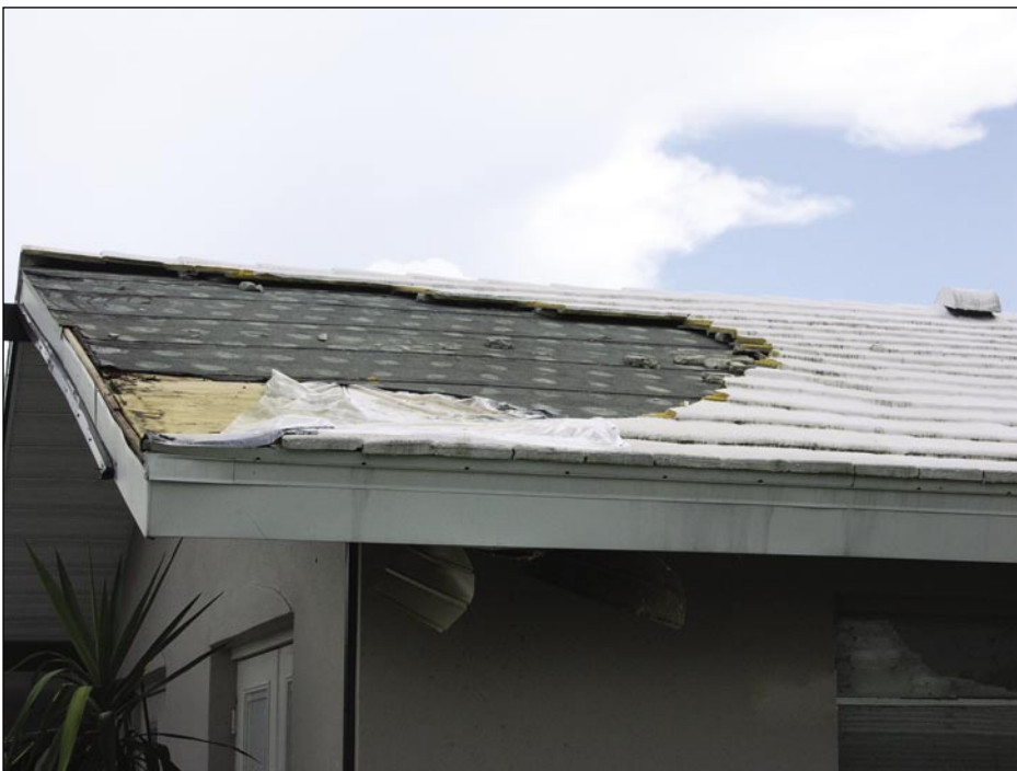
Figure 5-47. The other side of the roof shown in Figure 5-46 with a portion of the underlayment and several tiles blown off (Punta Gorda Isles)
