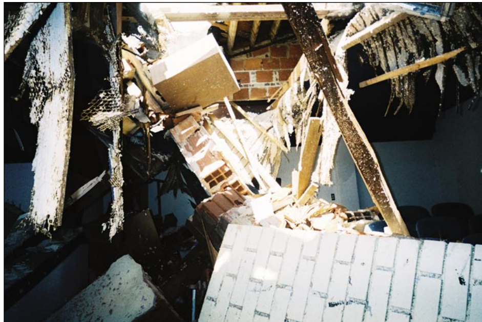
Figure 6-10. Hollow clay tile wall/ parapet damage to roof of a high school auditorium (Punta Gorda)
