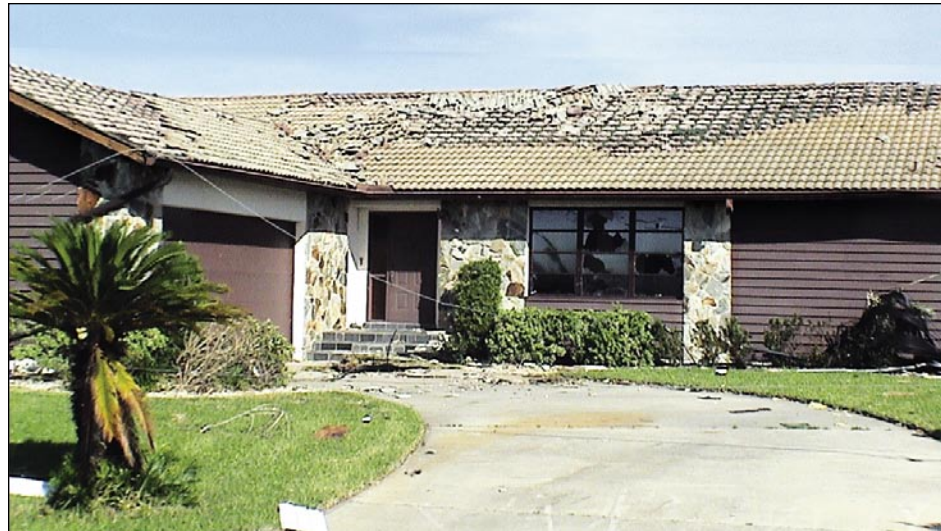
Figure 3-31. Extensive damage to mortar-set tile roof on this pre-2001 FBC home. Note broken windows to the right of the front door (Punta Gorda).
