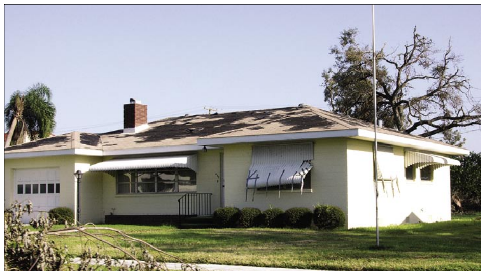
Figure 5-25. Residence with a significant number of asphalt shingles lost. The metal window shutters shown were not designed for windborne debris (Fort Meade).
