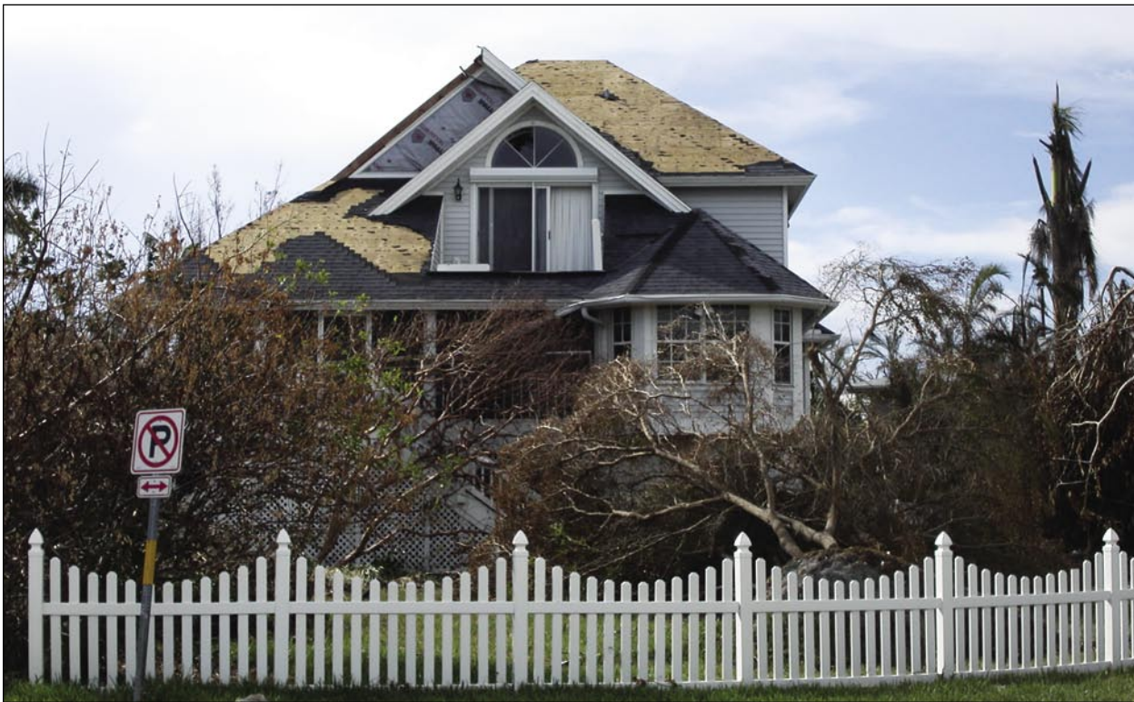
Figure 3-15. Typical asphalt shingle roof covering loss on elevated, two-story house (Captiva Island)
