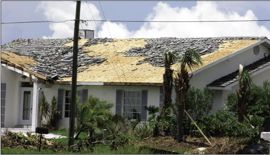
Figure 5-30. A large area of underlayment at this mortar-set flat tile roof blew away. The loss of tile underlayment was atypical (Punta Gorda).
