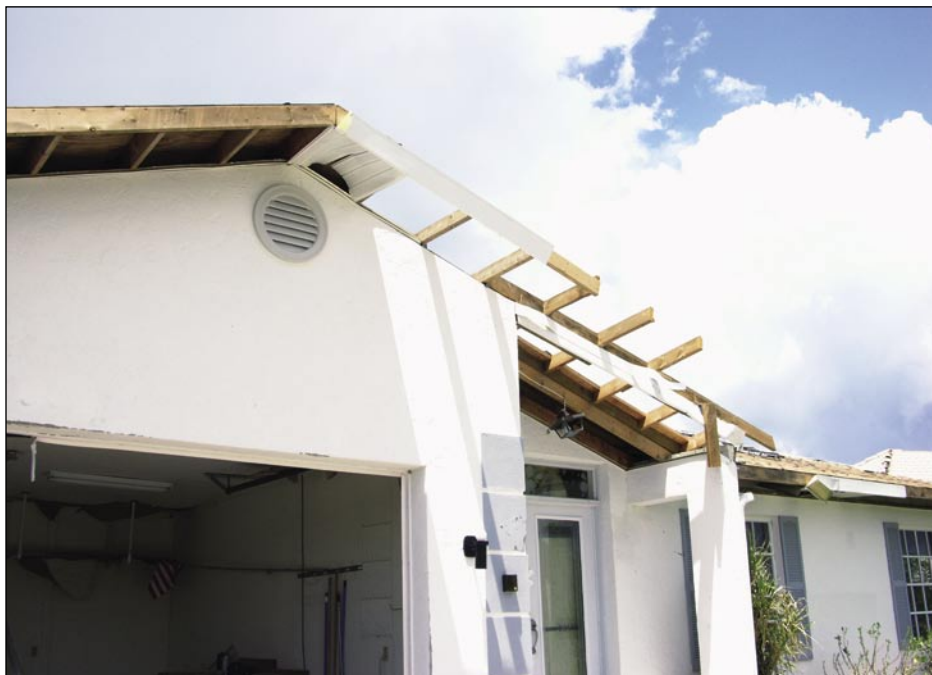
Figure 4-6. Roof decking failed due to uplift (Deep Creek)
