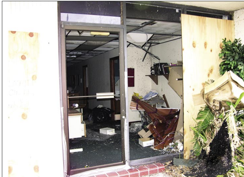
Figure 5-2. Tempered glass in office building entry door and side windows broken by missiles (Punta Gorda)
