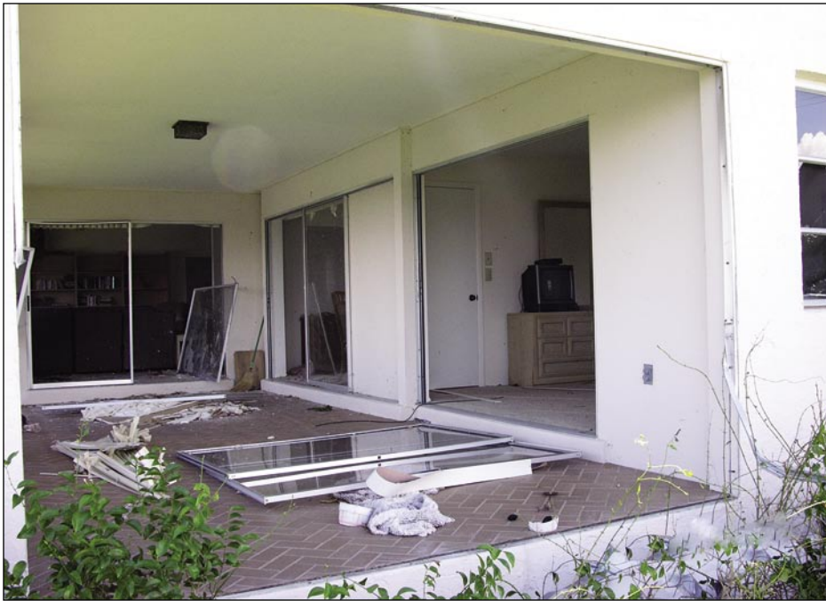
Figure 5-1. Sliding glass doors blown out of their tracks (Punta Gorda Isles)
