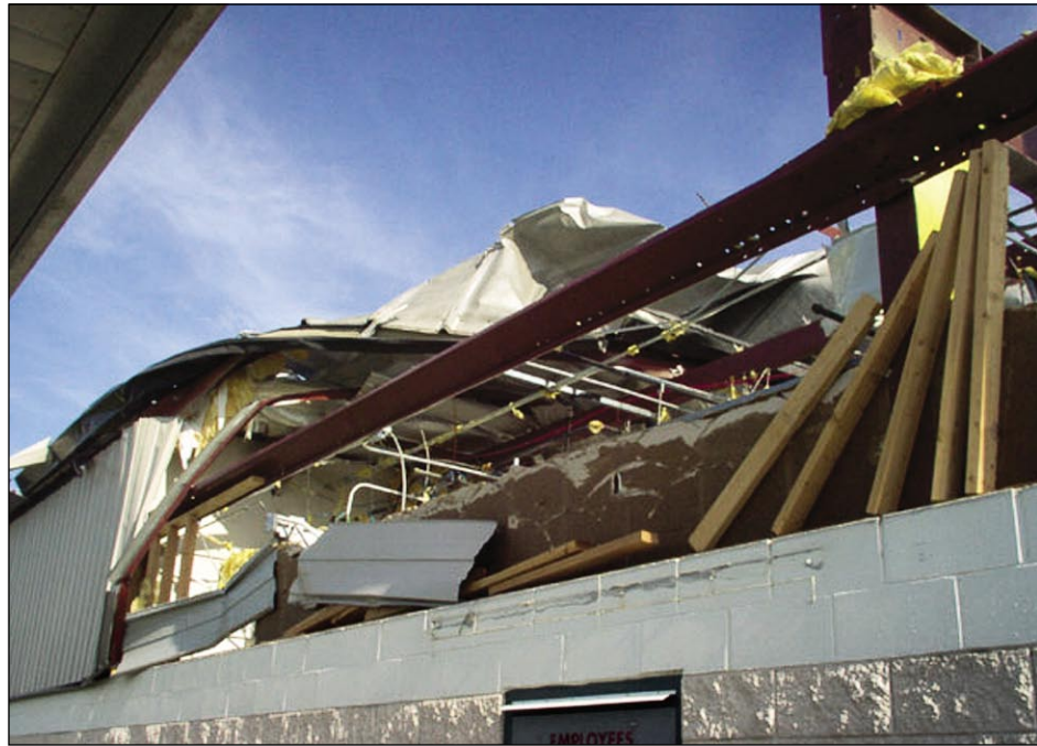
Figure 6-2. Failure of wood stud wall supporting wall panels above masonry wall (Charlotte County EOC)
