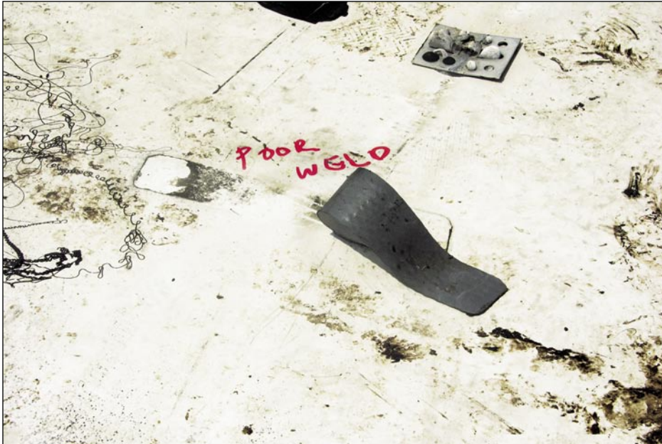
Figure 5-82. The LPS conductor pulled away from the conductor connector at the top of the photo. The conductor was also attached to the membrane with poorly welded strips of PVC (Port Charlotte).
