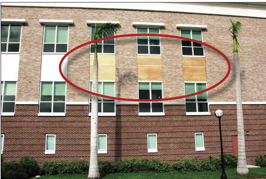
Figure 5-20. Plywood panels installed where aluminum spandrel panels were blown out of the curtain wall (Punta Gorda)
