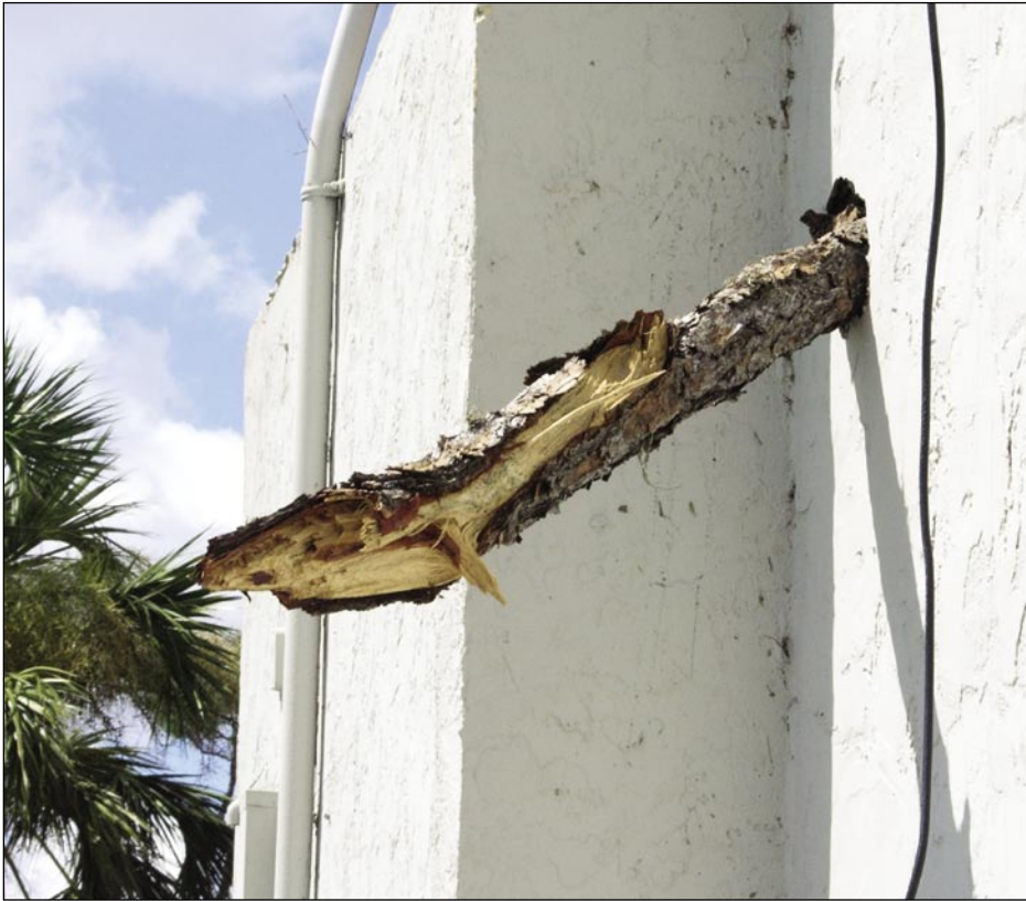
Figure 3-35. Impact of tree branch through the stucco and metal lath wall system of a fire station. The branch was about 5 inches in diameter and protruded about 3 \frac{1}{2} feet out of the wall (Aqui Esta, east of Punta Gorda Isles).
