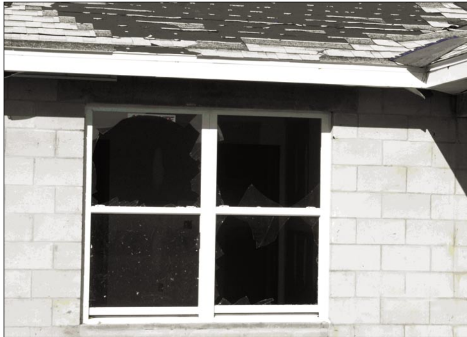
Figure 5-12. Three of four panes broken by windborne debris; other windows in this house also broke (Deep Creek).
