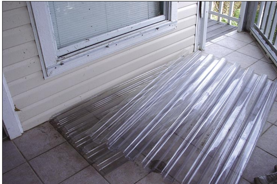
Figure 5-15. All of the windows on this house were covered by plastic shutters, many of which were blown off during the hurricane, resulting in several broken windows (North Captiva Island).
