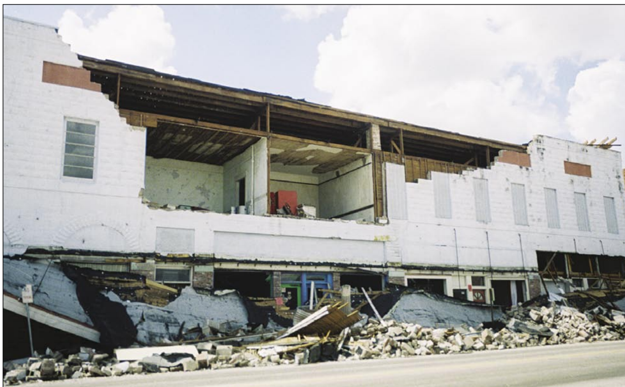
Figure 3-25. Example of unreinforced masonry wall and parapet collapse due to breaching of roof (on opposite side of building) (Wauchula)
