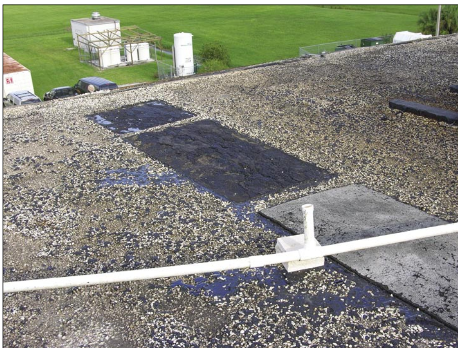
Figure 5-60. This view of the back side of the upper roof of a hospital (see Figure 6-8) shows that the missing gutter and asphalt plank walkway pad were blown away (Arcadia).
