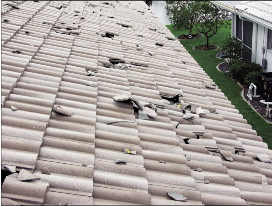
Figure 5-49. A view of the roof on the back side of the residence shown in Figure 5-41. Tiles (including a hip tile) from the front garage roof landed in this area and broke several field tiles (Deep Creek).
