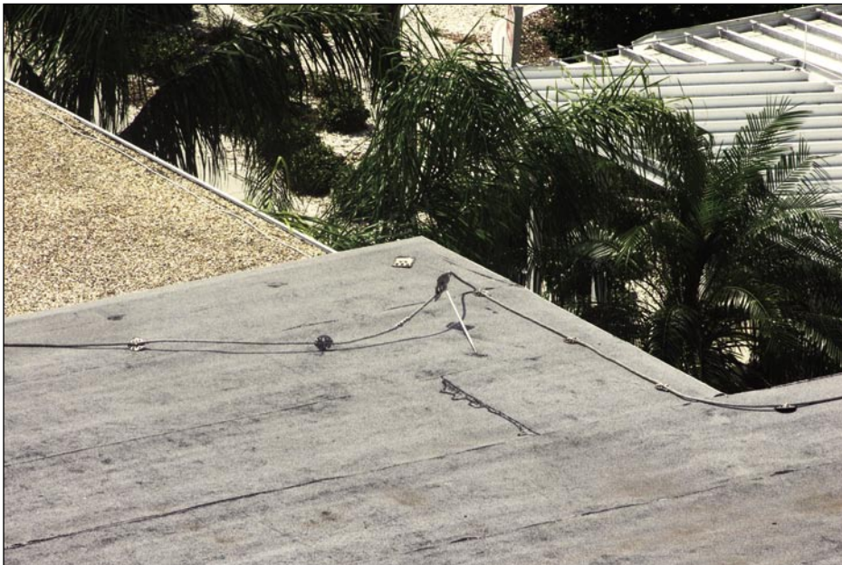
Figure 5-83. The conductor connectors detached from the cap sheet on a hospital's BUR. The air terminal was also displaced (Port Charlotte).
