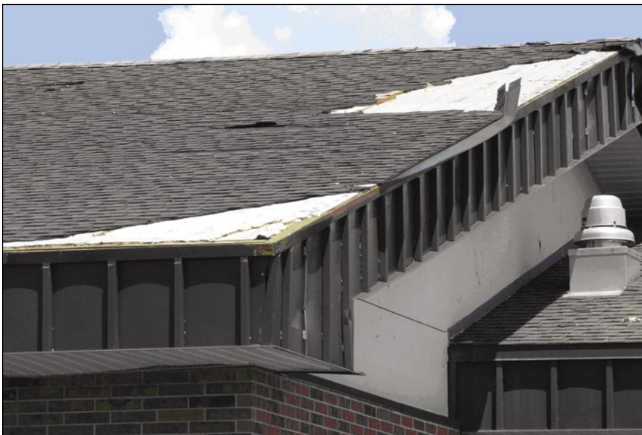
Figure 5-29. Edge flashing that caused a progressive failure of the shingles (Deep Creek)
