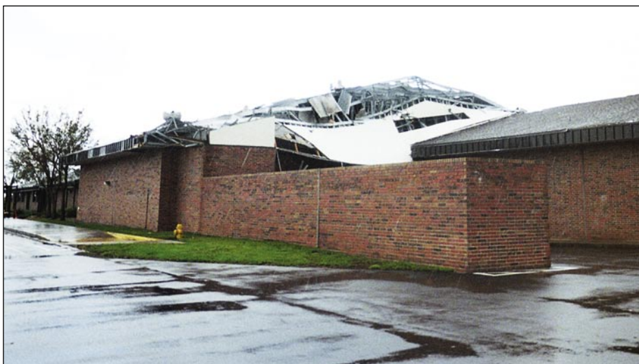
Figure 6-12. Collapsed gable end wall at an elementary school (Deep Creek)
