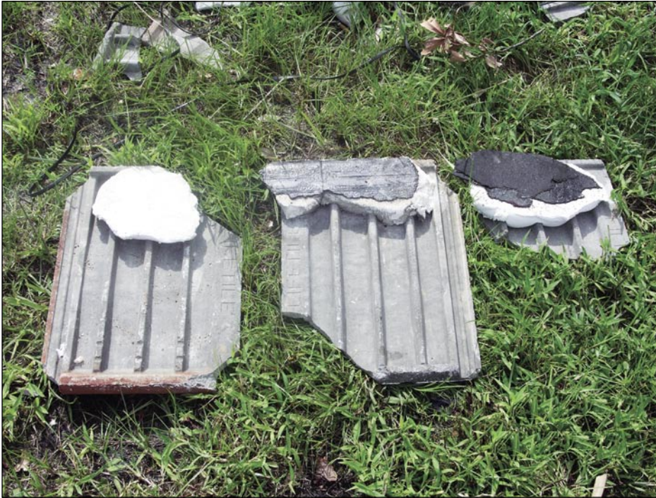
Figure 5-33. Tile debris from the roof shown in Figure 5-32 (Port Charlotte)
