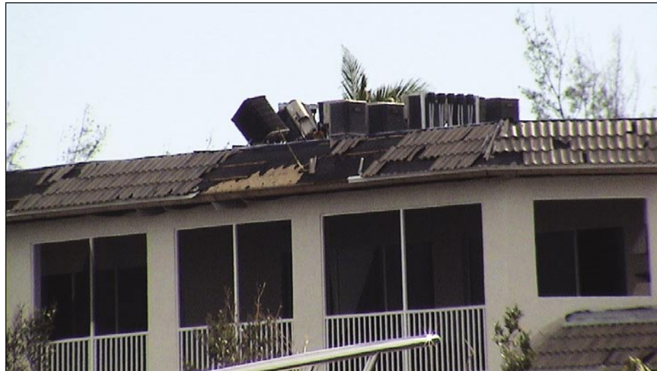
Figure 3-29. Dislocation of rooftop equipment (Pine Island)
