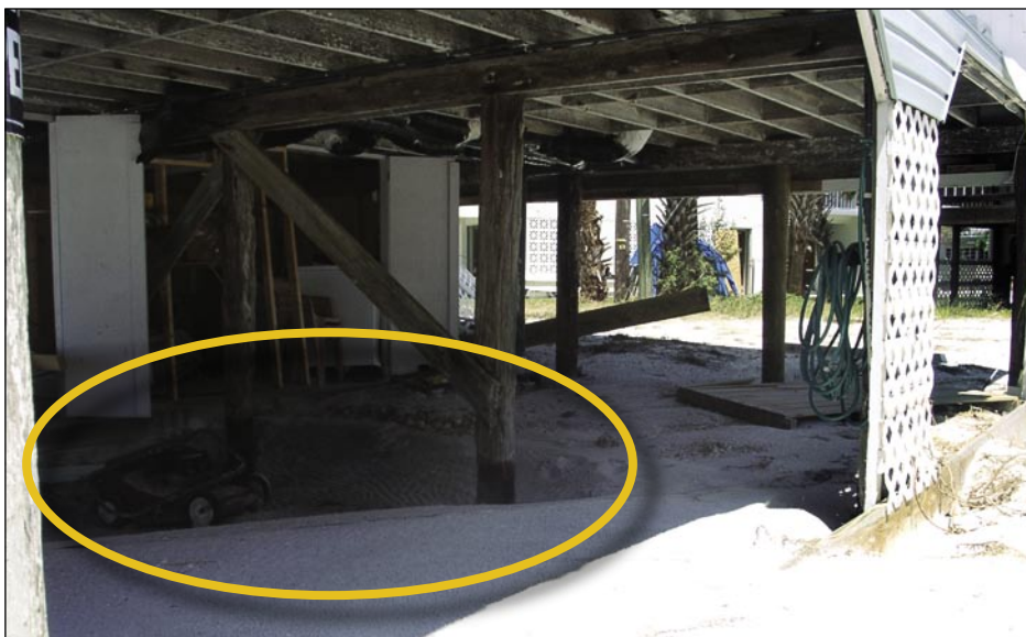
Figure 3-49. Minor scour around pile (Fort Myers Beach)
