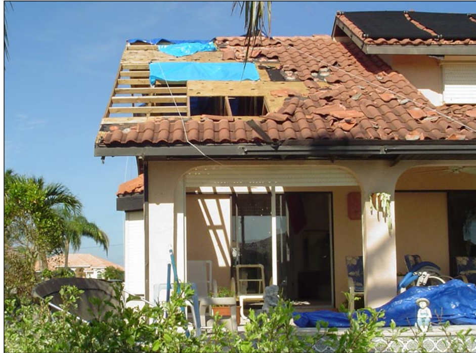
Figure 3-18. Example of roof decking loss on one-story house (Punta Gorda)
