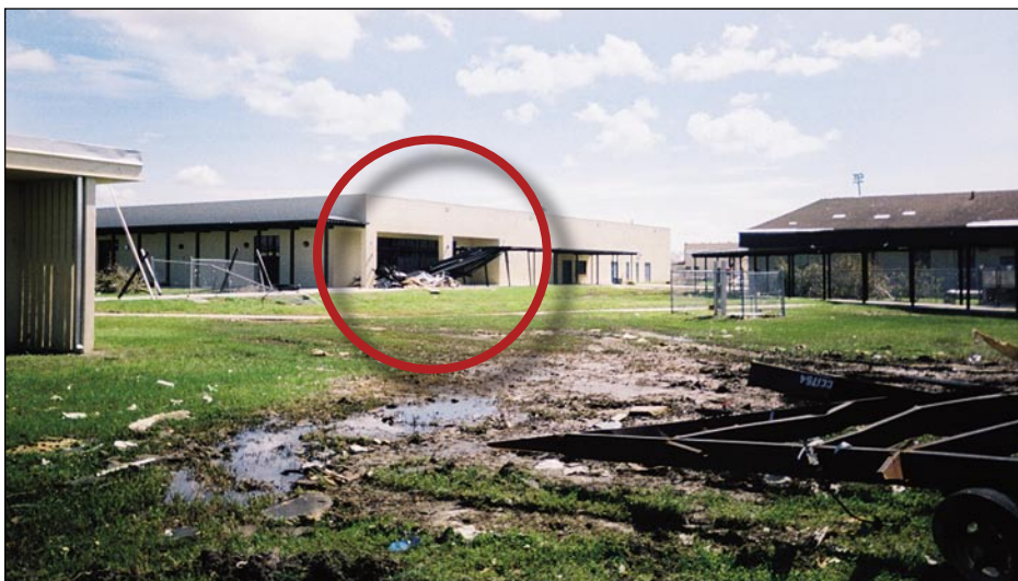
Figure 6-15. Collapsed metal walkway canopy at a high school (Punta Gorda)
