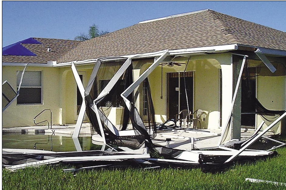
Figure 4-25. Typical consequence of corner post failure (Punta Gorda Isles)
