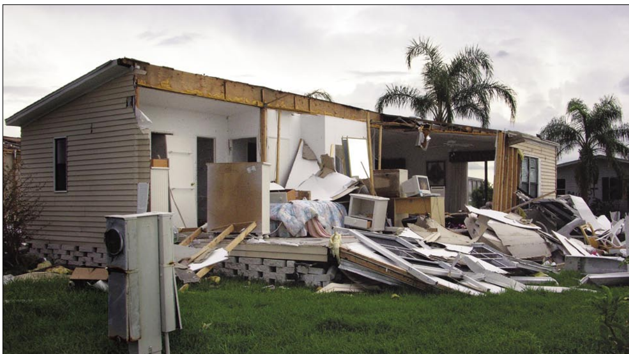
Figure 3-8. Post-1994 manufactured home with major roof and wall failure (east of Port Charlotte)
