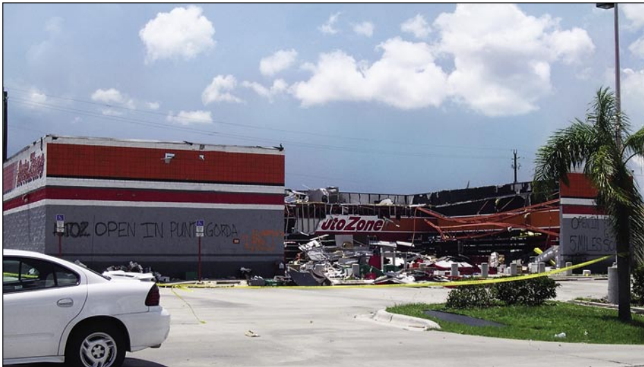
Figure 3-11. Damage to a pre-2001 FBC masonry building with steel joist roof framing and metal deck (Port Charlotte)
