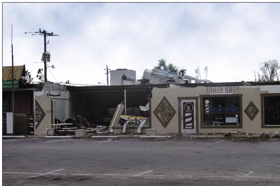
Figure 4-14. Partial failure of an unreinforced concrete masonry commercial structure (Port Charlotte)
