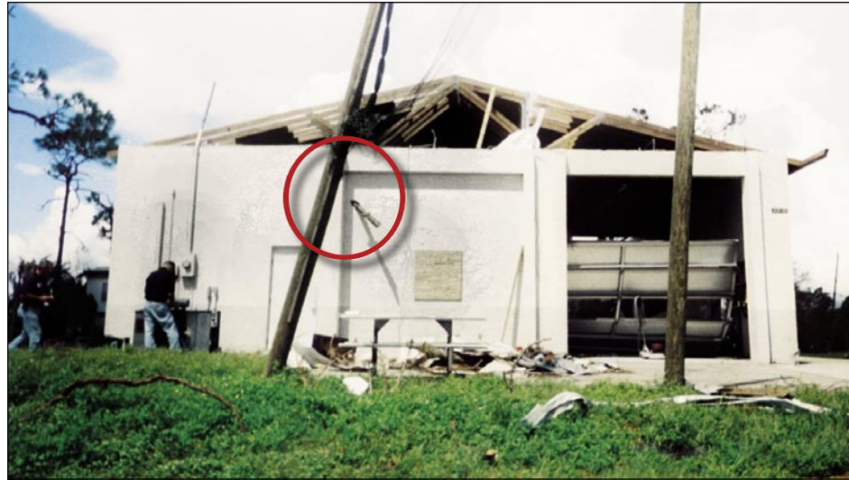
Figure 3-57. Gable end wall collapse and rolling and sectional door failure at fire station (Aqui Esta, east of Punta Gorda Isles). A close-up of the missile in the circle is shown in Figure 3-35.
