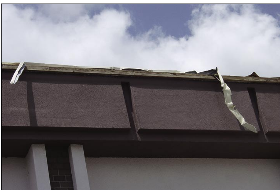
Figure 6-22. Edge flashing failure at Port Charlotte Middle School
