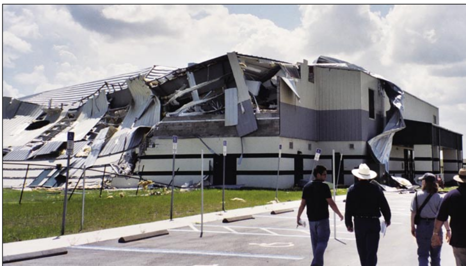
Figure 6-18. End wall failure at Turner Agri-Civic Center (Arcadia)
