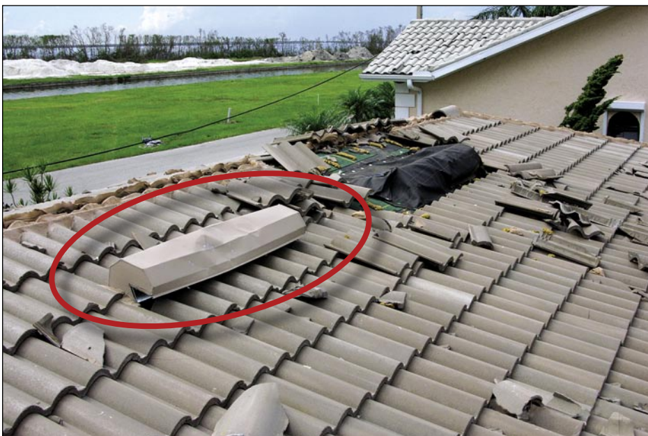
Figure 5-22. The attic vent to the right (temporarily covered with felt) on this foam-set tile roof lifted during the hurricane and allowed water to enter the residence shown in Figure 5-21. The failed vent is like the one on the left (Punta Gorda Isles).
