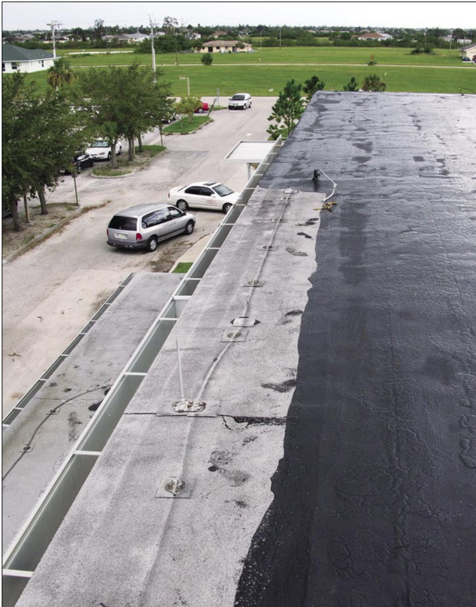
Figure 5-63. The edge flashing had a 2-inch vertical flange that extended into the gutter. The flashing was not cleated (Cape Coral).
