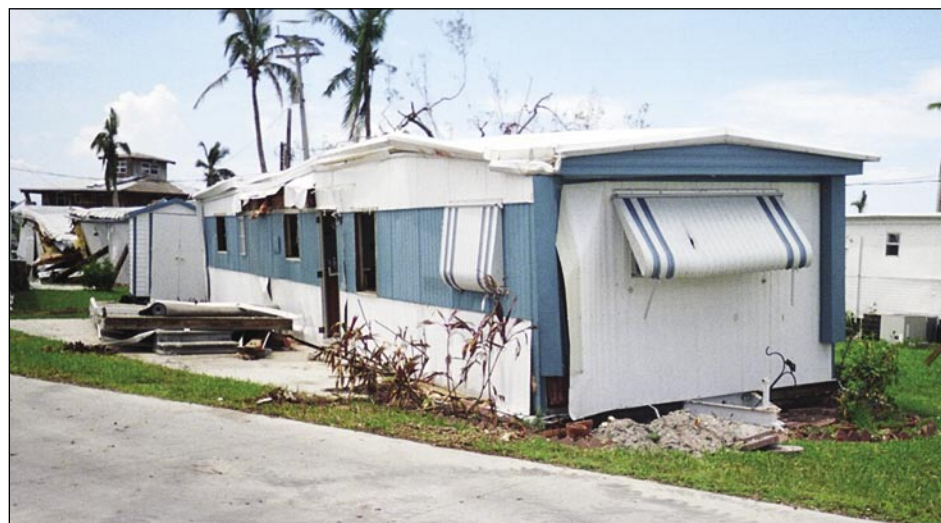
Figure 3-7. Pre-1976 manufactured home unit displaced from its foundation, damaging the structure itself (Pine Island)
