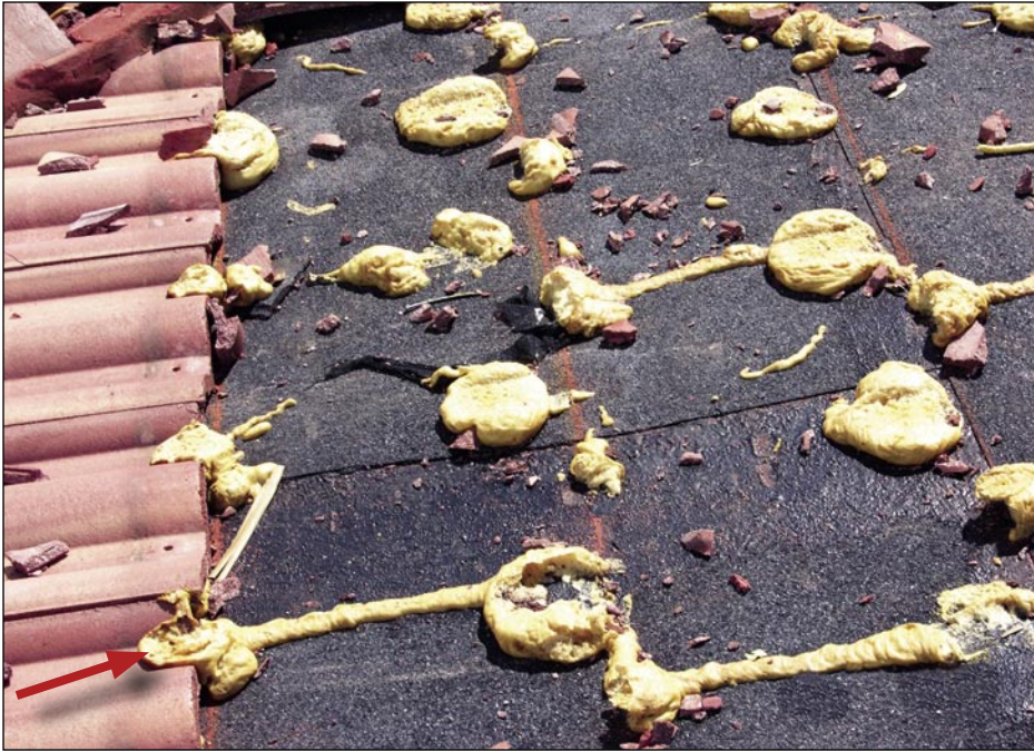
Figure 5-43. This photo clearly shows insufficient contact area of foam-set paddy on the bank's roof (Punta Gorda Isles).
