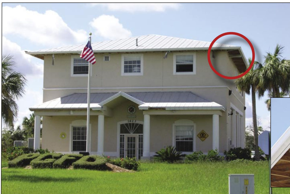
Figure 5-71. Essentially all of the perforated aluminum soffit on this fire station was blown away (Aquí Esta, east of Punta Gorda Isles).
