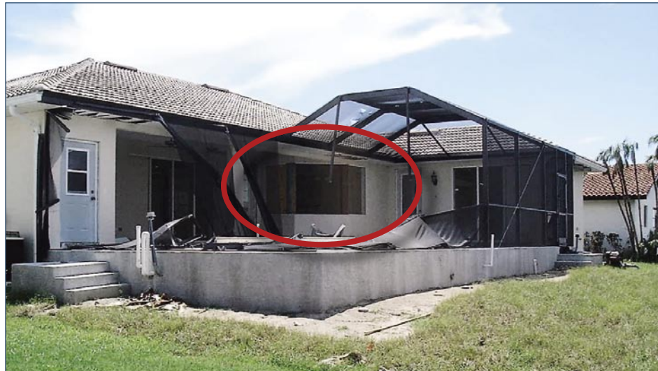
Figure 3-47. Example of damage to pool screen enclosure. Note broken window in center of photo from debris (Punta Gorda Isles).
