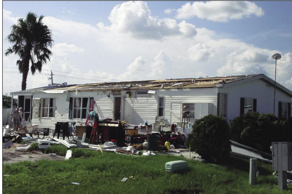
Figure 4-10. Post-1994 HUD manufactured home with significant roof damage (peeling of roof panels) resulting from collapse of attached accessory structure (Zolfo Springs).
