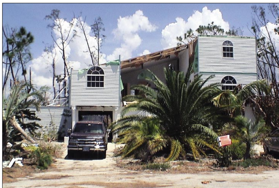
Figure 4-5. Failure of the roof over a cathedral ceiling from pressurization of the house when the window failed on the windward face (Pine Island)
