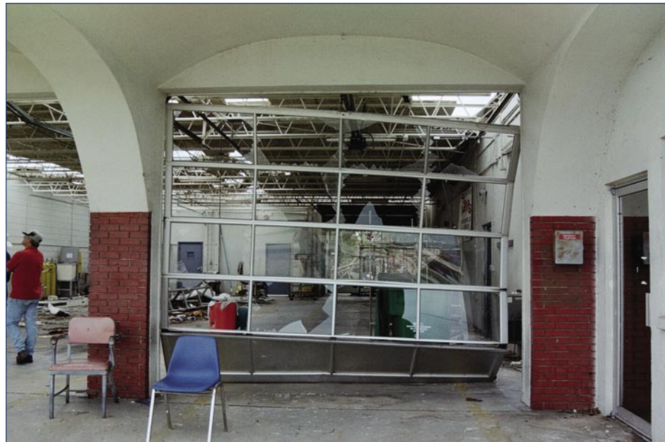
Figure 6-5. View of damaged garage door and interior of Port Charlotte Fire Station No. 1; note missing roof deck panels over apparatus bay.
