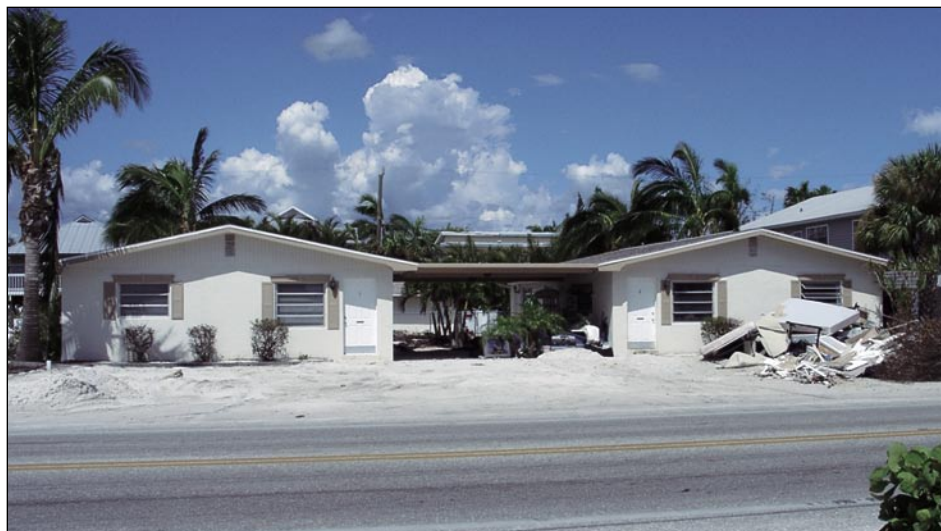
Figure 3-52. Typical house with first- floor living space at grade sustained 2 to 3 feet of storm surge damage (lack of wall damage suggests low velocity flows) (Fort Myers Beach)
