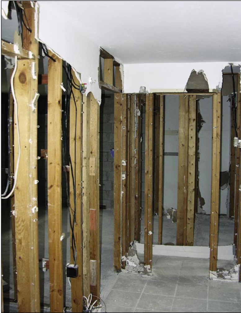
Figure 5-21. After the attic vent failed, water entered this residence. Wet carpeting and a substantial amount of wet gypsum board had to be removed (Punta Gorda Isles).
