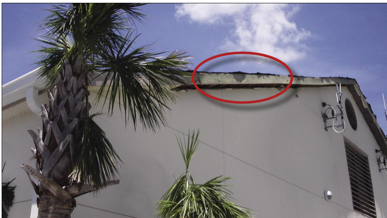
Figure 6-7. Damaged soffit at Punta Gorda Public Safety Complex
