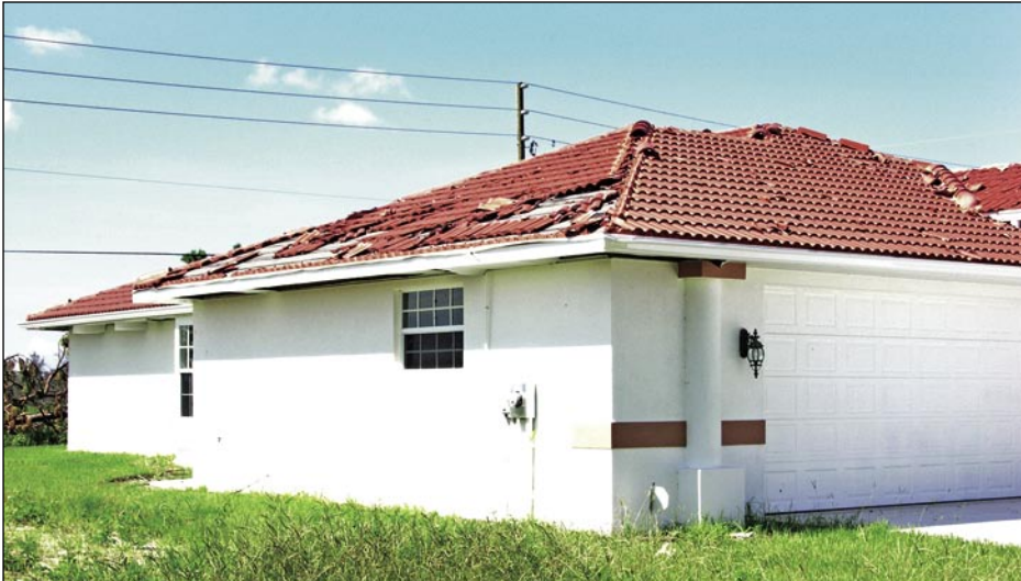
Figure 5-35. Windborne debris (likely tiles from this roof) broke several of the field tiles (Deep Creek).
