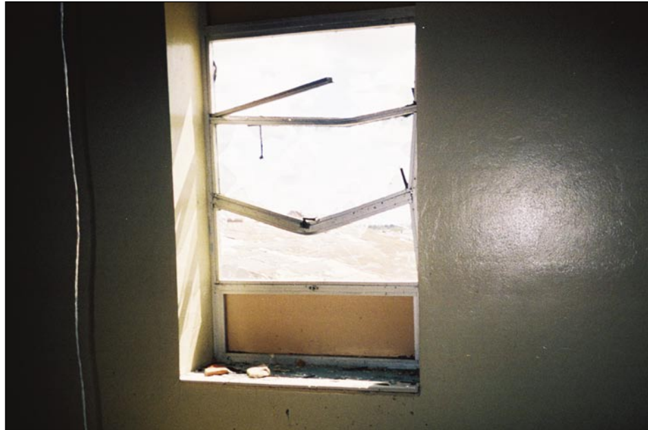
Figure 6-14. Broken window damage at a high school (Punta Gorda)
