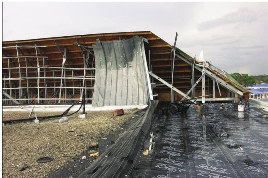
Figure 5-53. The wood and metal framed superstructure blew away and exposed the lightweight concrete roof deck (Port Charlotte).
