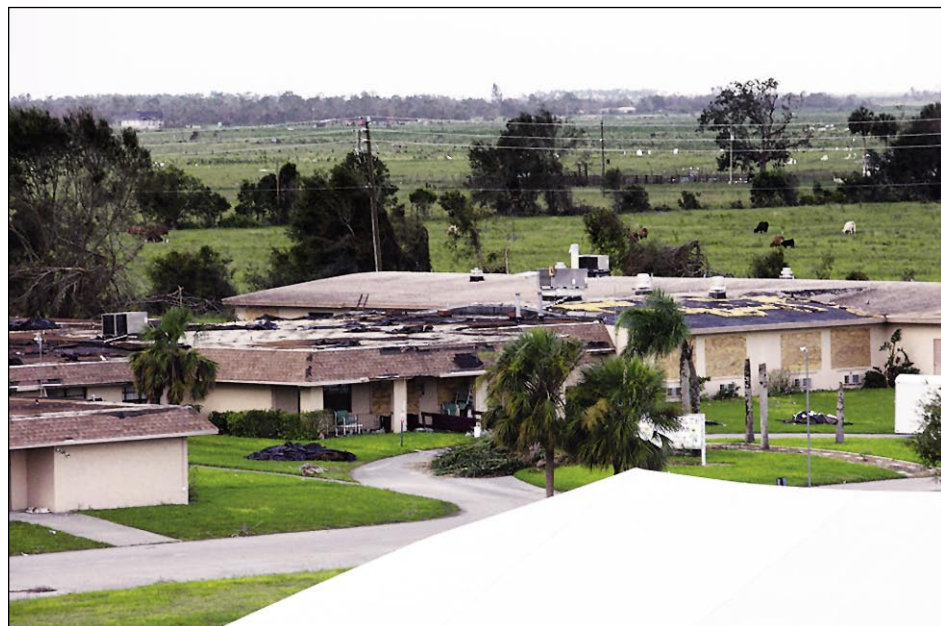
Figure 6-9. Roof covering damage resulting in water intrusion, which required evacuation of a skilled nursing facility (Arcadia)
