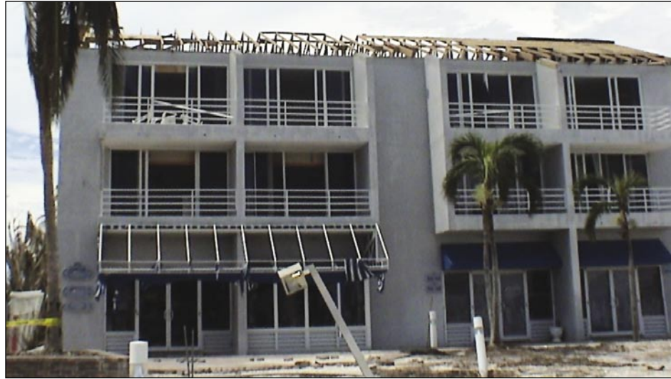
Figure 3-6. Damage to older multi-family building roof deck with inadequately supported and braced overhang (Captiva Island)
