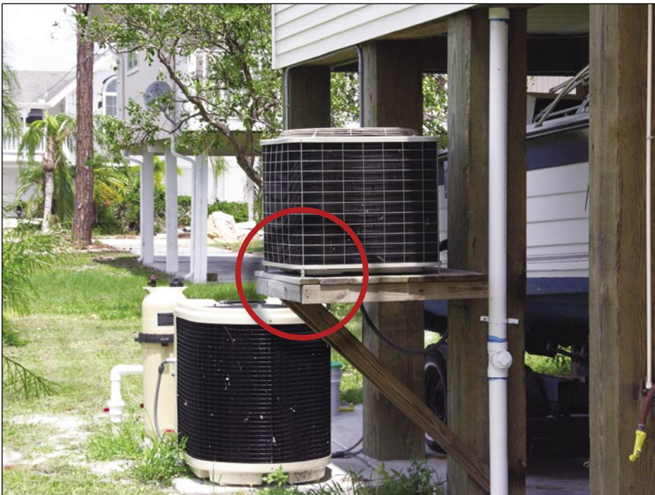
Figure 5-73. Condenser on the elevated platform attached with four angle brackets. The other condenser, located adjacent to it on the ground, should also have been on an elevated platform to account for storm surge (Pine Island).
