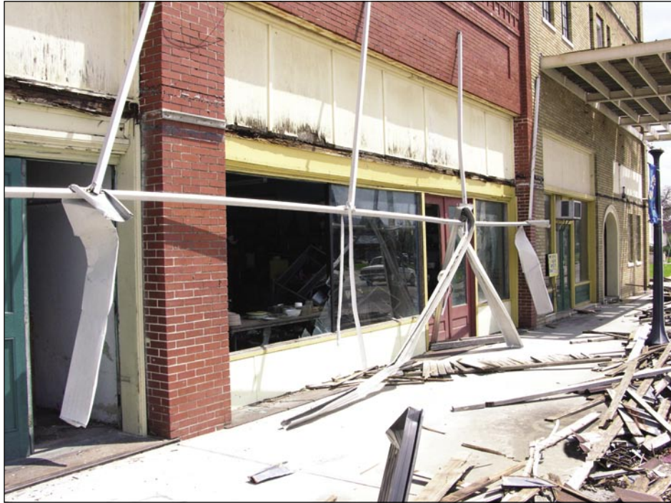
Figure 5-17. Broken glass in windows and doors in this building. Buildings across the street also had several broken windows caused by windborne debris (Wauchula).
