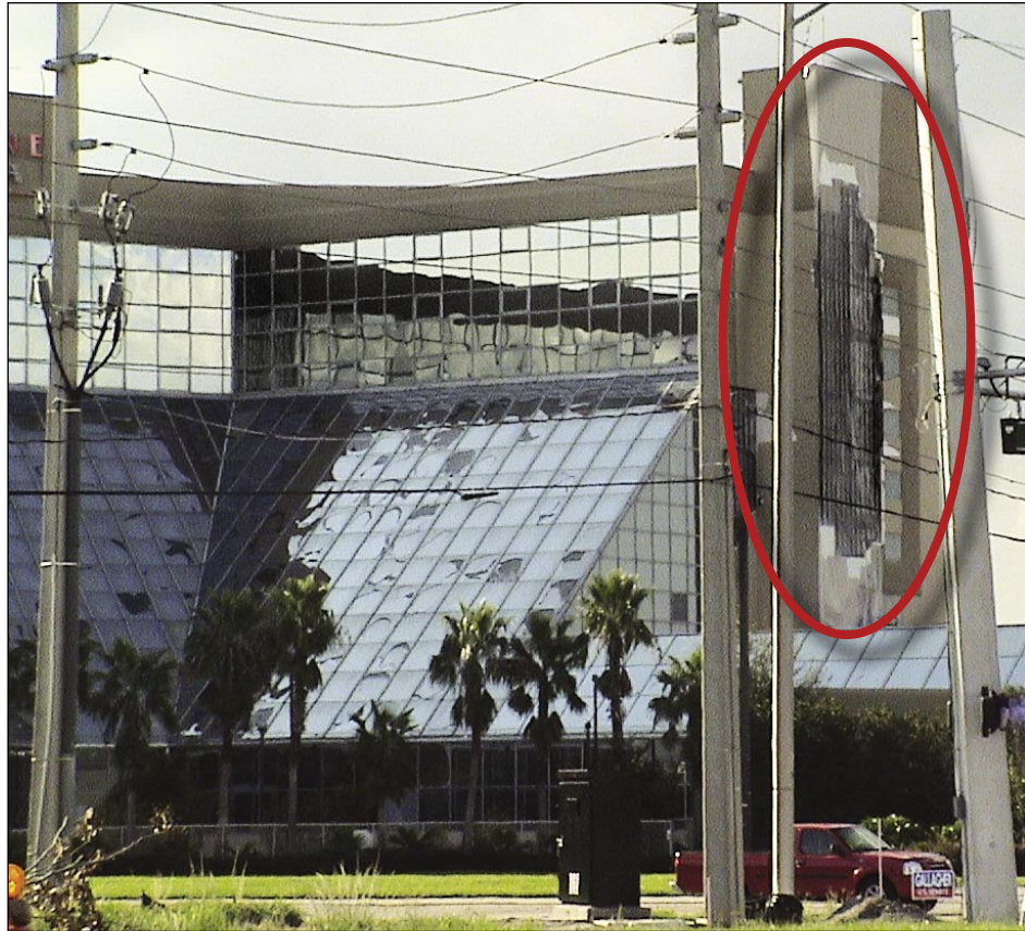
Figure 3-33. Damage to glass atrium of high-rise hotel. Note the loss of EIFS, which was the cause of the glass breakage (Orlando).
