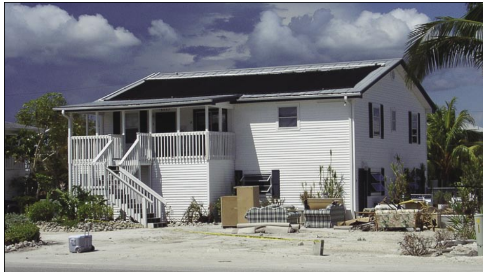
Figure 3-51. Storm surge damage of 2 to 3 feet limited to lower floor of two-story house (Fort Myers Beach)
