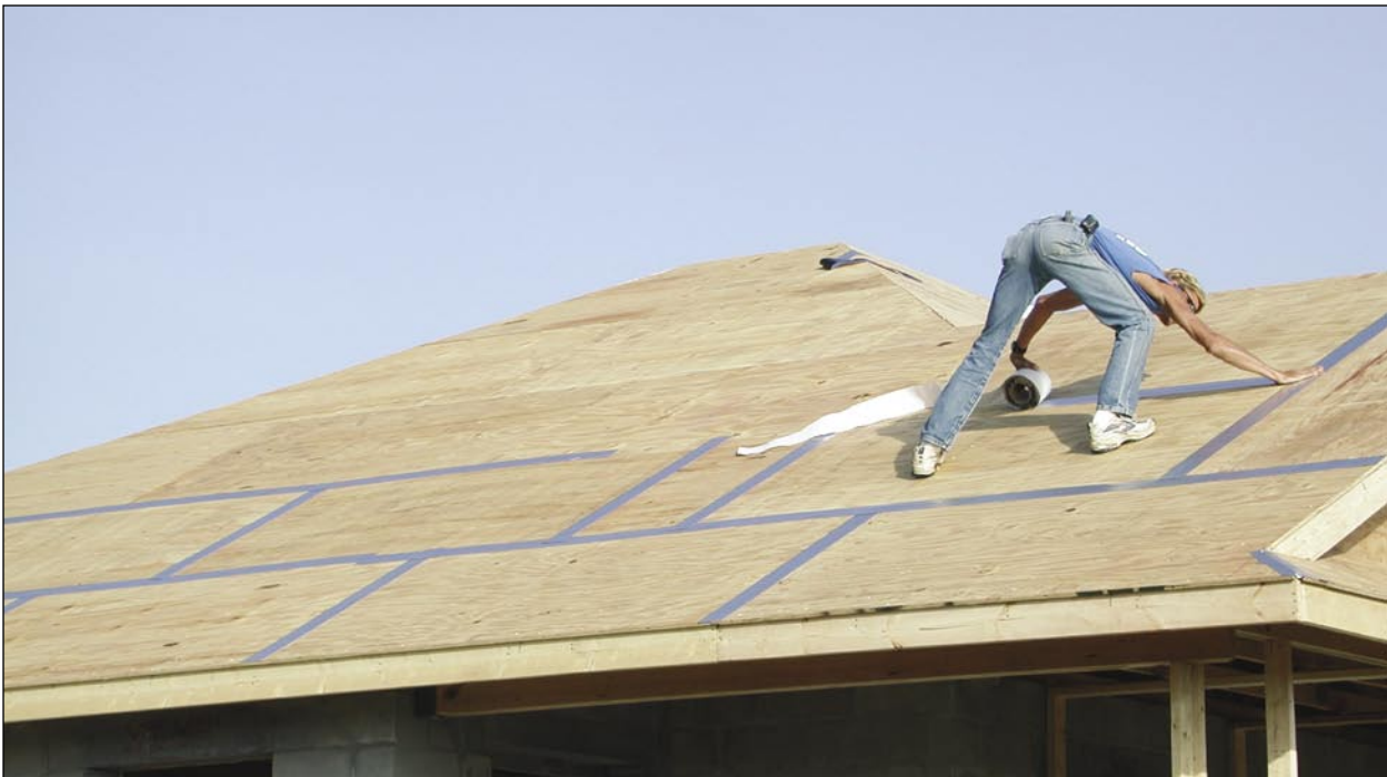
Figure 5-23. Installation of self-adhering modified bitumen tape at sheathing joints, as part of an enhanced underlayment system on a Fortified...for safer living™ house under construction (IBHS)
