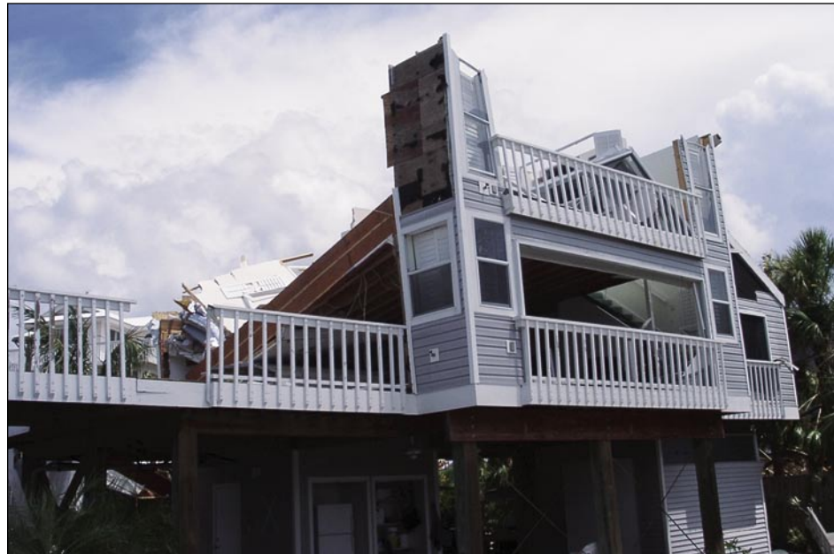
Figure 4-3. An older building that was renovated for architectural improvements a few years ago collapsed due to limited load path connections (North Captiva Island).
