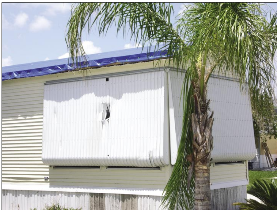
Figure 5-14. Metal awning shutter penetrated by a missile (Zolfo Springs)
