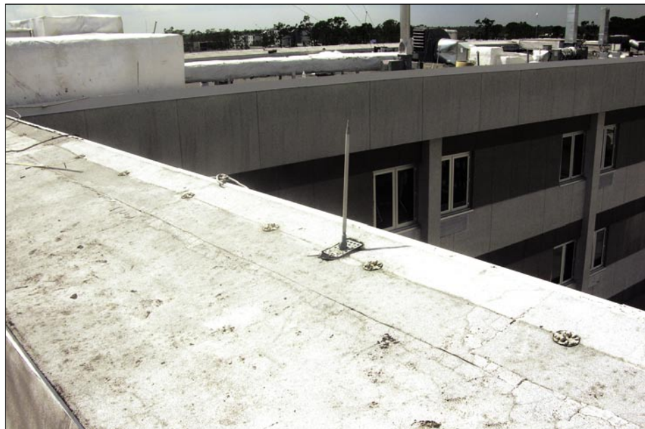
Figure 5-81. The LPS conductor on this hospital blew away, but the air terminal was still attached. A lightning strike to this air terminal would not be safely dissipated (Port Charlotte).
