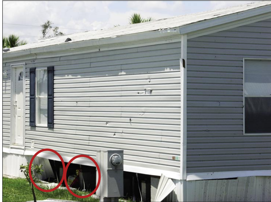
Figure 5-66. The vinyl siding on this manufactured house was ruptured in several locations by windborne debris (most of which were likely building envelope components from other nearby manufactured houses). Note the missing skirt and loose foundation anchor straps (Zolfo Springs).
