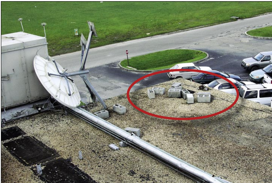
Figure 5-79. This satellite dish at a hospital was held down only with CMU. Note the loose LPS conductors and displaced air terminal at the corner (Arcadia).
