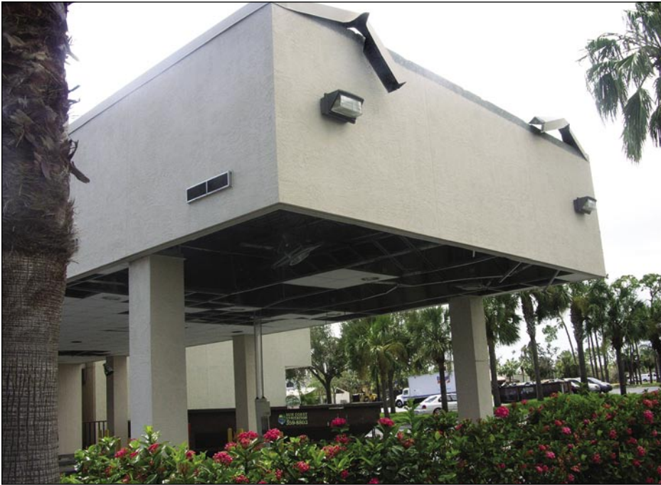
Figure 5-70. Loss of soffit at a bank drive-through. Note the coping damage (Port Charlotte).
