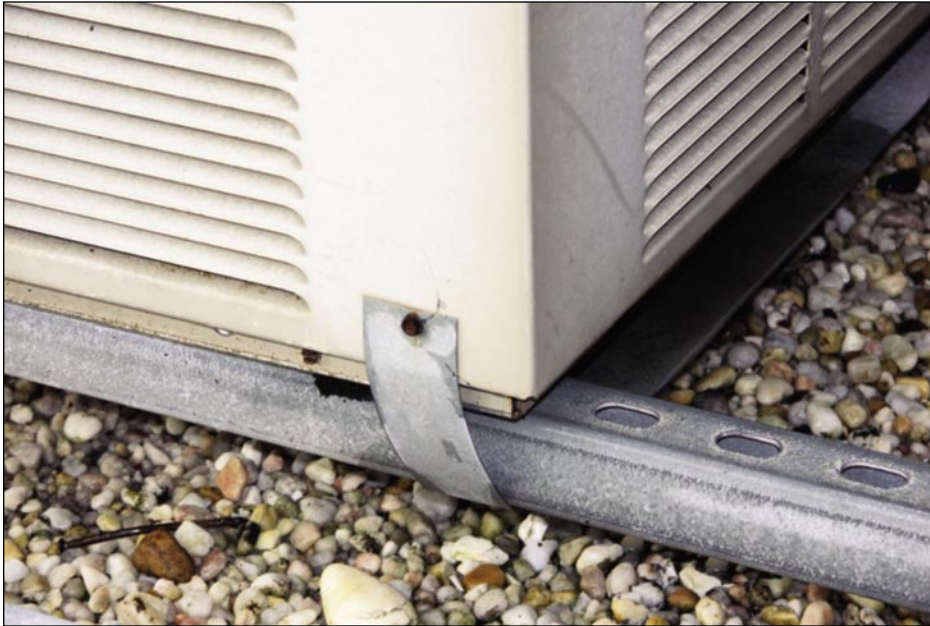
Figure 5-75. Rooftop condenser anchored to a support rail, but with only one small screw (which was corroded) used to connect the strap (Port Charlotte).
