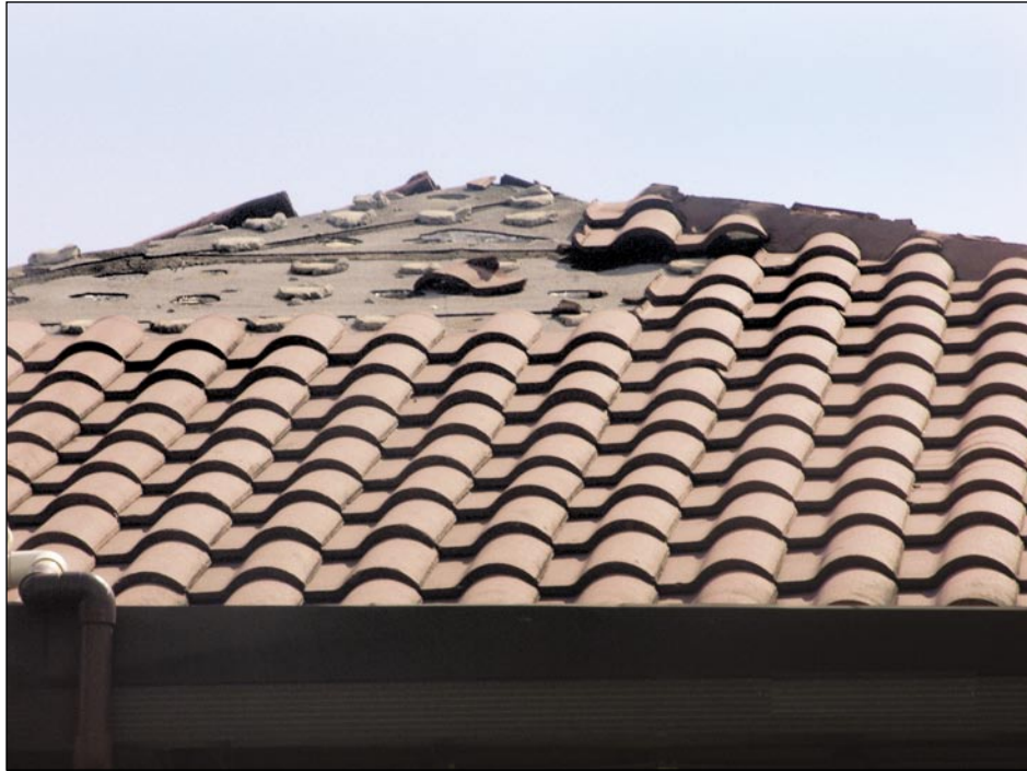
Figure 5-31. Mixed failure modes occurred on this mortar- set tile roof (Port Charlotte).
