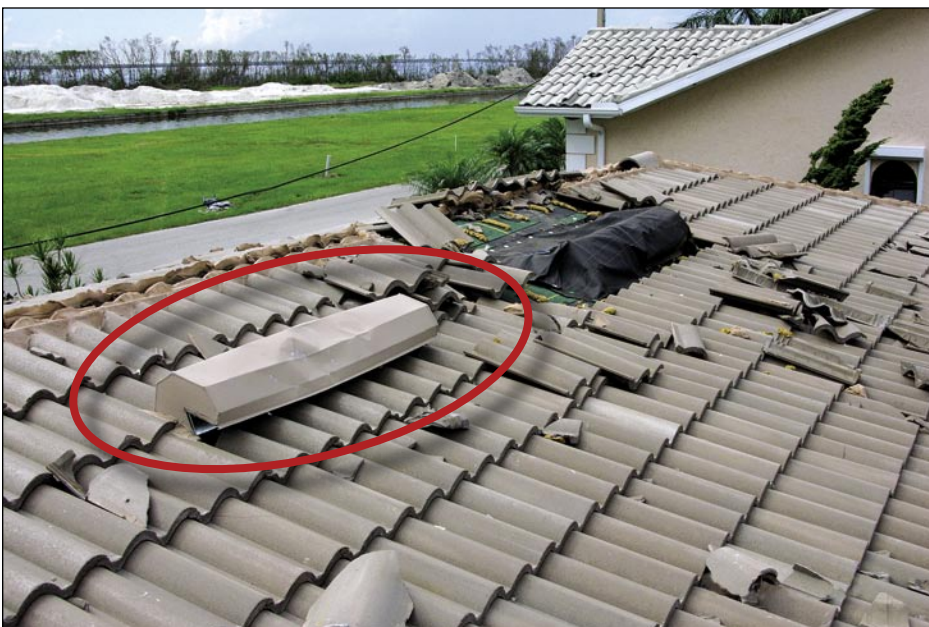
Figure 5-22. The attic vent to the right (temporarily covered with felt) on this foam-set tile roof lifted during the hurricane and allowed water to enter the residence shown in Figure 5-21. The failed vent is like the one on the left (Punta Gorda Isles).
