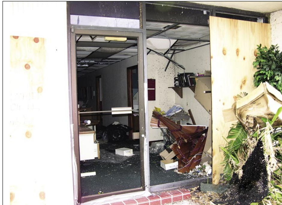
Figure 5-2. Tempered glass in office building entry door and side windows broken by missiles (Punta Gorda)
