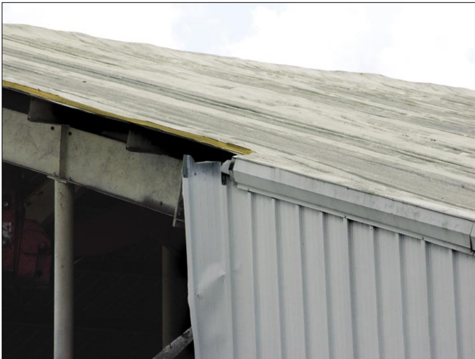
Figure 5-58. The metal wall panels and metal edge flashing on this building blew away, but the exposed fastener R-panels with an SPF covering did not progressively fail (Wauchula).
