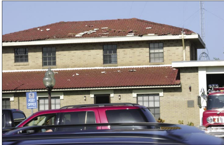
Figure 5-37. Fire station with at least three battens blown off. Some tiles remained attached (Fort Meade).
