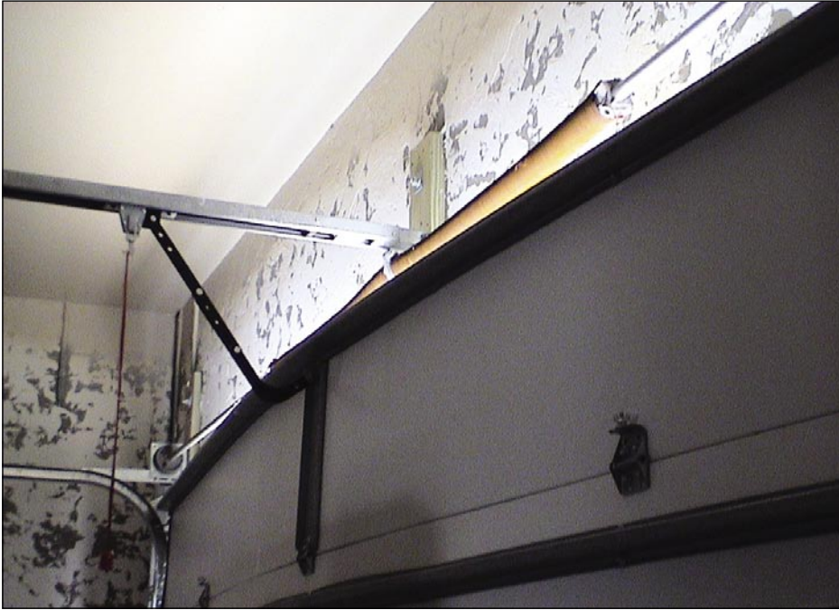
Figure 5-6. Garage door failed because the removable stiffener bar was not in place at the time of the hurricane (Punta Gorda Isles).
