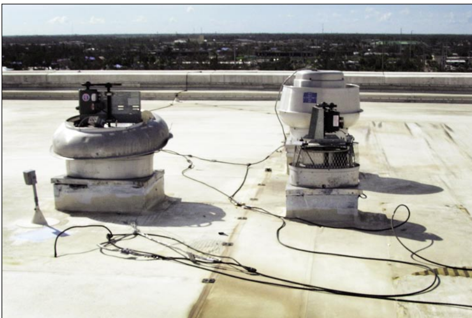
Figure 5-76. Cowlings blown off two exhaust fans in the foreground. Note also the loose LPS conductors and missing walkway pad (Punta Gorda).
