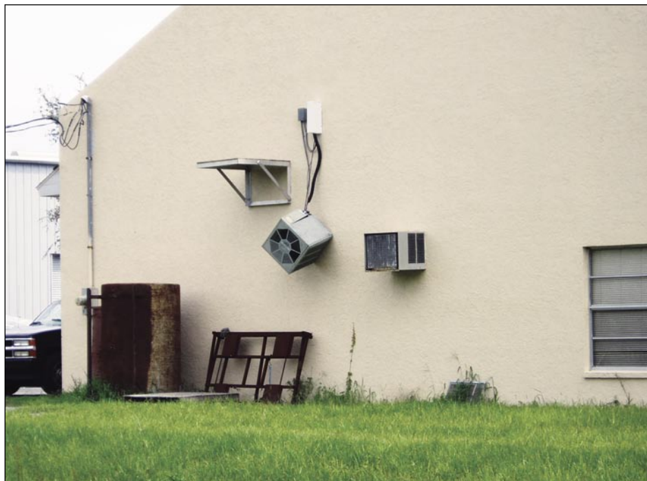
Figure 5-74. Condenser unit displaced from the elevated platform (Port Charlotte)
