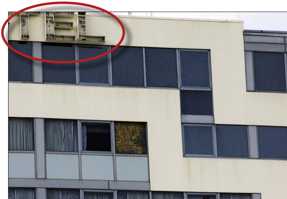
Figure 5-16. Window most likely broken by missing plastic lens covers on hotel sign (see top of building) (Orlando airport area)
