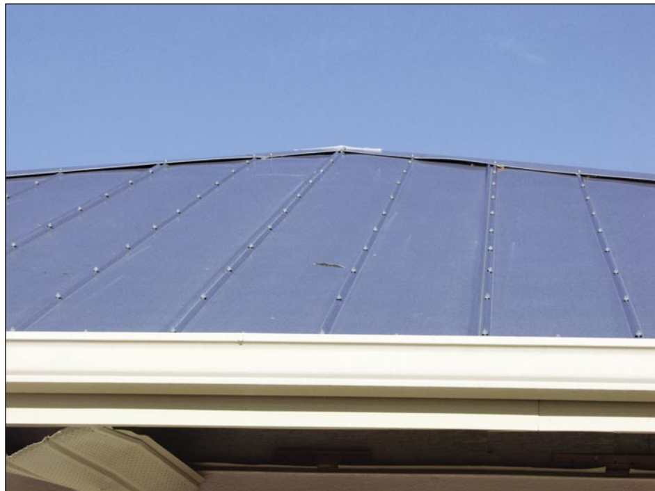
Figure 5-50. The number of fasteners was not increased at the corner, perimeter, hip, or ridge areas (close-up of the residence shown in Figure 5-5). Also note that several of the soffit panels were blown away (Deep Creek).
