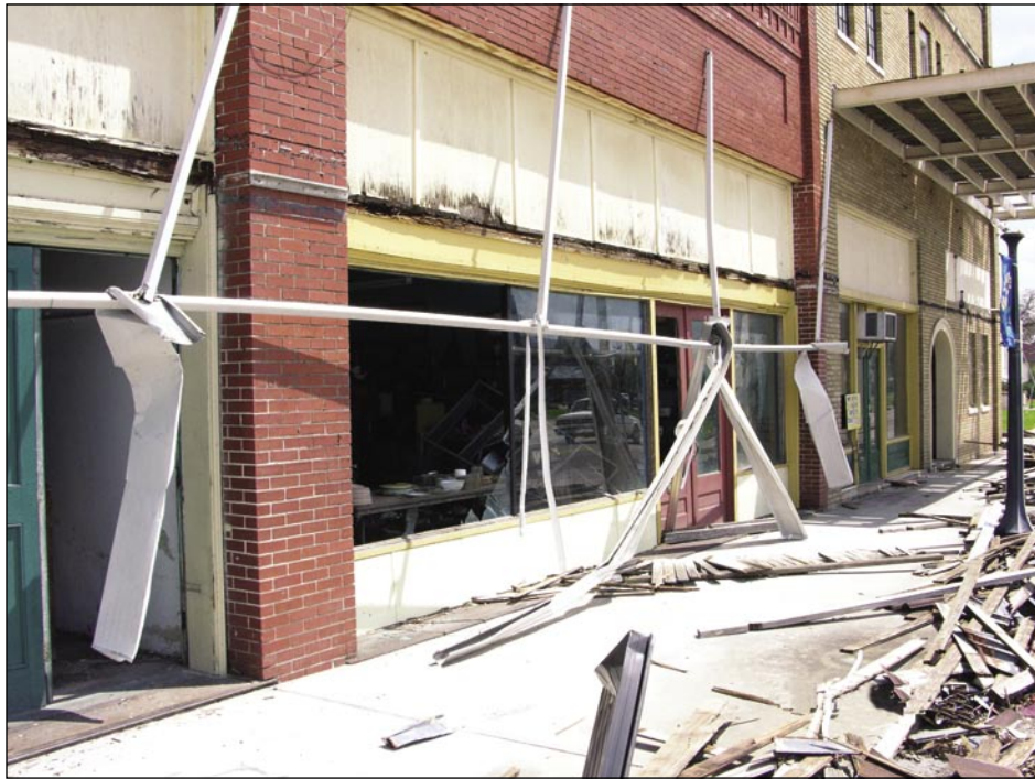
Figure 5-17. Broken glass in windows and doors in this building. Buildings across the street also had several broken windows caused by windborne debris (Wauchula).
