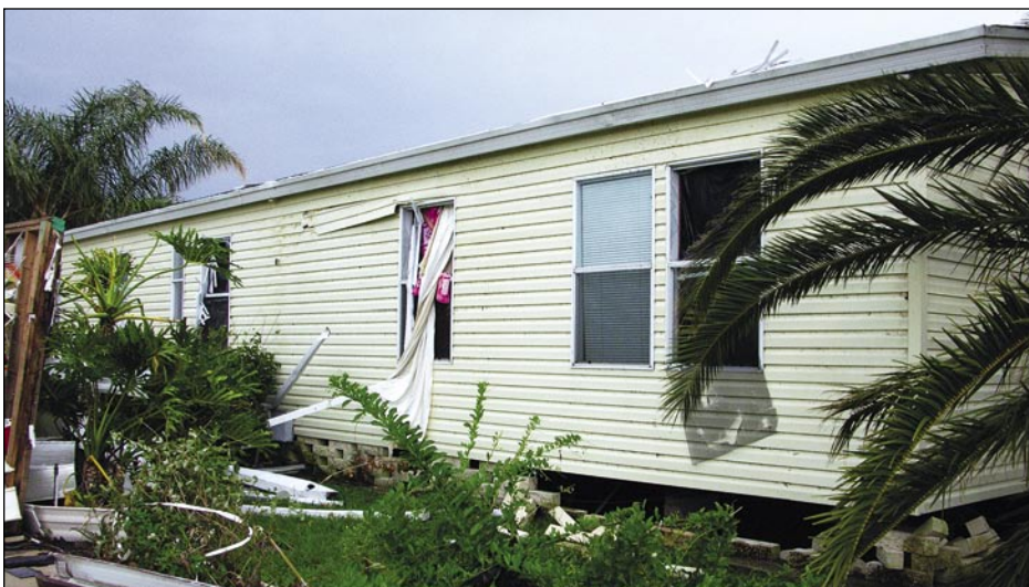
Figure 5-11. Most of the windows on this side of a manufactured home were broken by windborne debris (east of Port Charlotte).
