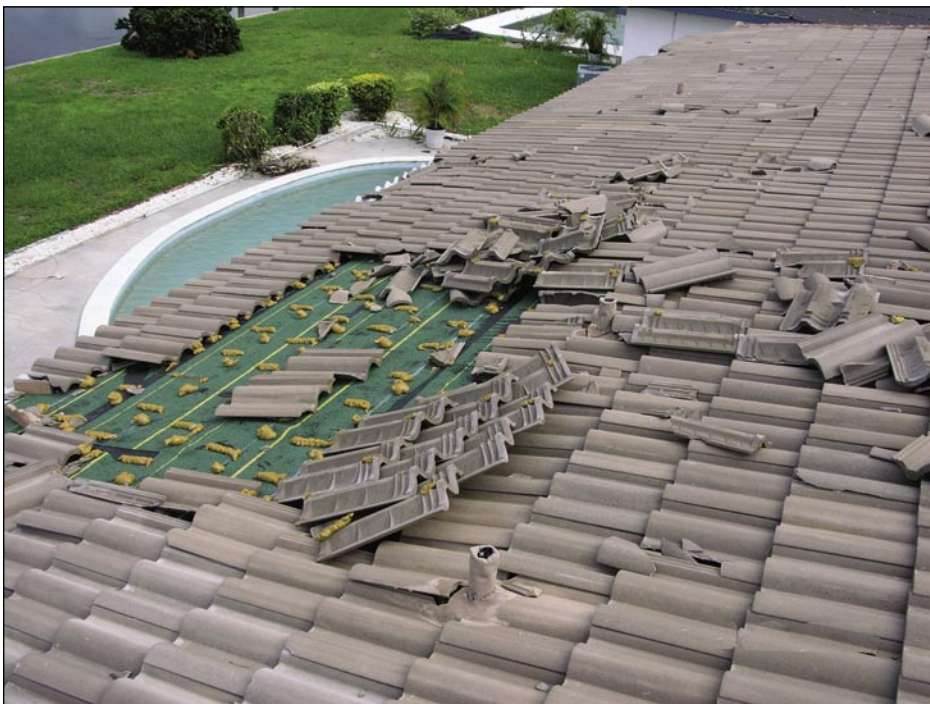
Figure 5-38. In addition to the damage shown in this photo, this one-story roof lost virtually all of the hip and ridge tiles (see Figures 5-22, 5-39, and 5-40) (Punta Gorda Isles).
