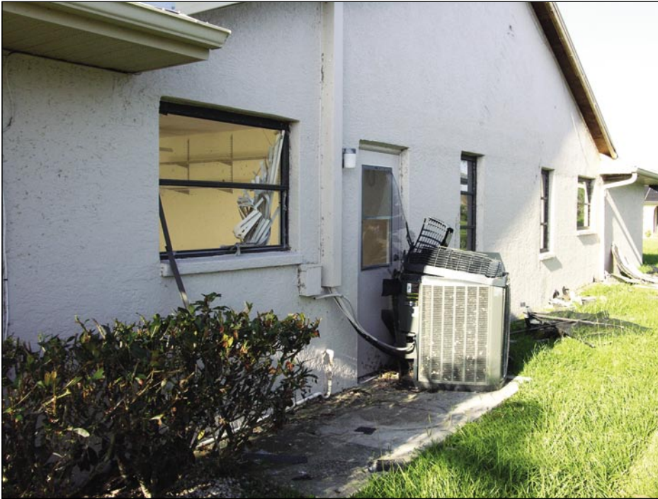
Figure 5-72. This condenser was not anchored to the concrete pad. The electrical and copper tube connections kept it from blowing farther away (Deep Creek).
