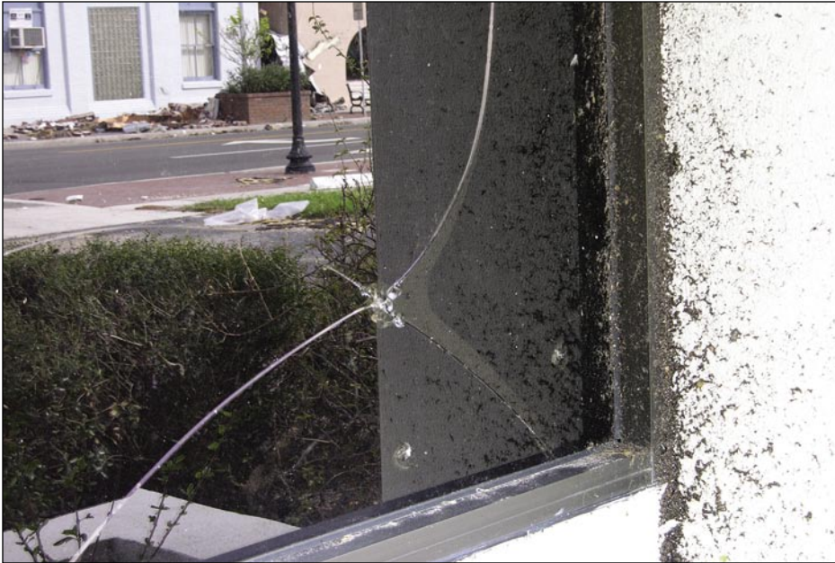
Figure 5-19. Windows broken by aggregate from a nearby BUR. Besides impact at the crack intersection, aggregate chipped the glass in three other locations (Punta Gorda).
