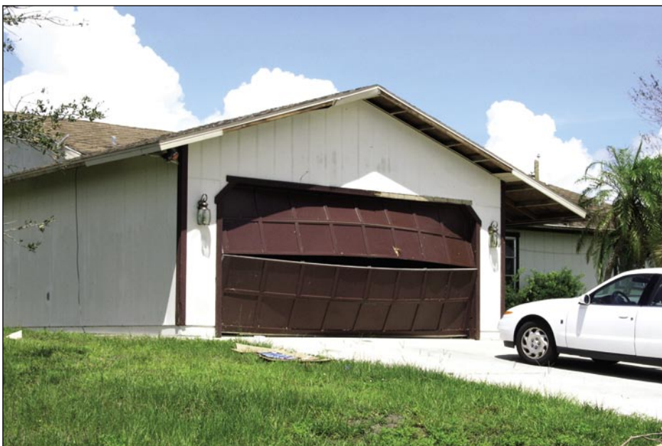
Figure 5-4. Door lacked sufficient strength to resist the suction load (Deep Creek)
