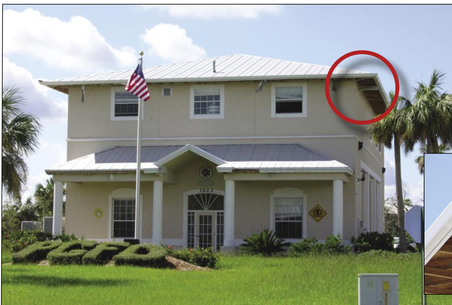
Figure 5-71. Essentially all of the perforated aluminum soffit on this fire station was blown away (Aquí Esta, east of Punta Gorda Isles).
