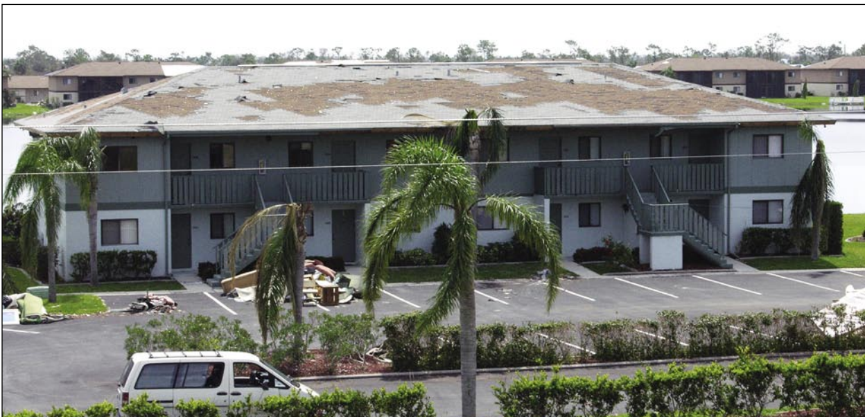
Figure 5-28. Re-covered apartment building (the newer shingles are grey and the older shingles are brown) (Deep Creek).
