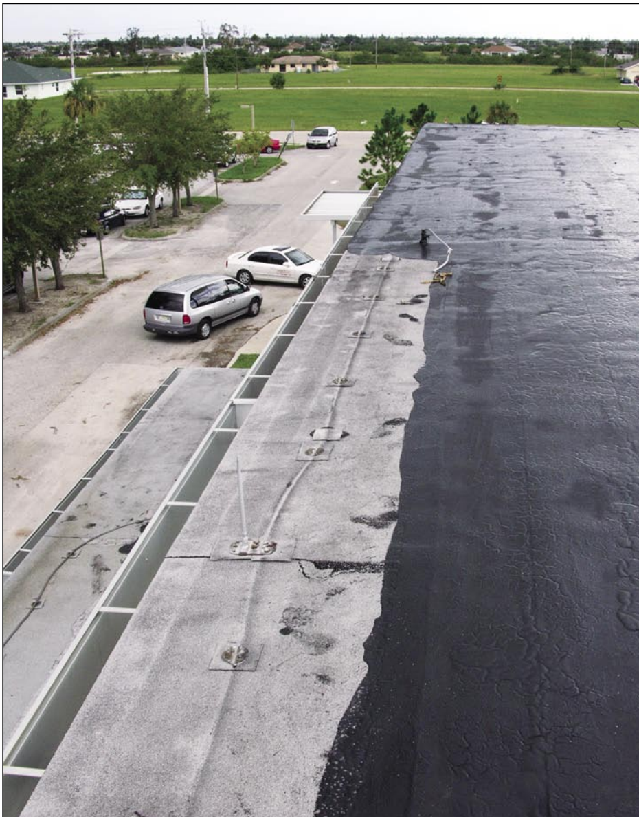
Figure 5-63. The edge flashing had a 2-inch vertical flange that extended into the gutter. The flashing was not cleated (Cape Coral).
