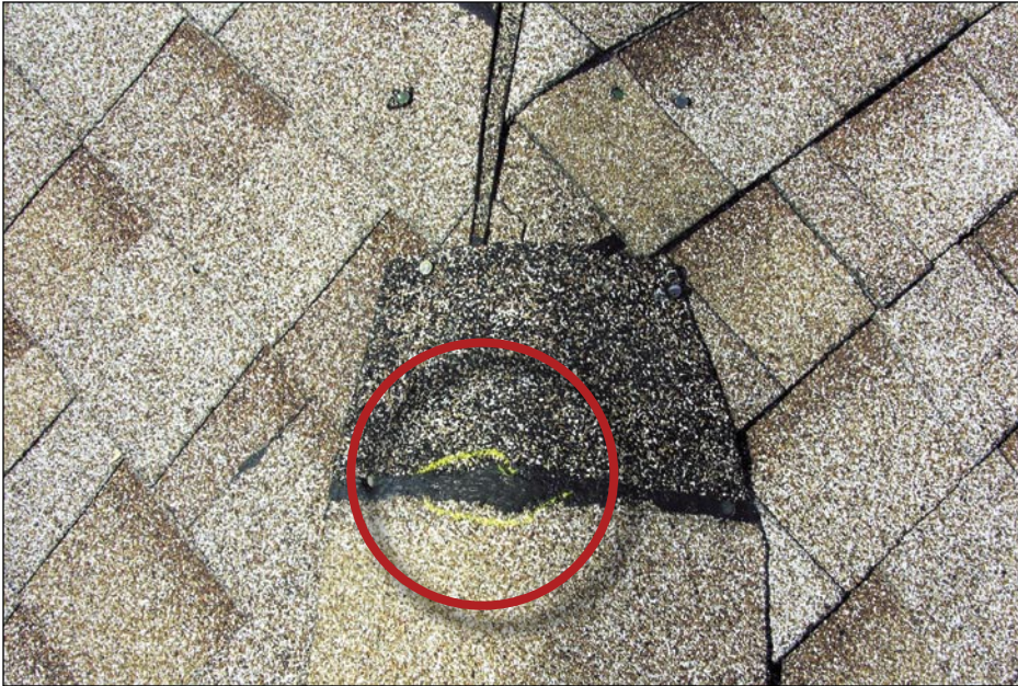
Figure 5-26. Only the portion of the self-seal adhesive that is indicated in yellow had bonded (within the red circle). No bonding occurred on the right side of the hip line (Deep Creek).
