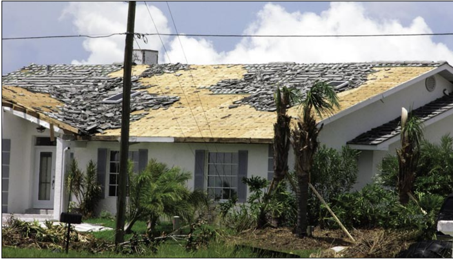
Figure 5-30. A large area of underlayment at this mortar-set flat tile roof blew away. The loss of tile underlayment was atypical (Punta Gorda).
