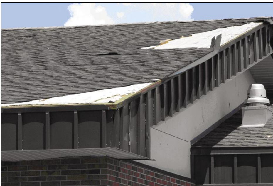
Figure 5-29. Edge flashing that caused a progressive failure of the shingles (Deep Creek)
