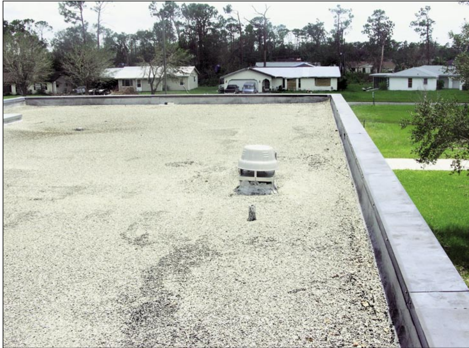
Figure 5-61. Although this roof had an 11-inch high parapet, aggregate was blown off (Port Charlotte).
