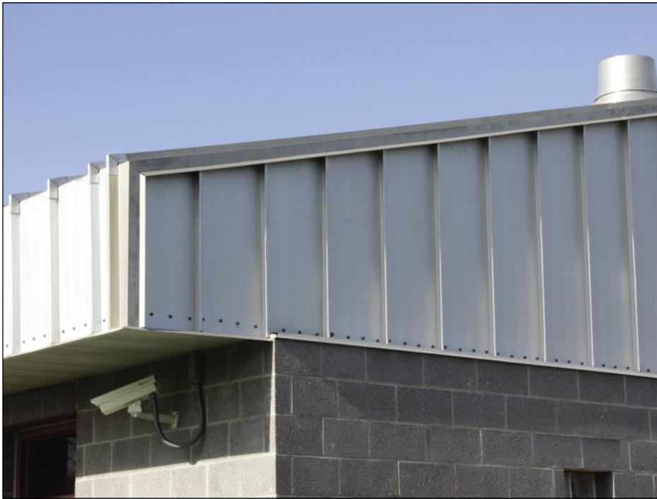
Figure 5-67. Standing seam metal panels with a 16-inch rib spacing were used at the fascia and secured with closely spaced exposed fasteners (Arcadia).
