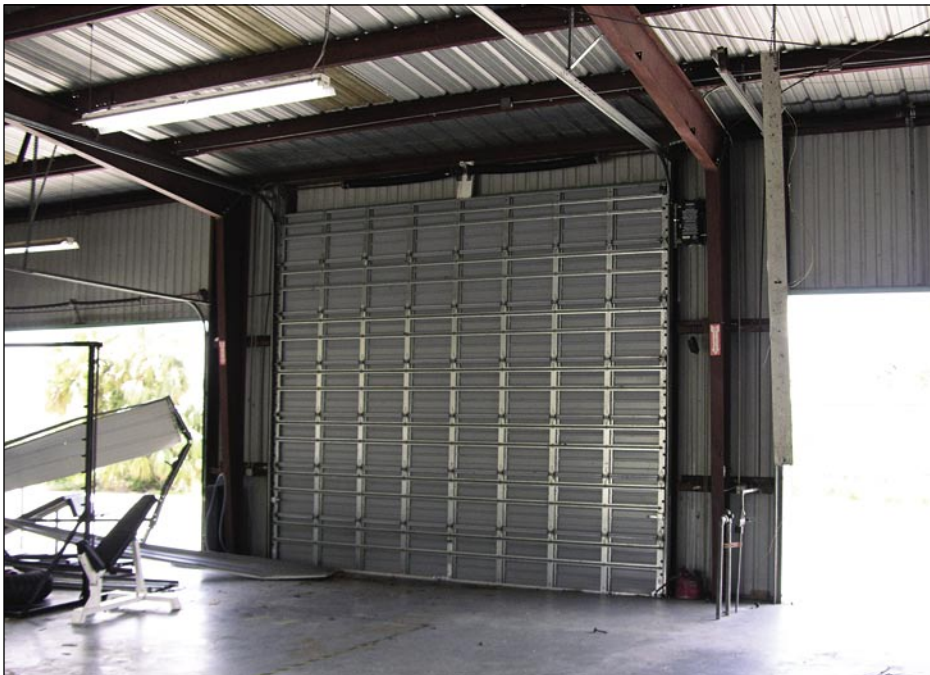
Figure 5-9. Windward side of a fire station; two doors blew inward, but the newer center door remained intact (Punta Gorda).
