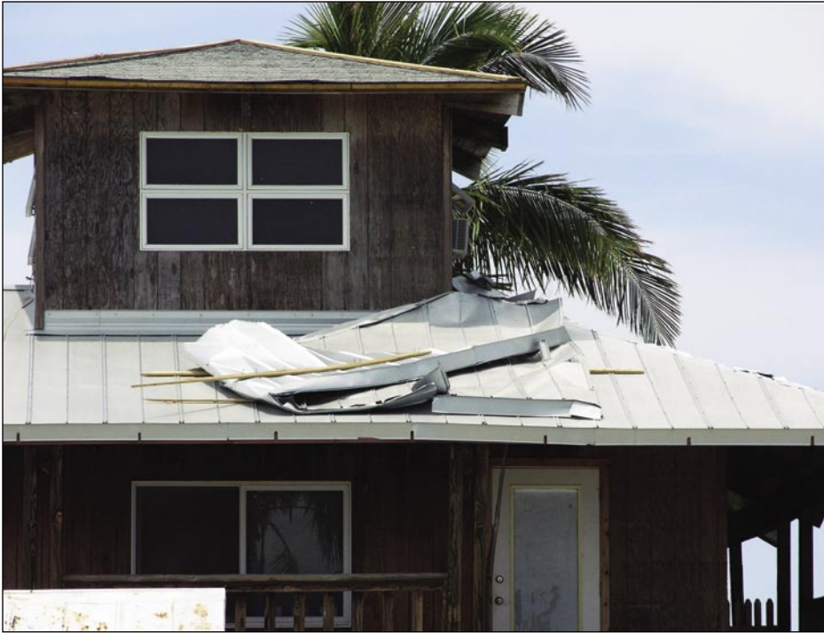
Figure 5-51. These panels blew off the upper roof and landed on the lower roof of this house (Bokeelia, north end of Pine Island).
