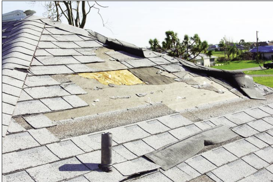
Figure 5-24. Asphalt shingle roof installed on a new residence about 2 months before the hurricane hit; shingles were blown off several areas (Deep Creek).
