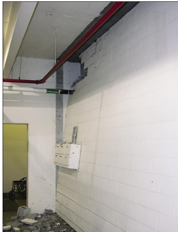
Figure 5-8. After the door shown in Figure 5-7 failed, buildup of internal pressure tilted the wall (Punta Gorda).
