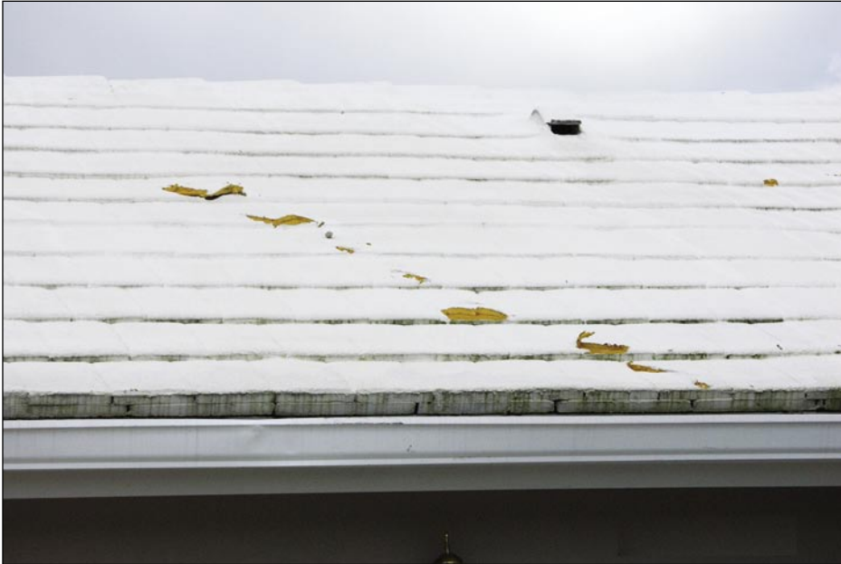
Figure 5-46. This residence had a tile roof that had been covered with SPF. A missile gouged the foam, but no tile debris was blown off (Punta Gorda Isles).
