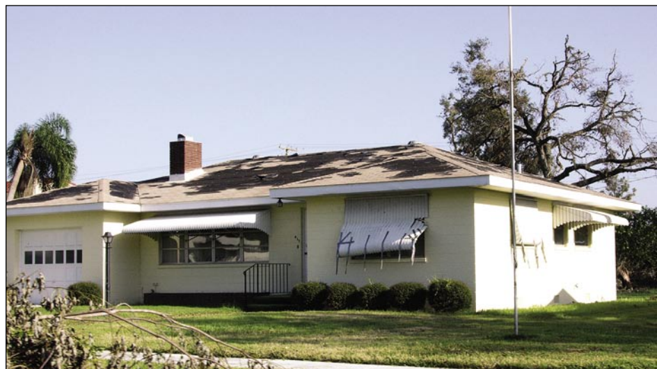
Figure 5-25. Residence with a significant number of asphalt shingles lost. The metal window shutters shown were not designed for windborne debris (Fort Meade).
