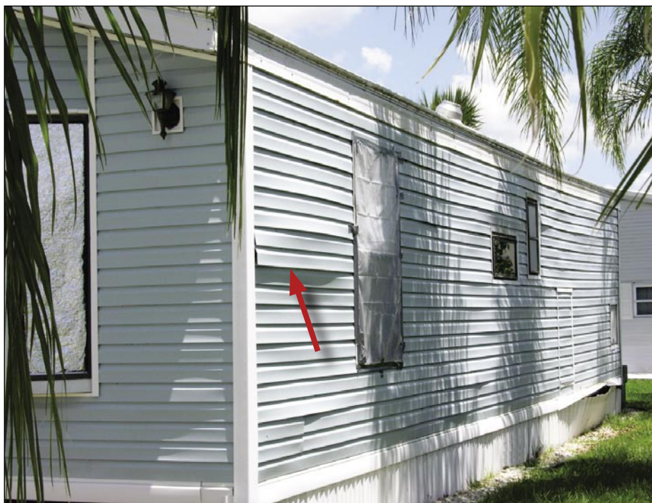
Figure 5-65. The vinyl siding panel with the red arrow is unlatched. The panel above and several others are also unlatched (Zolfo Springs).
