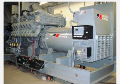
Women’s Hospital Generator
