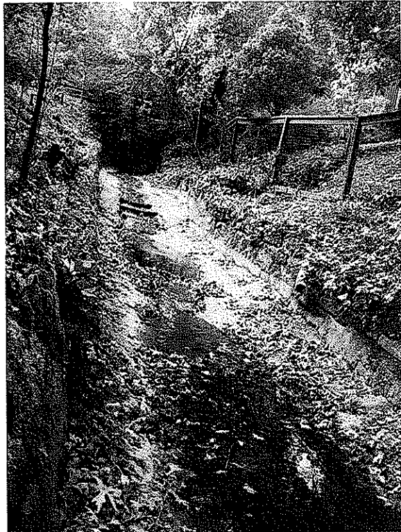
Orinda Stormwater System
