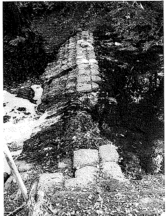
Orinda Stormwater System – stone dropoff
