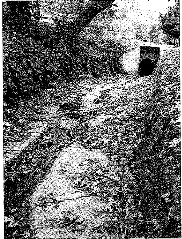
Orinda Stormwater System – pipe drain
