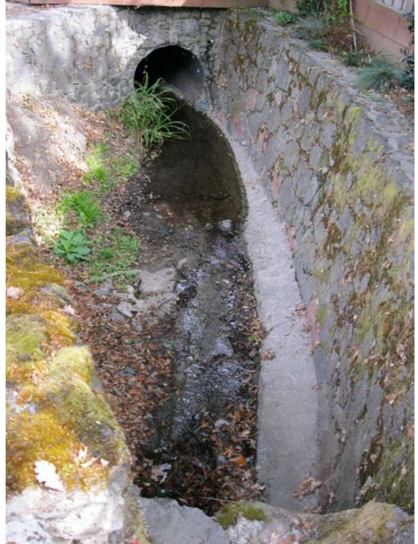
Orinda Stormwater Stytem – Drain
