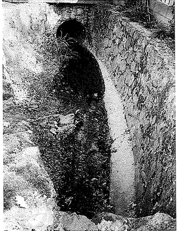
Orinda Stormwater Stytem – Drain
