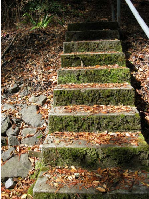
Orinda Stormwater Stytem – Steps
