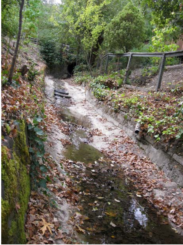
Orinda Stormwater System
