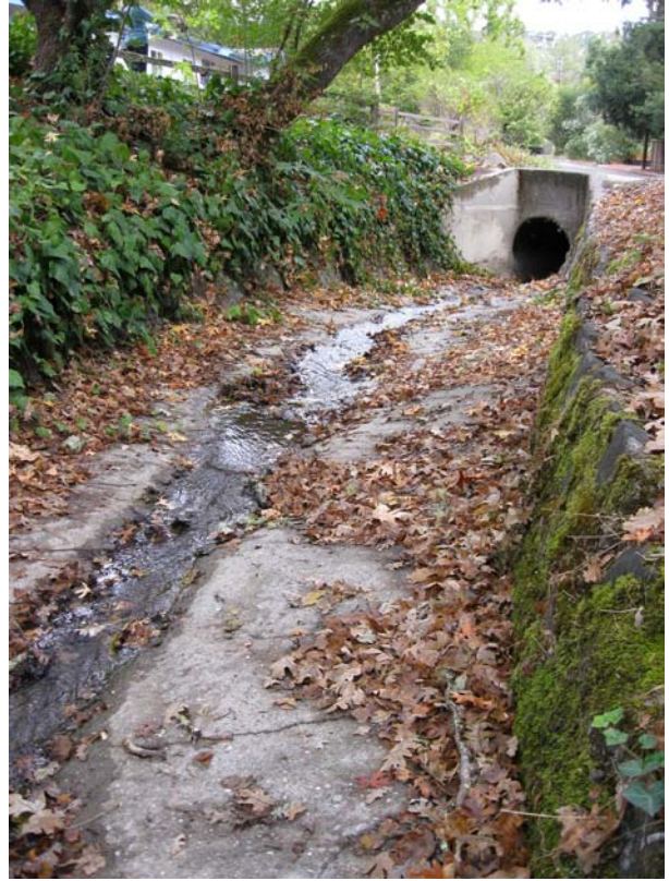
Orinda Stormwater System – pipe drain
