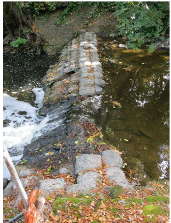
Orinda Stormwater System – stone dropoff
