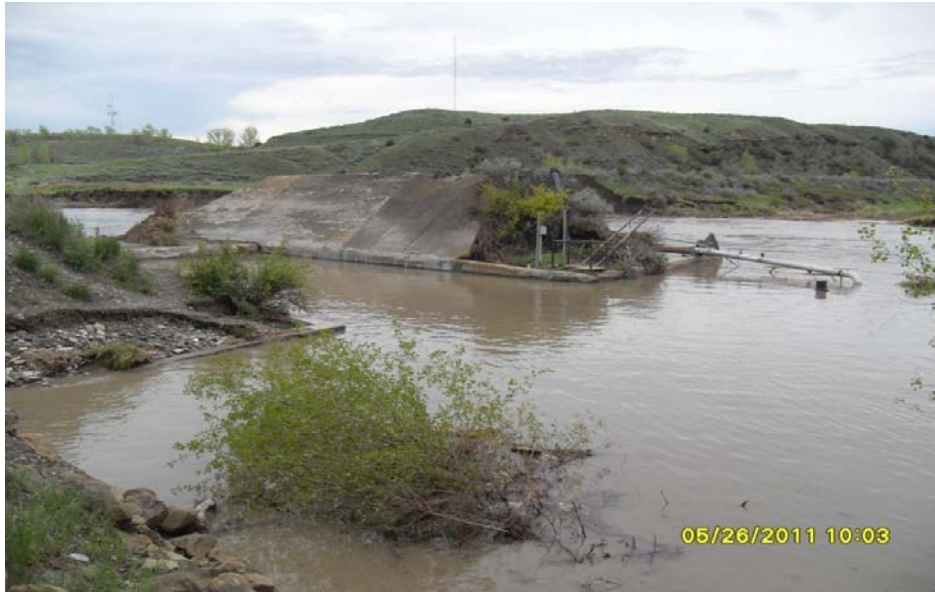
Figure 2: Photo looking southwest at the Pryor Creek Crossing. May 2011, flood waters washed out approximately 200-feet of the canal upstream of the crossing and heavily damaged the existing concrete box culvert.
