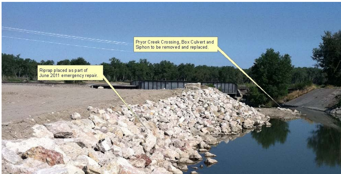
Figure 3: Photo of the emergency fix completed in June 2011 to the Pryor Creek Crossing that allowed for irrigation water to be delivered for the 2011 irrigation season.
