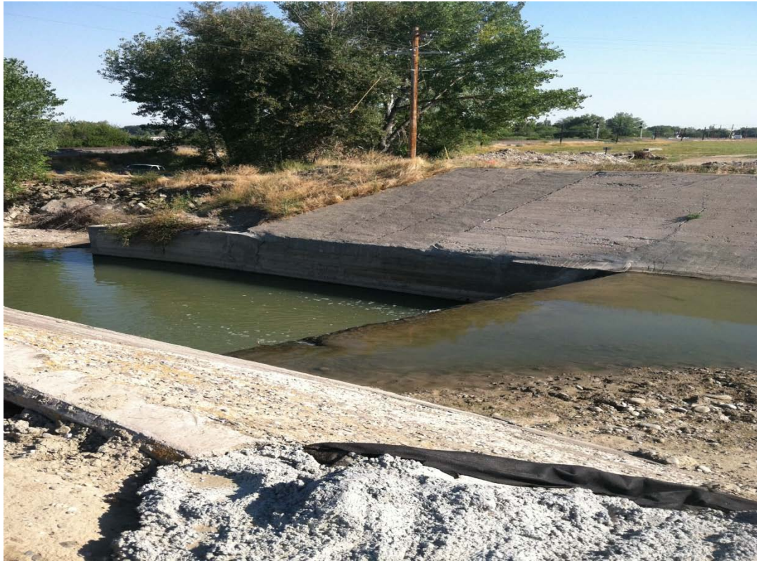
Figure 7: Picture of Pryor Creek Crossing looking towards the Yellowstone River. The drop in the picture does not allow for fish passage into Pryor Creek from the Yellowstone River.
