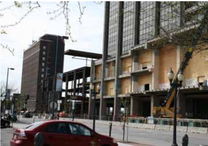
Photograph #11: View from the intersection of 1 st Avenue and the Cedar River Corridor Trail southwest along 1 st Avenue showing construction activities on the Cedar Rapids Convention Center.
