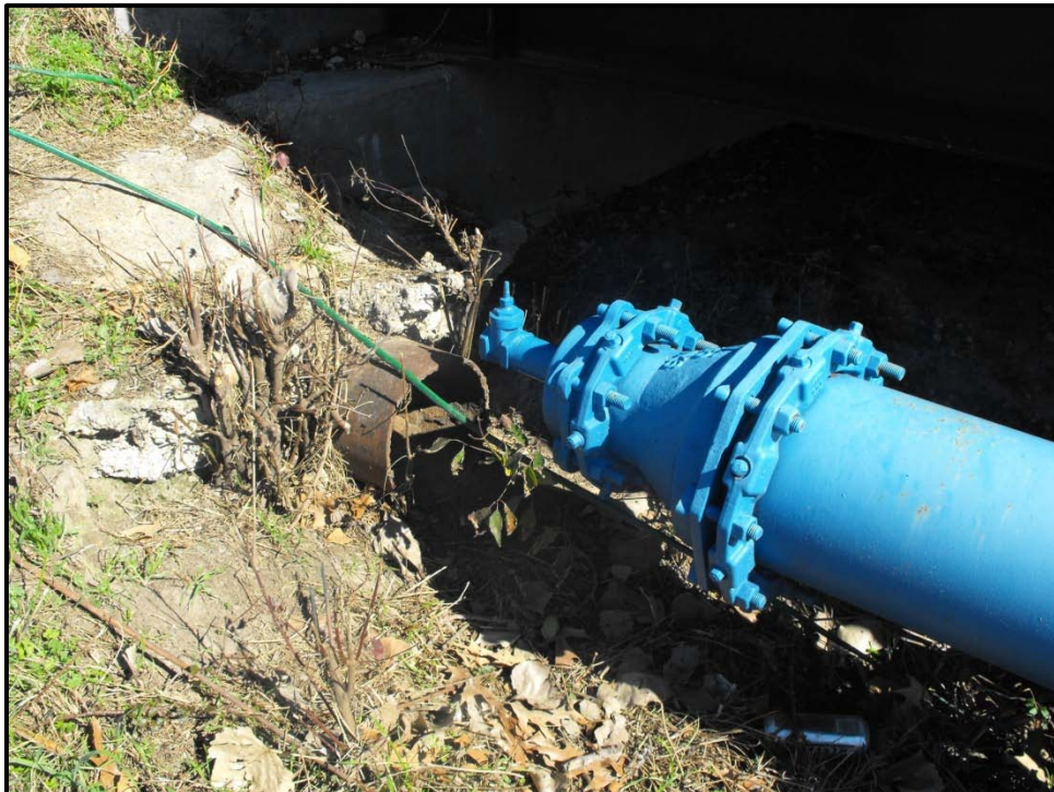
Facing east, this is a view of water main stub that is located under western side of the bridge that connects the parking area and driveway on the project site to the parking area and driveway on the Jersey Meadow Golf Course property. An old relict water line is located underground and enters onto the subject site.
