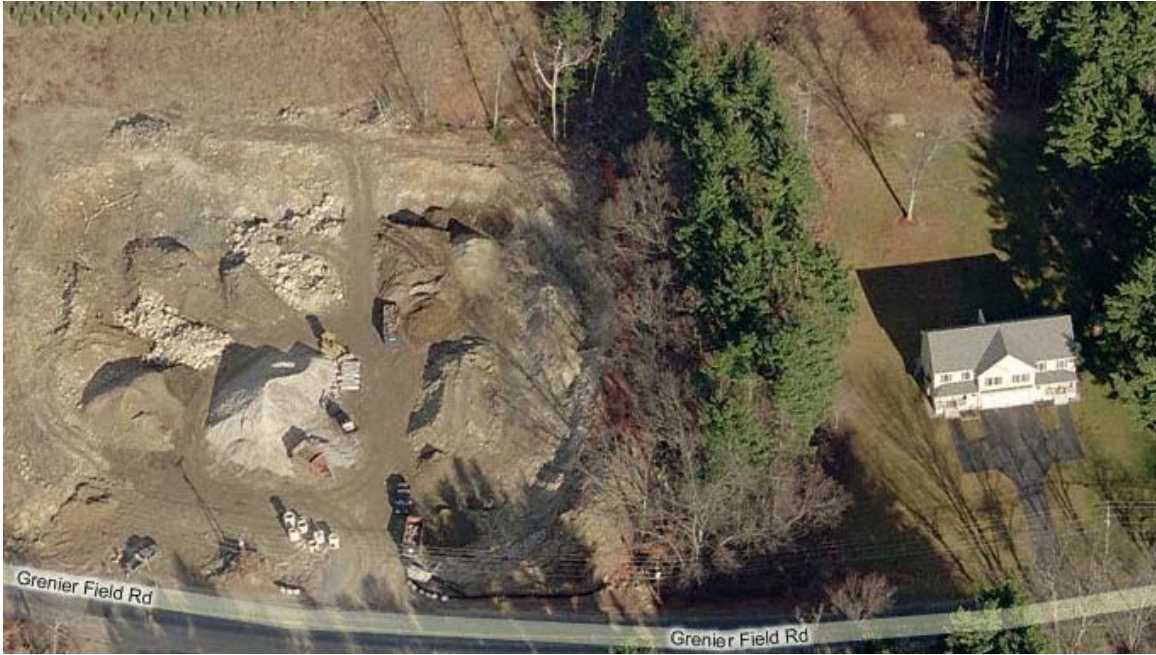
Photo 7. Bird's eye view of the proposed North Fire Station location (excavated area) looking toward the north. Note one residential property adjacent to the right (east).
