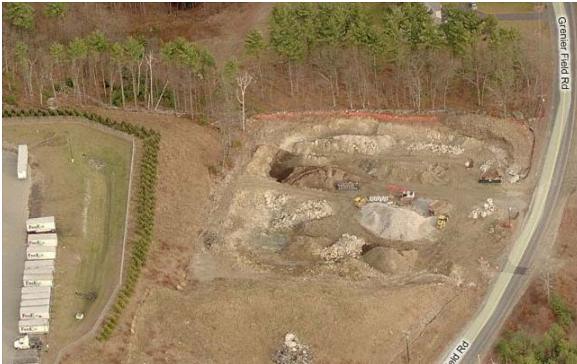
Photo 10. Bird's eye view of the proposed North Fire Station location (excavated area) looking toward the east. Note the FedEx facility to the left (north).
