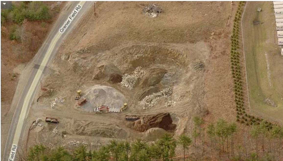
Photo 8. Bird's eye view of the proposed North Fire Station location (excavated area) looking toward the west. Note FedEx facility to the right of the photo (north and up hill of the proposed location). A race track is off the photo to the upper left (southwest).
