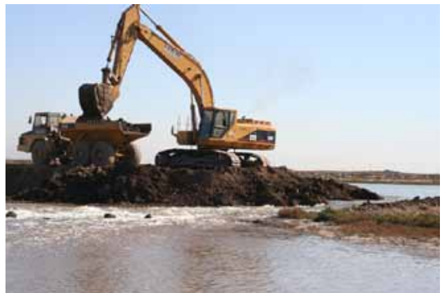
Removing or breaching manmade levees can be an effective way to restore natural processes.
