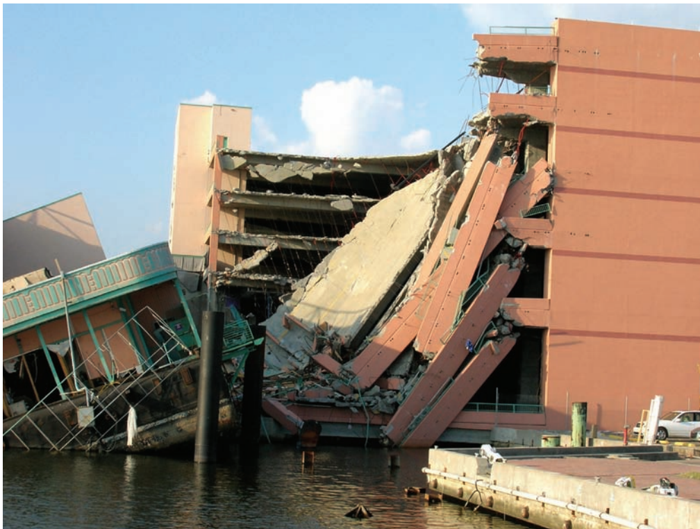
Figure 2-25 Progressive collapse of upper floors of a parking garage due to damage in lower level columns from impact of an adjacent barge-mounted casino (Hurricane Katrina, 2005).
