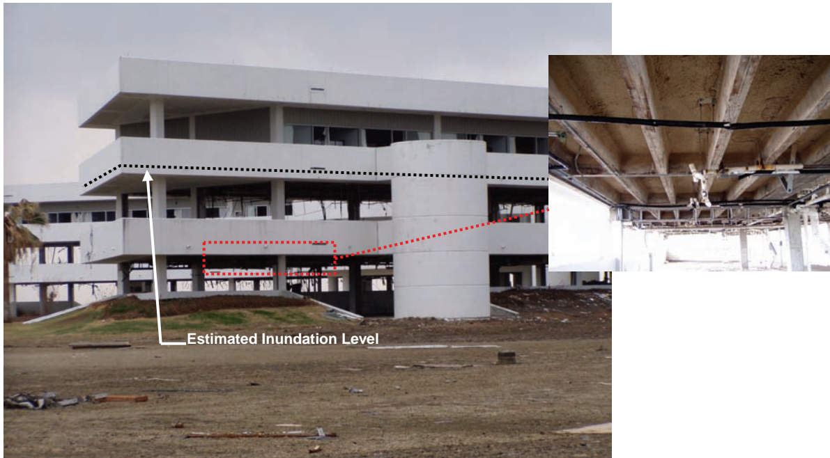
Figure 2-23 Pass Christian office building with cast-in-place concrete pan joist floor system that suffered non-structural damage at first two floors but no structural damage (Hurricane Katrina, 2005).
