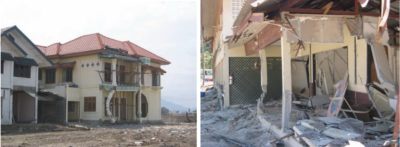
Figure 2-17 Damage to non-engineered concrete columns due to debris impact (Photos courtesy of M. Saatcioglu, A. Ghojarah and I. Nistor, CAEE, 2005).
