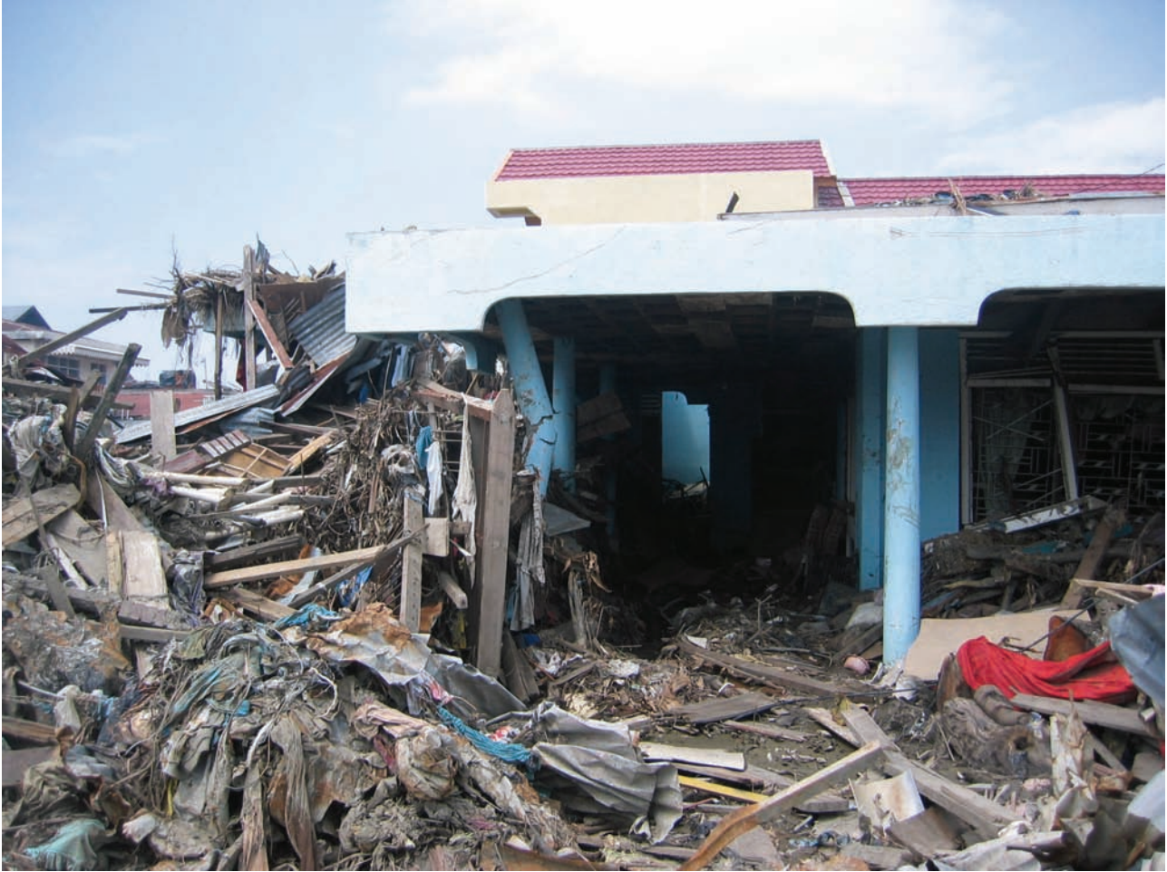
Figure 2-18 Damage to corner column due to debris damming (Photo courtesy of M. Saatcioglu, A. Ghojarah and I. Nistor, CAEE, 2005).
