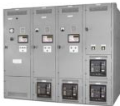
Figure 4: Service entrance with transfer switch (floor-mounted).
