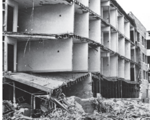
■ Figure 14. Heavily damaged Hotel Californian, 1925 Santa Barbara, California earthquake. —NISEE, U.C. Berkeley
