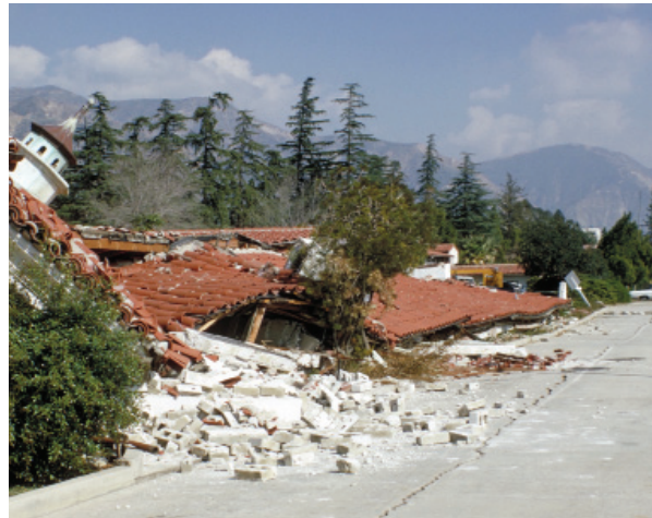
■ Figure 9. Complete collapse of an unreinforced concrete block building, 1971 San Fernando earthquake. —Karl Steinbrugge, NISEE, U.C. Berkeley
