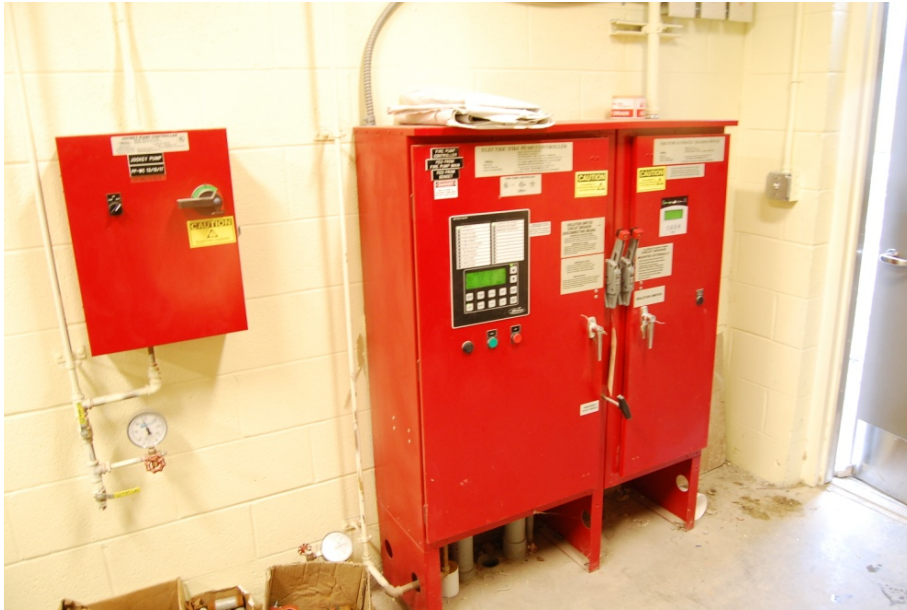
Figure 4-2 Typical fire pump controller.
