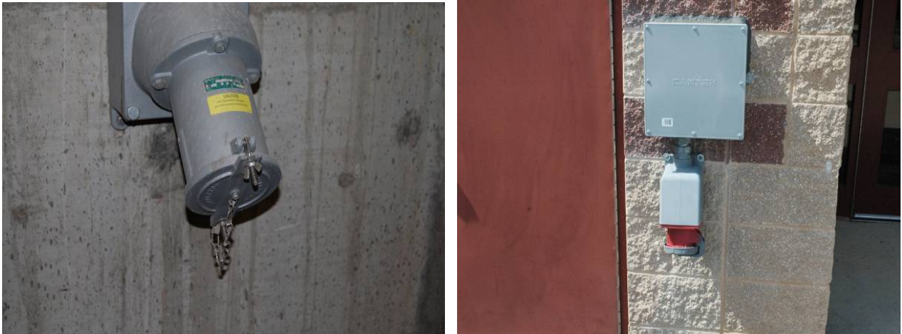
Figure 5-8 Building-mounted twist-lock plugs for connecting temporary generator cables.
