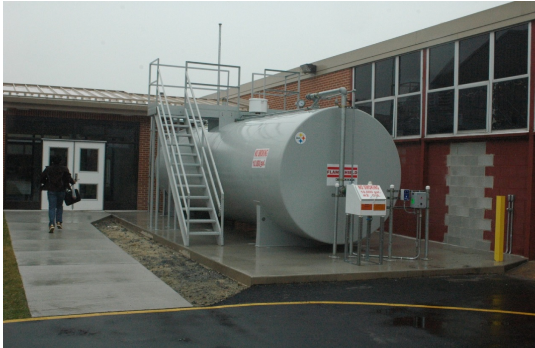
Figure 5-5 Fuel oil storage tank used for heating equipment that can supply an emergency diesel generator.
