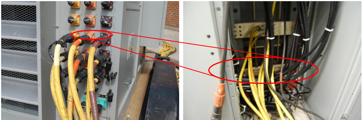
Figure 5-9 Electrical connection point for temporary generator using slip-fit connectors (left), and cables at building connection (right).
