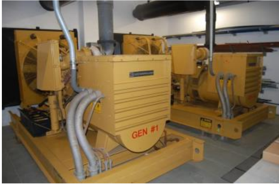
Figure 6-4 Interior generator protected from the effects of wind and wind-borne debris.
