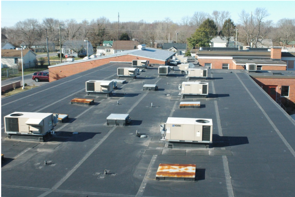
Figure 4-4 Roof-top mounted DX HVAC units.
