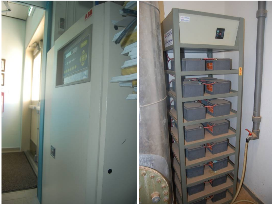
Figure 5-1 UPS system containing an inverter (left) and battery rack (right) located in a low seismic area.
