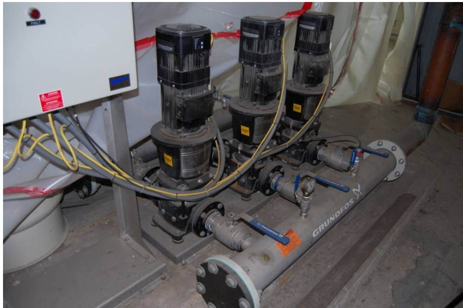
Figure 4-8 Domestic water booster pumps.
