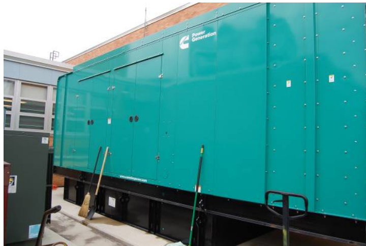
Figure 5-4 Exterior emergency generator placed in a sound-attenuating enclosure.
