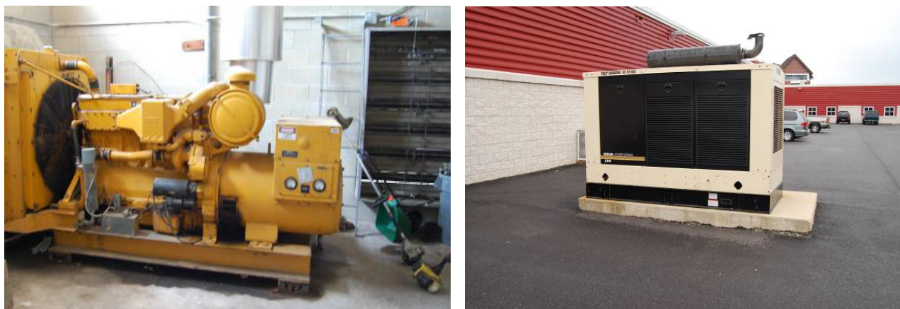
Figure 5-3 Emergency generator installed on the interior (left) and exterior (right).
