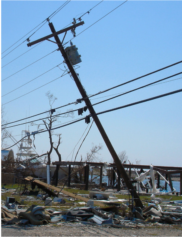
Figure 2-10 Overhead line damaged when flooding saturated soils and reduced strength of guy anchors (Deleon, 2014). Hydrodynamic loads from moving floodwaters may have contributed to failure.
