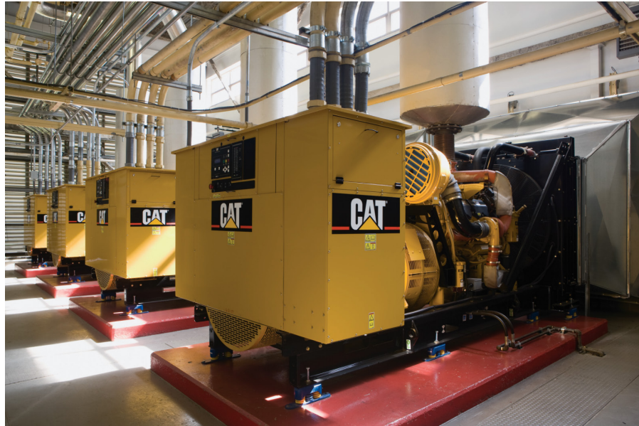
Figure 6-5 Emergency generator supported by seismically-rated vibration isolators.
