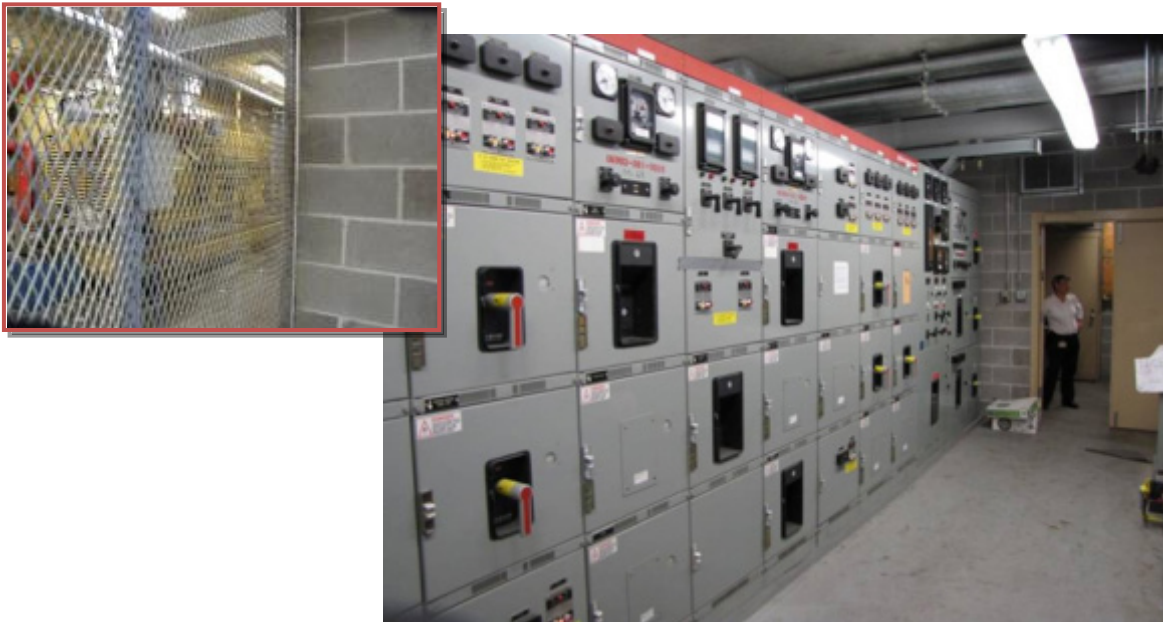
Figure 6-3 Switchgear, normal, and emergency power feeds, and associated equipment elevated to the same level as the emergency generator at UTMB, Galveston, Texas in 2010.
