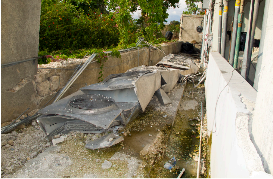
Figure 2-16 Falling debris from security wall and parapet damaged cooling equipment for servers resulting in the data center going off line in the 2011 Haiti earthquake.
