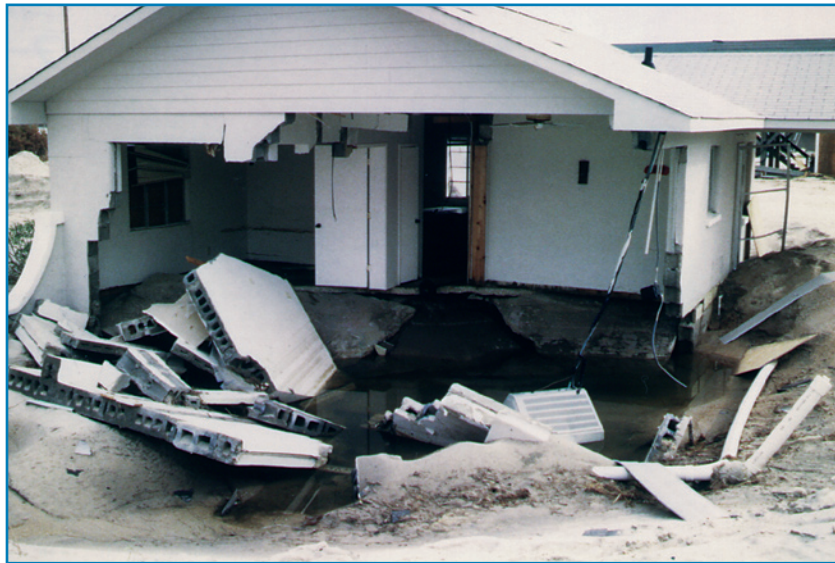
Figure 2-16: Scour around the foundation of this building contributed to significant damage.
