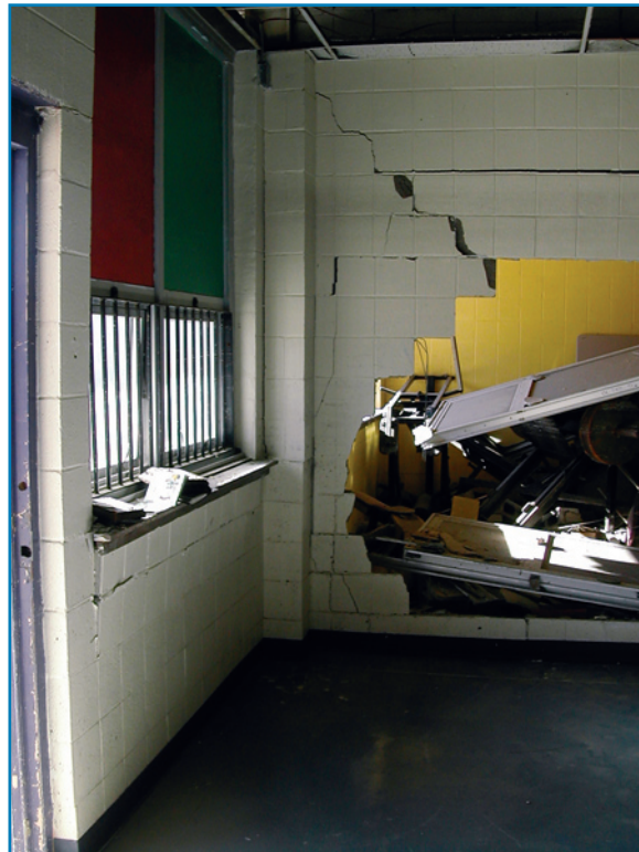
Figure 2-14: Interior unreinforced masonry walls of the Port Sulphur High School in Louisiana were damaged by hydrostatic loads associated with Hurricane Katrina's storm surge (2005).
