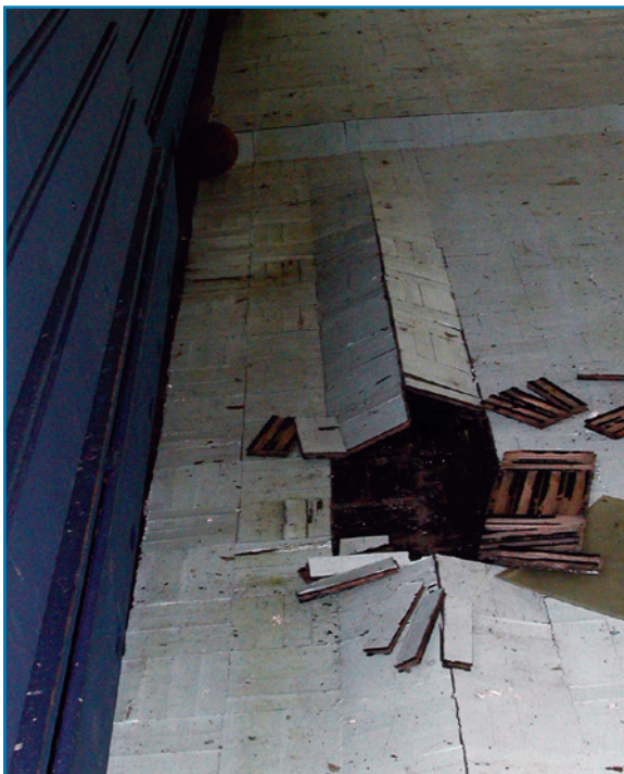
Figure 2-17: This parquet wood gymnasium floor was damaged by dimensional changes due to saturation. Hurricane Katrina (2005)
