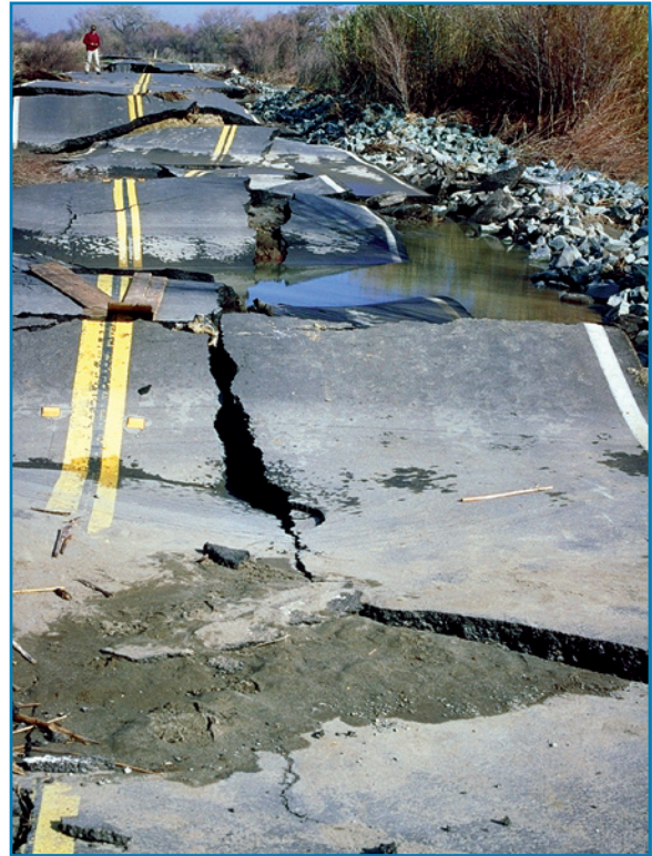
Figure 2-13: Flooding caused the failure of this road bed. SOURCE: U.S. ARMY CORPS OF ENGINEERS
