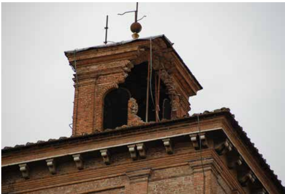
Fig.3 Damage to one of the turrets at the Castle of Ferrara during the earthquake in 2012, Italy.
