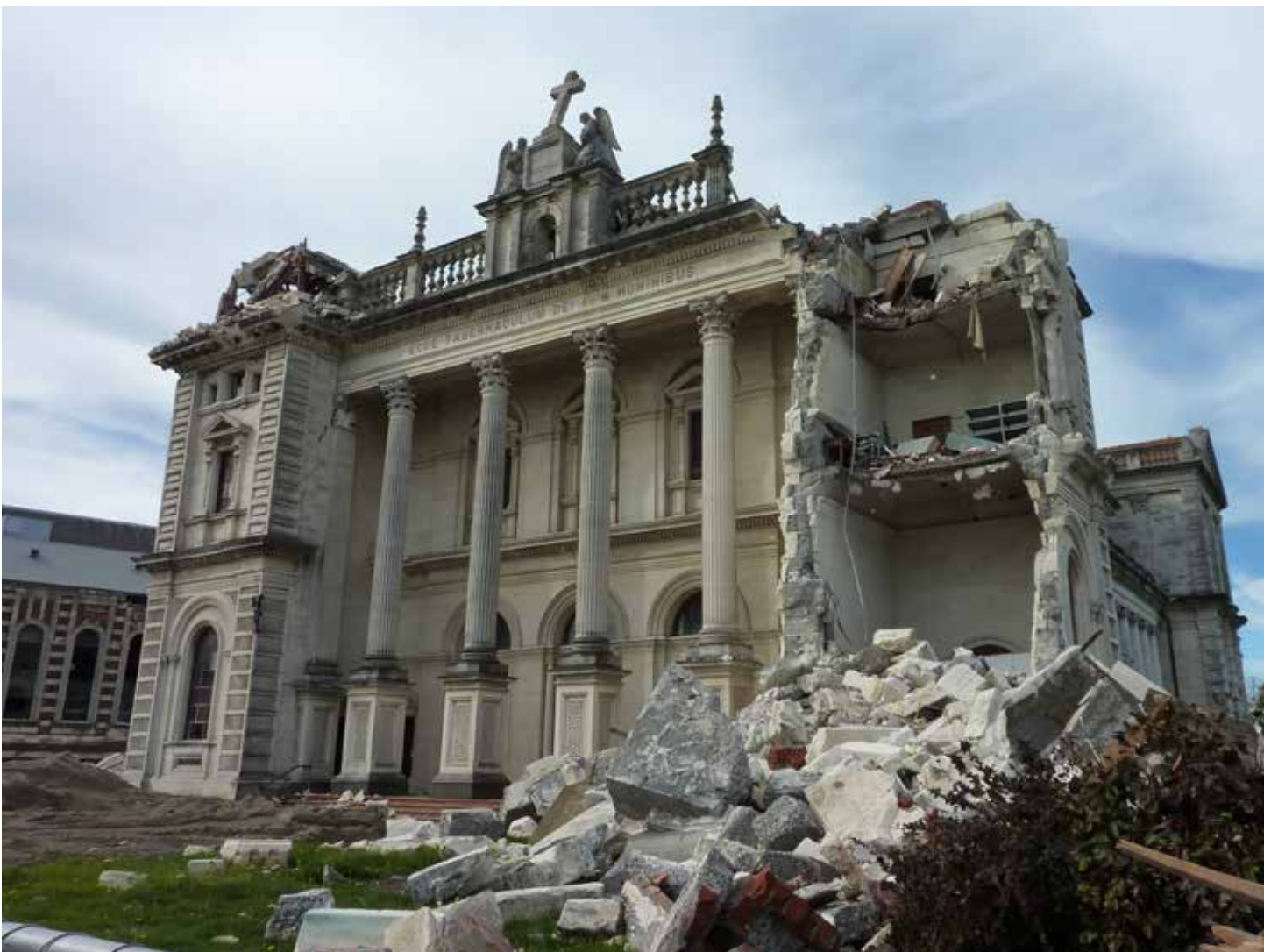
Fig.12 Earthquake damage to the Catholic Basilica in Christchurch, New Zealand. SOURCE: Bryan Lintott , 2011
