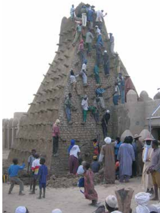
Fig.9 Repair work at Timbuktu, Mali. The World Heritage site has suffered significant damage during recent civil unrest SOURCE: Francesco Bandarin, UNESCO, 2005. http://whc.unesco.org/en/list/119/
