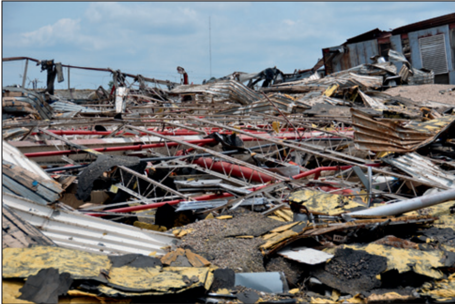
Figure 7-57: View of a portion of the collapsed one-story area (Tuscaloosa, AL)
