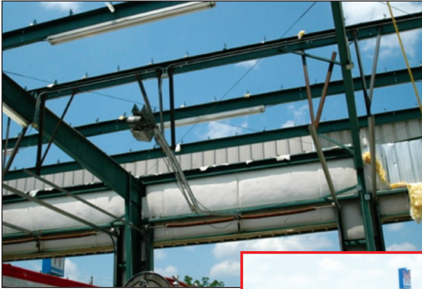
Figure 7-32: The metal roof panels blew off the apparatus bay of the fire department. The panels unlatched from the clips, shown at another angle in the inset (Fultondale, AL).
