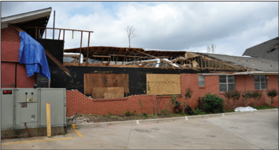
Figure 7-10: Roof structure and brick veneer were blown off the nursing home (Tuscaloosa, AL)
