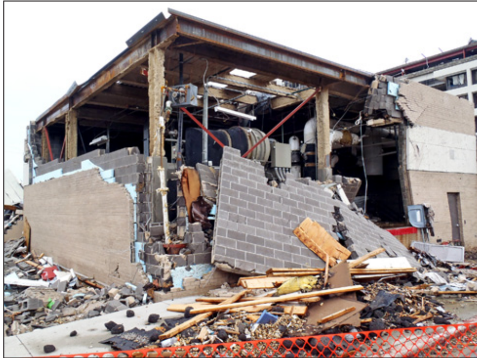
Figure 7-27: Exterior wall collapse (EIFS over unreinforced CMU) at an equipment room (Joplin, MO)
