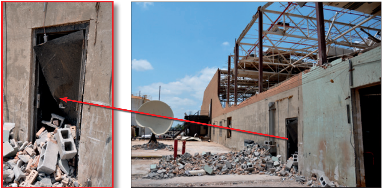
Figure 7-60: Part of the southern portion of the building. The inset shows a metal door that buckled inward (Tuscaloosa, AL).
