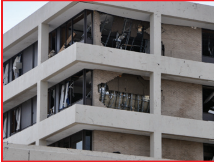
Figure 7-24: Collapse of a portion of the exterior metal composite foam wall panels at the East Tower addition (red arrows). The inset shows collapsed brick veneer at the Original Tower. Most of the glazing shown in this photograph was broken (Joplin, MO).
