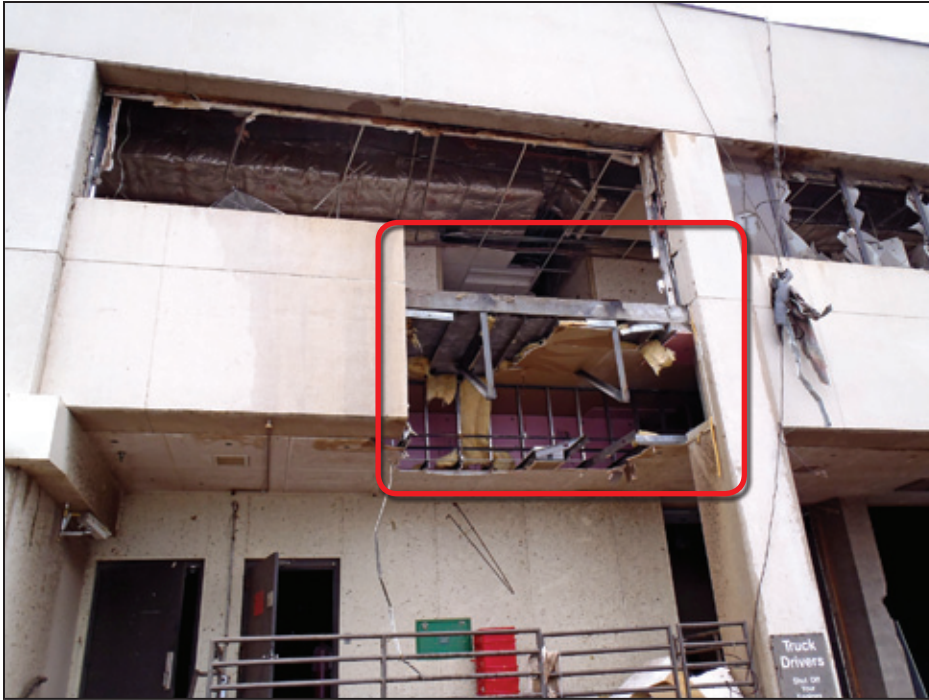
Figure 7-25: View of a missing precast concrete wall panel (red box) at the loading dock (Joplin, MO)
