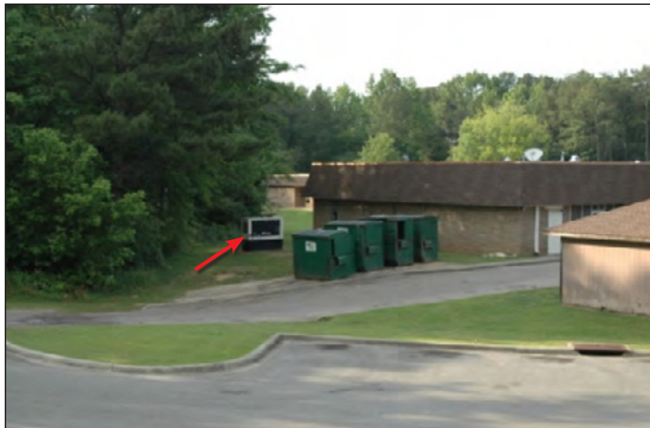
Figure 7-7: The emergency generator (red arrow) is located near many trees that could easily have damaged the generator and taken it out of service (Birmingham, AL)
