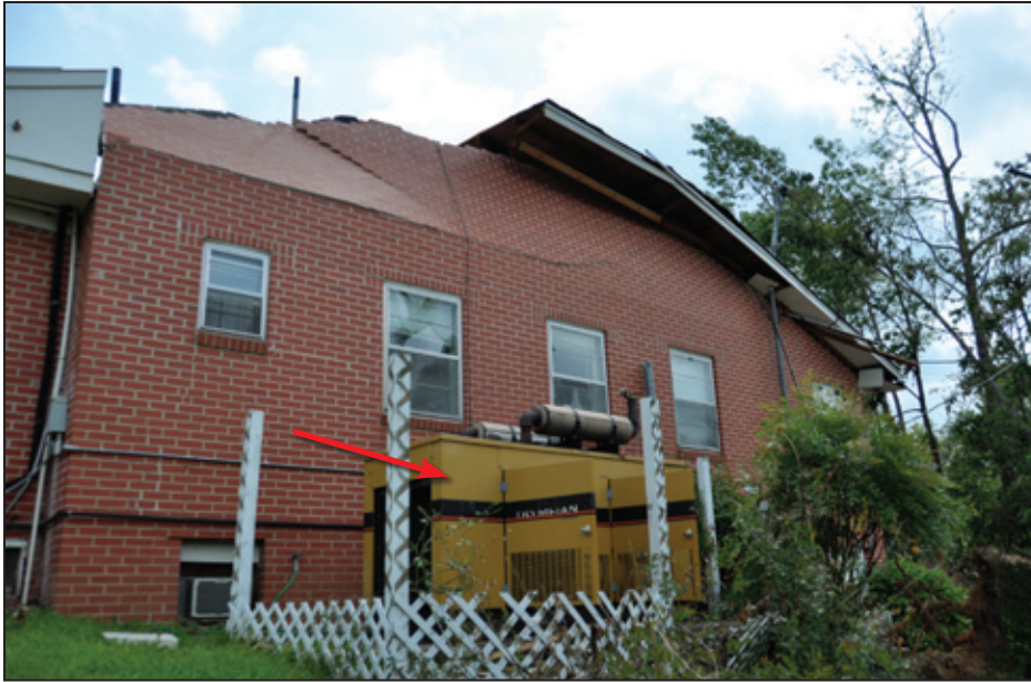
Figure 7-15: Generator at the southwest side of the facility (red arrow). Note the roof structure blow-off and wall collapse (Tuscaloosa, AL).
