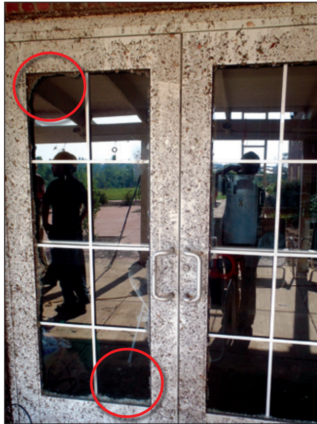
Figure 4-6: Double-glazed window with outer pane sacrificed (remaining fragments are circled in red), leaving the inner glazing intact (Mercy Village, Joplin, MO); refer also to Section 4.2.3 for a case study of Mercy Village
