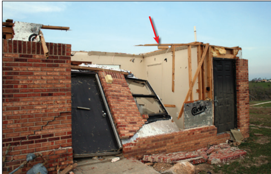
Figure 4-23: Example of DOD 6 showing failure of roof framing that resulted in loss of lateral support for the top of this wall (red arrow) (Phil Campbell, AL) [MAT EF Rating = 2]
