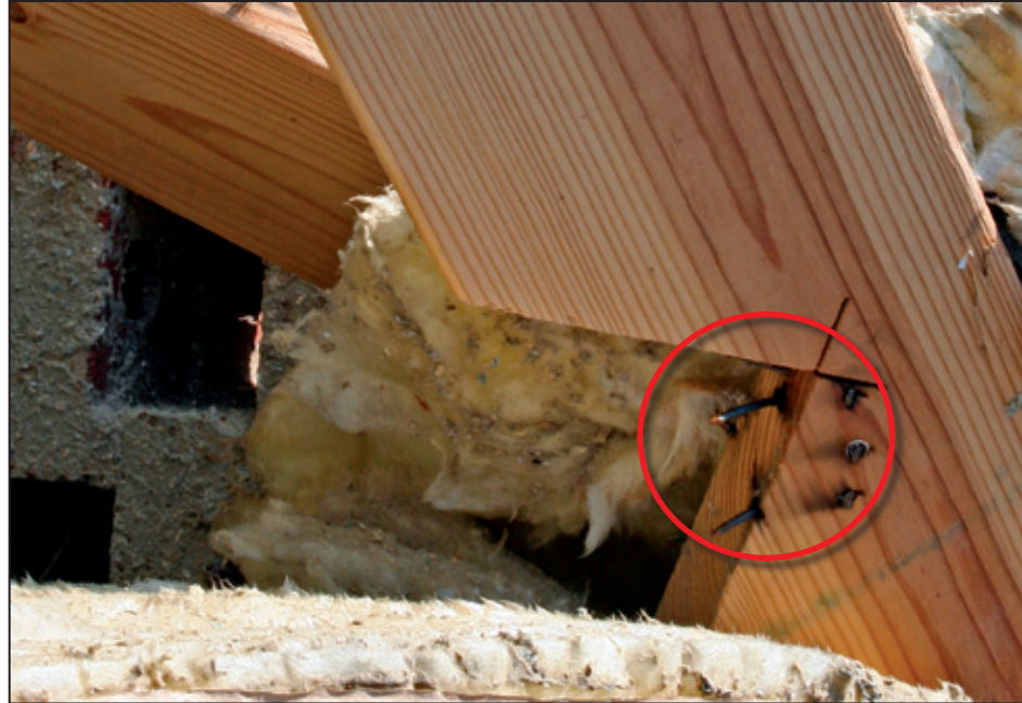
Figure 4-20: Over-notched rafter found on ground with two toe nails withdrawn from plate (red circle) (Harvest, AL) [MAT EF Rating = 1]
