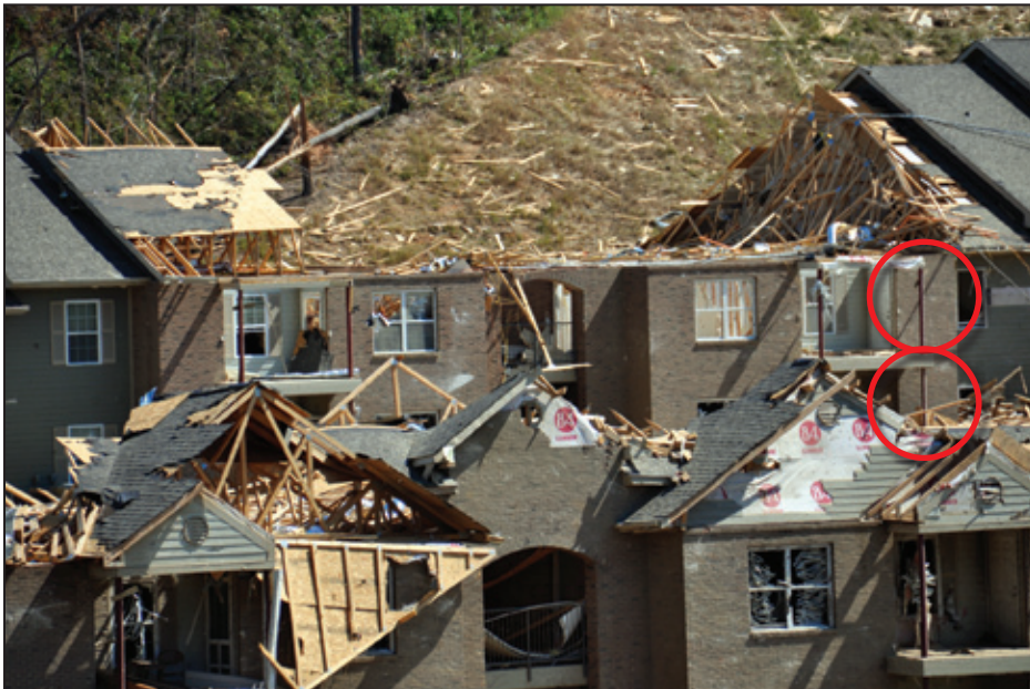
Figure 4-35: Example of DODs 3 and 4 showing two-story Chastain Manor Apartments with varying roof damage. Note upper and lower steel pipe porch columns (red circles).
