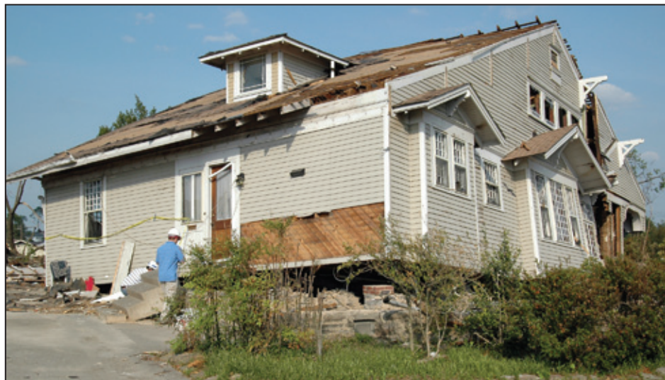
Figure 4-17: Example of DOD 5 showing residential building shifted off masonry piers (Cullman, AL) [MAT EF Rating = 2]
