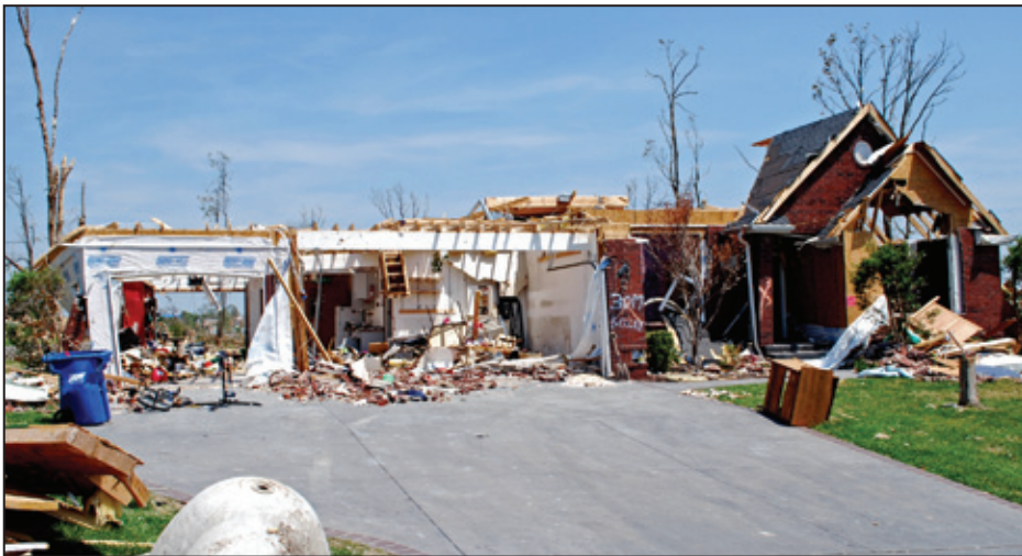
Figure 4-9: Example of damage including loss of large sections of roof (DOD 6) apparently initiated from garage door failure (DOD 4) (Joplin, MO) [MAT EF Rating = 2]
