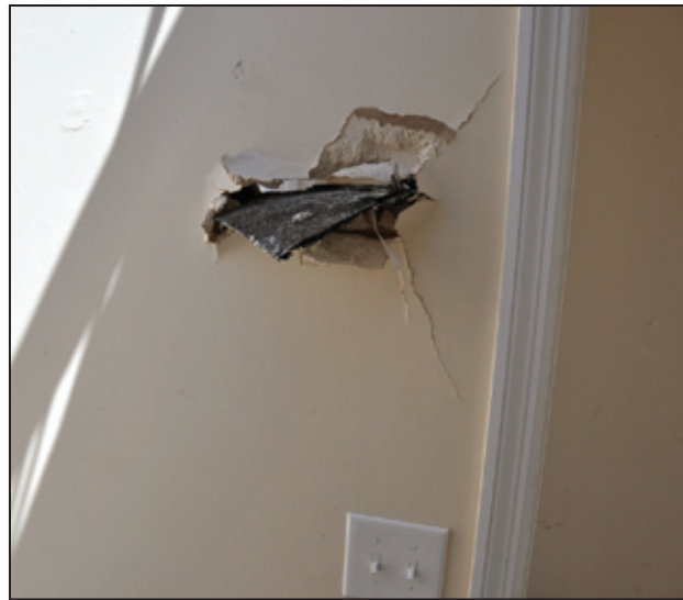
Figure 4-1: Wind-borne asphalt shingle penetrated the gypsum board on both sides of this interior wall at Chastain Manor Apartment Complex (Tuscaloosa, AL)
