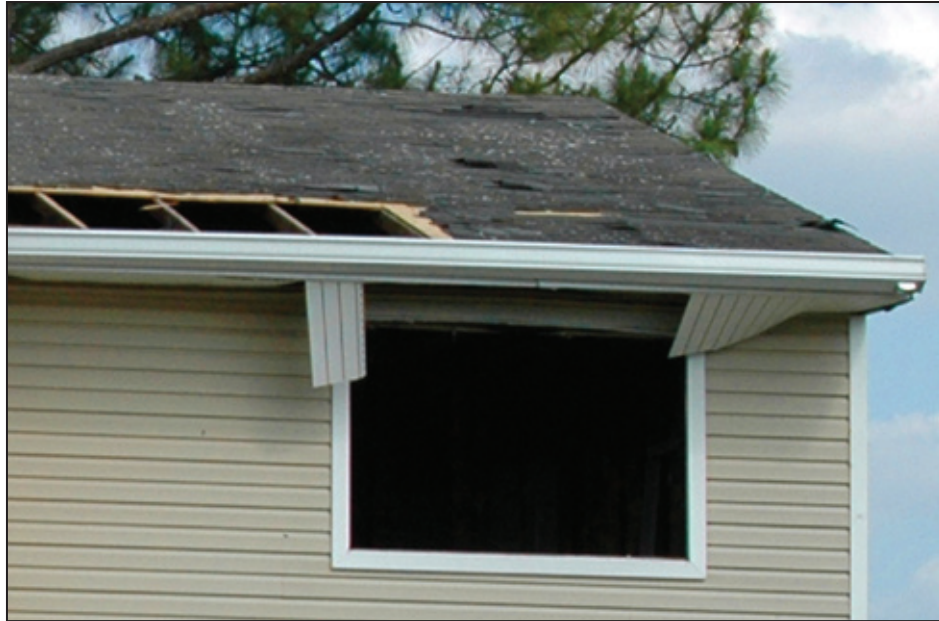
Figure 4-13: Example of DOD 4 showing where roof decking lifted and blew off above damaged soffit in roof Zone 2 (see Figure 4-12) (Birmingham, AL) [MAT EF Rating = 2] 4
