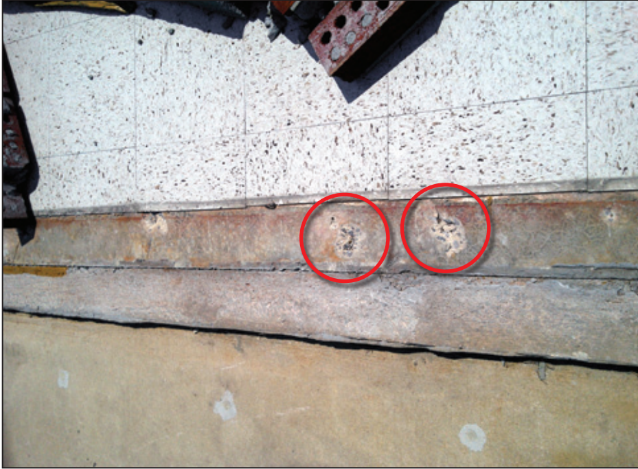
Figure 4-30: Wall-to-foundation failure where bottom plate and concrete nails were pulled out by high winds. Shallowly embedded concrete nails pulled small cones of concrete up with bottom plate (red circles) (Hackleburg, AL). [MAT EF Rating = 3]
