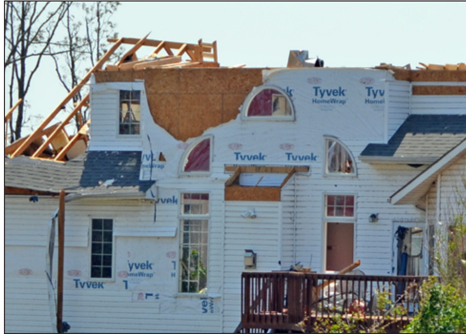
Figure 4-4: Example of DOD 2 (loss of siding) through DOD 6 (large sections of roof structure removed) (Joplin, MO) [MAT EF Rating = 2]
