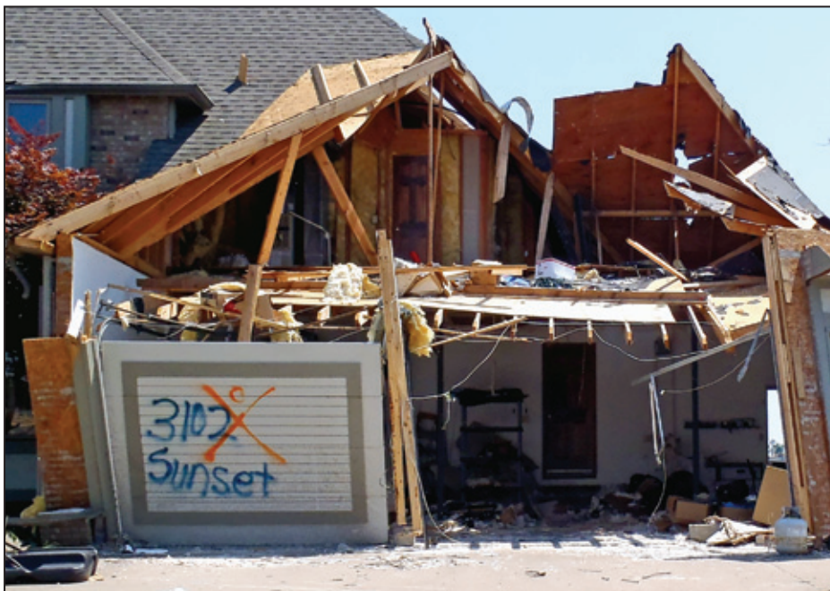
Figure 4-25: Example of DOD 6 where most walls remained standing, but under-braced garage entry wall failed (Joplin, MO) [MAT EF Rating = 2]
