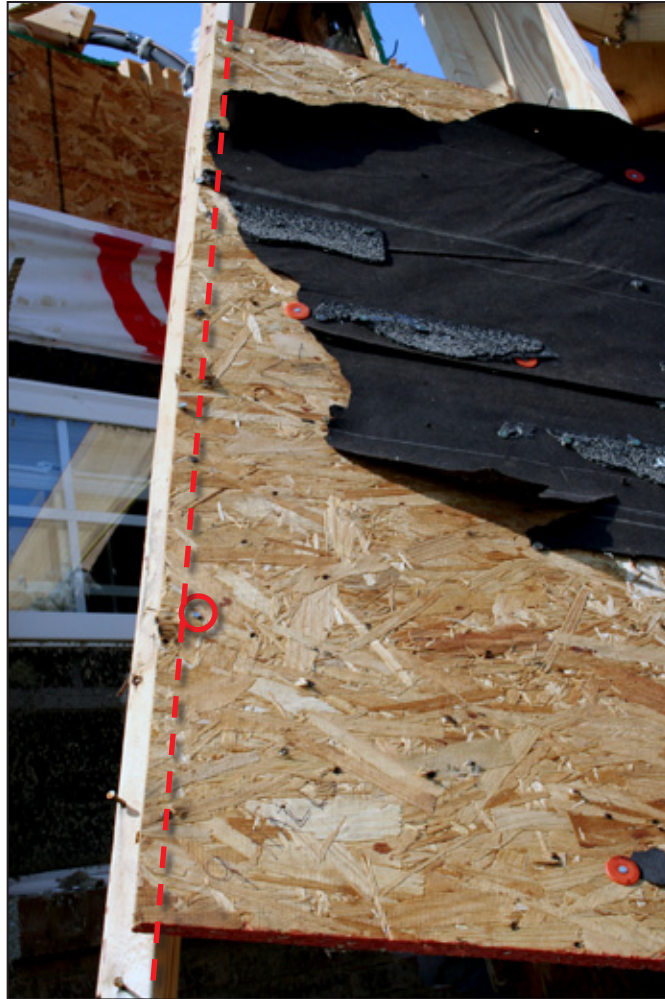
Figure 4-15: Red circled roof deck nail not connected to rafter (edge shown with red dashed line) (Harvest, AL)
