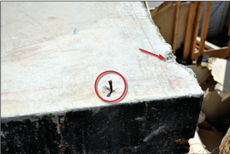
Figure 4-31: Wall-to-foundation connection failure. Note slab failure along right edge where the bottom plate separated and the nail was removed (red arrow). A remaining cut nail is indicated by the red circle. (Tuscaloosa, AL). [MAT EF Rating = 4]
