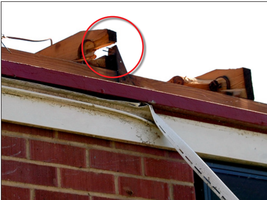
Figure 4-22: Example of DOD 6 showing insufficient connection of single roof-to-wall connector on remaining chord of roof truss at left (red circle) and none on truss at right (Tuscaloosa, AL) [MAT EF Rating = 2]
