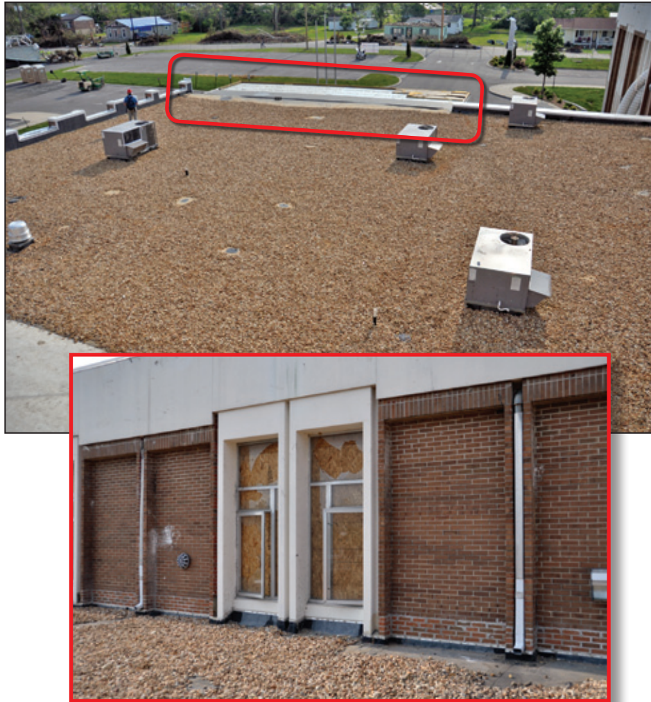
Figure 6-30: View of the aggregate ballasted roof. The fully adhered roof membrane blew away; inset below (red box) shows broken windows (Ringgold, GA).
