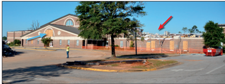
Figure 6-11: University Place Elementary School after the tornado. The red arrow shows the collapsed second story of one of the classroom wings. Several broken windows were boarded up at the time of the MAT visit (blue arrow) (Tuscaloosa, AL).
