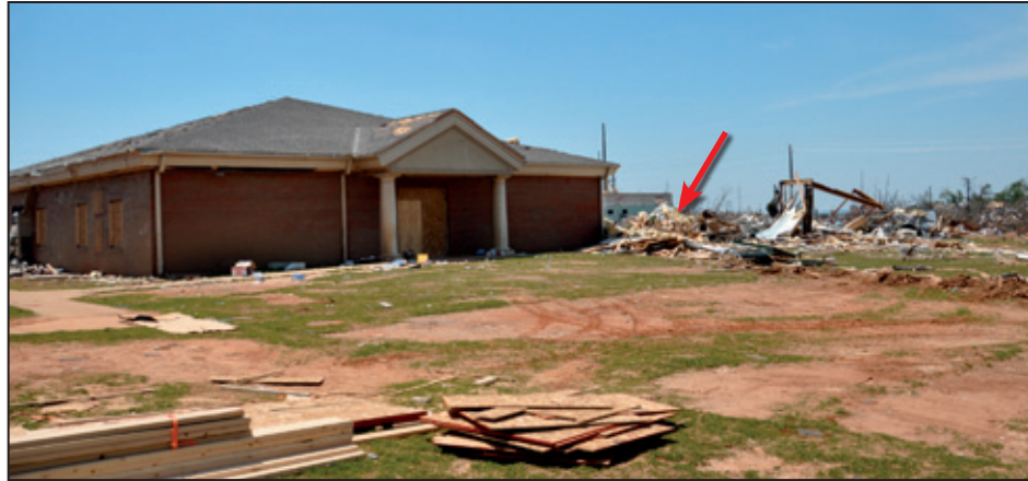
Figure 6-7: Center classroom wing remains standing while the wing to the right (red arrow) collapsed (Tuscaloosa, AL)
