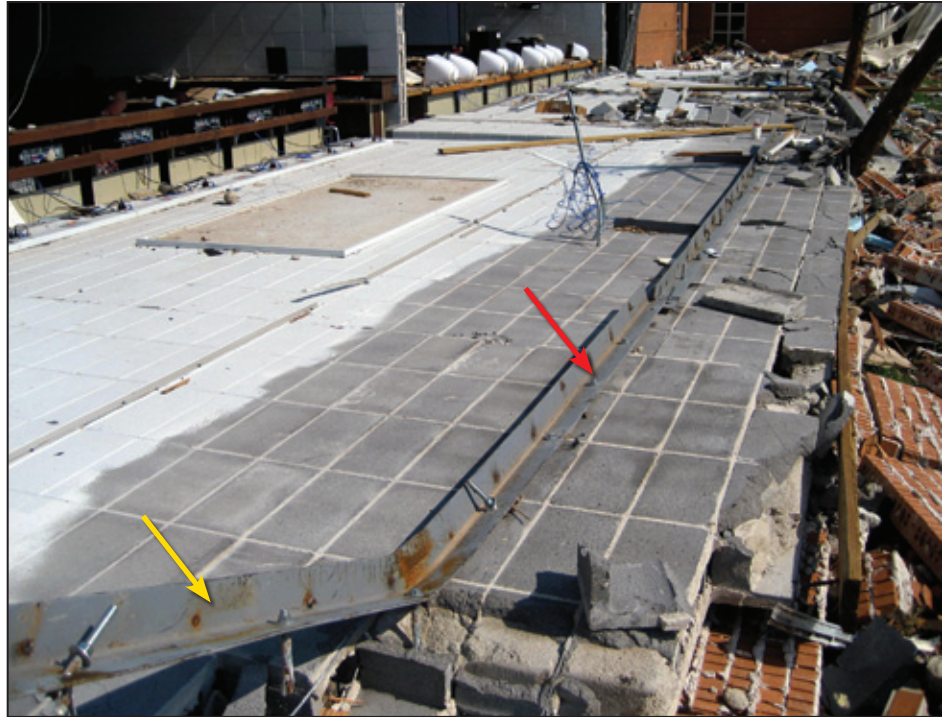
Figure 6-53: Collapsed brick veneer/ reinforced CMU. The red arrow indicates where the ledger angle is still connected to the CMU. The yellow arrow indicates where the angle's expansion bolts pulled out of the CMU (Joplin, MO).
