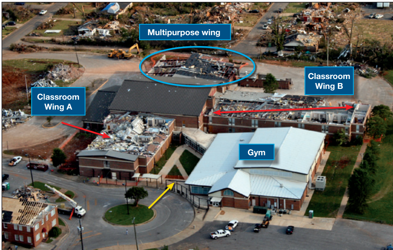
Figure 6-14: View looking south showing damage of the classroom wings (red arrows) and multipurpose wing (blue oval). The yellow arrow indicates damaged walkway canopy (Tuscaloosa, AL).
