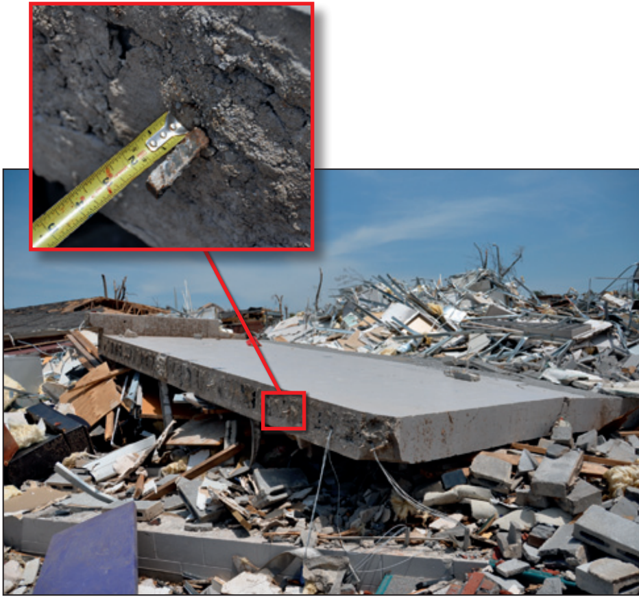
Figure 6-6: Interior reinforced CMU wall in the central core area where rebar had deficient splice lap. Inset shows a close-up of the deficient splice lap (Tuscaloosa, AL).
