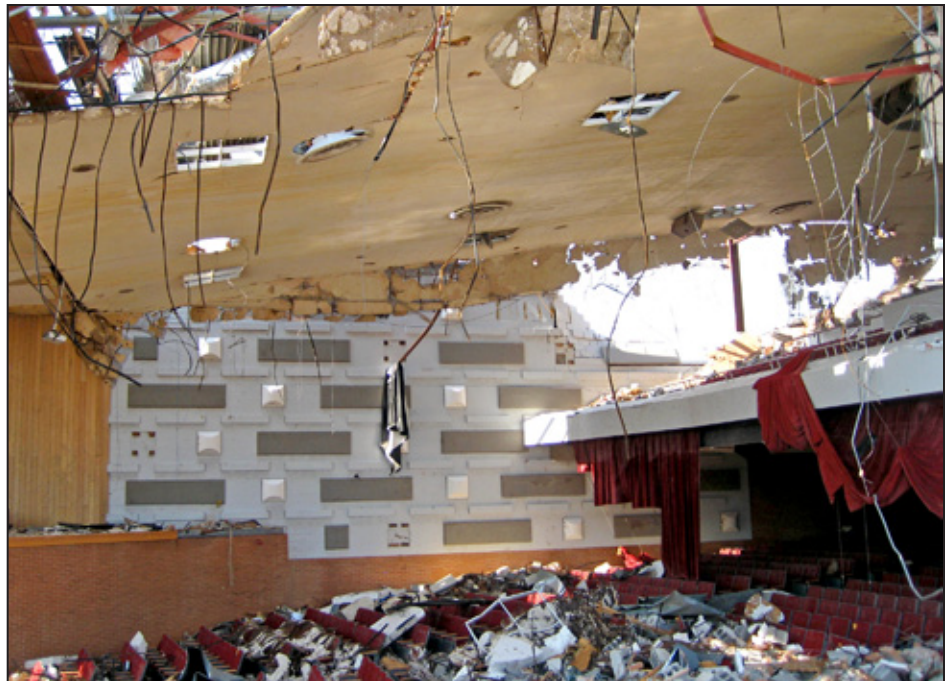
Figure 6-57: South wall of the auditorium, showing collapse of the masonry infill wall (Joplin, MO)
