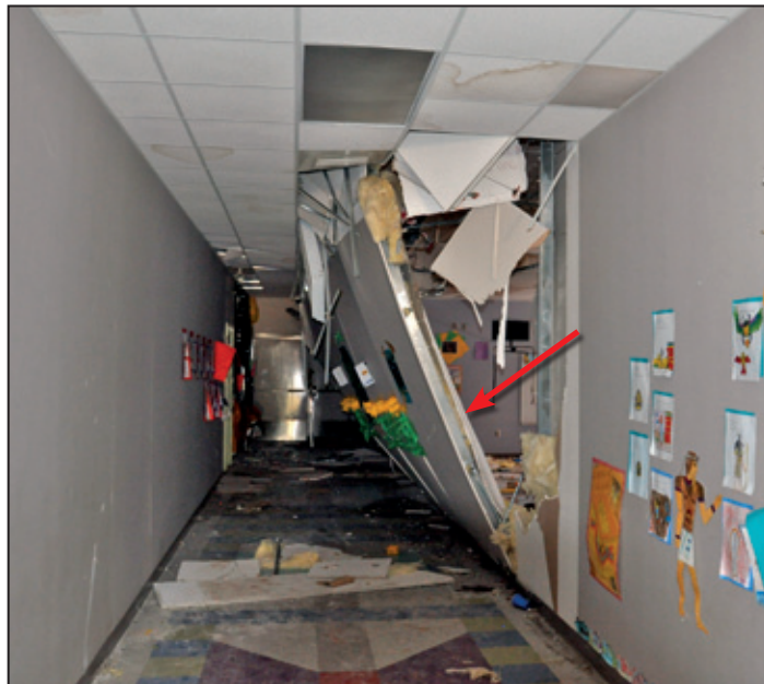
Figure 6-8: Partially collapsed corridor wall (red arrow) (Tuscaloosa, AL)
