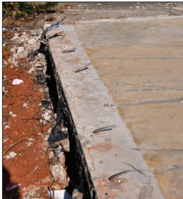
Figure 6-22: Rebar extending out of the slab at the multipurpose room end wall (Tuscaloosa, AL)
