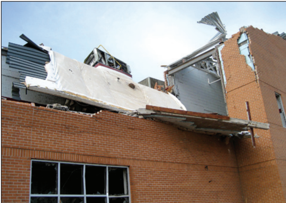
Figure 6-52: Collapse of the exterior brick veneer/reinforced CMU wall and roof assembly into the corridor at the north end of the north classroom wing (Joplin, MO)
