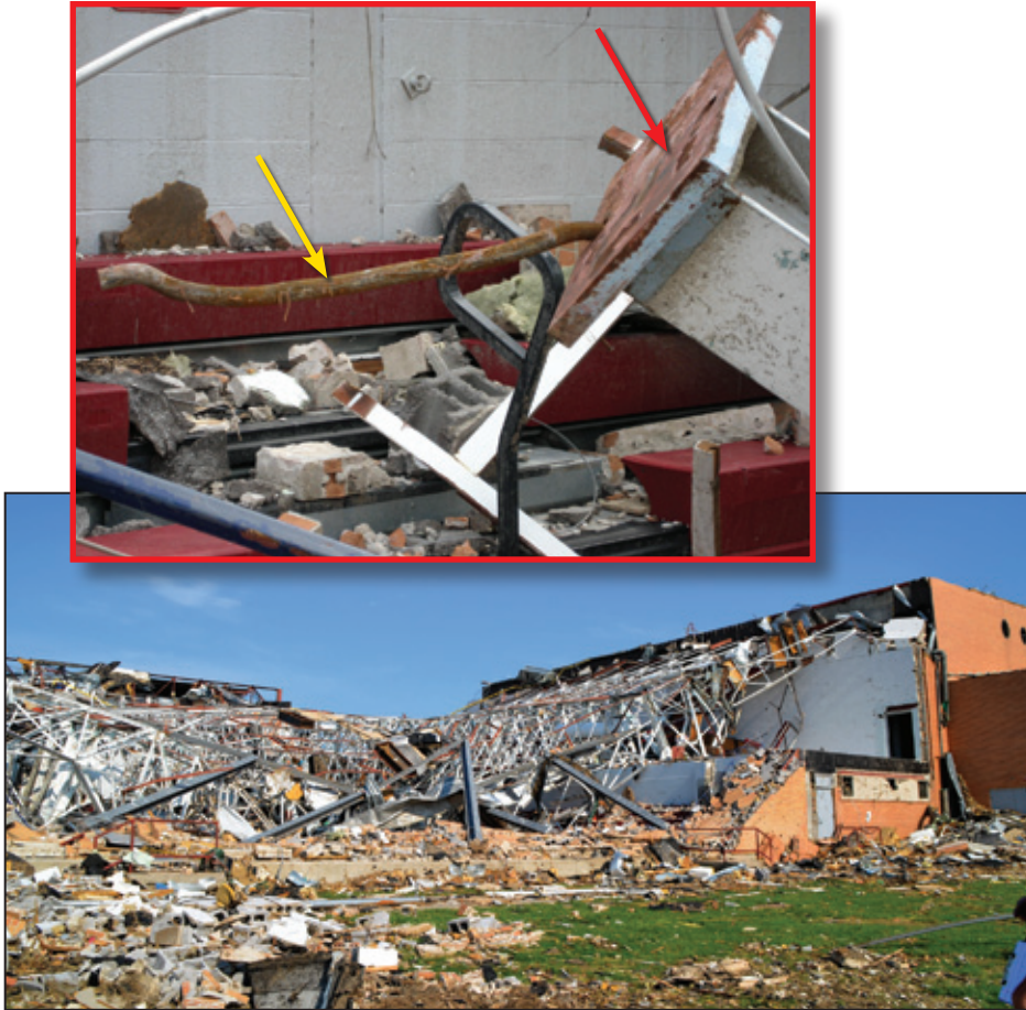
Figure 6-54: View of the collapsed gymnasium. The inset shows the base plate (red arrow) and an anchor bolt (yellow arrow) that connected the girder support column to the pilaster (Joplin, MO).
