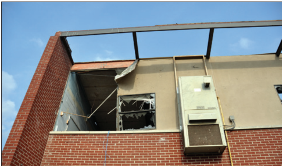
Figure 6-38: EIFS wall failure, glazing damage, and roof deck blow- off (Ringgold, GA)
