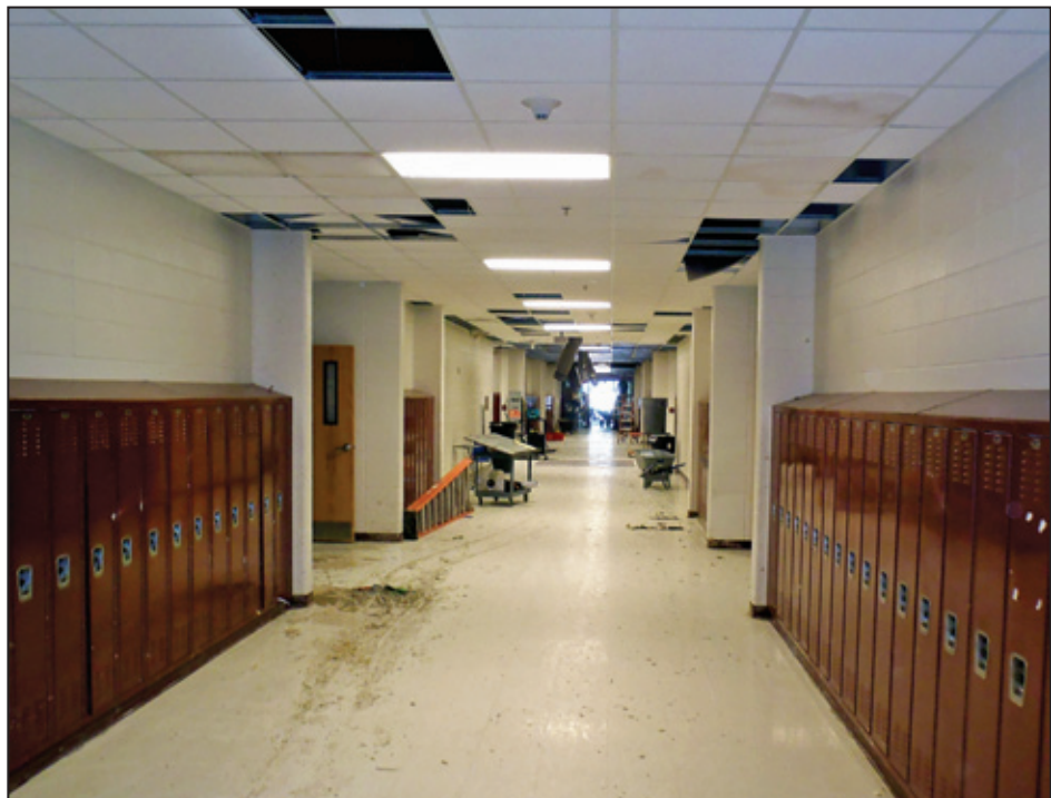
Figure 6-47: View of rain infiltration damage in a school corridor (Joplin, MO)
