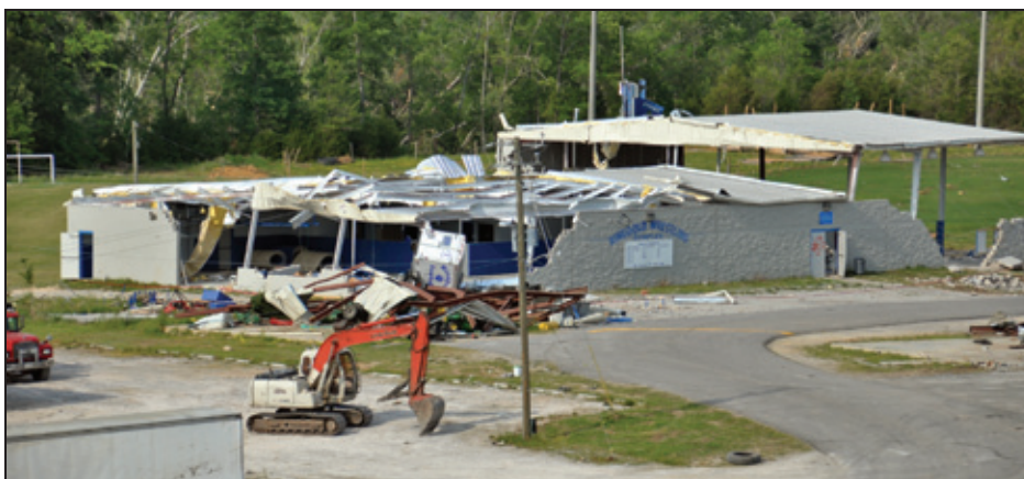
Figure 6-32: At the wrestling facility, most of the metal roof panels were blown off, much of the steel framing was damaged, and a portion of the unreinforced CMU wall collapsed. This facility was subsequently demolished (Ringgold, GA).
