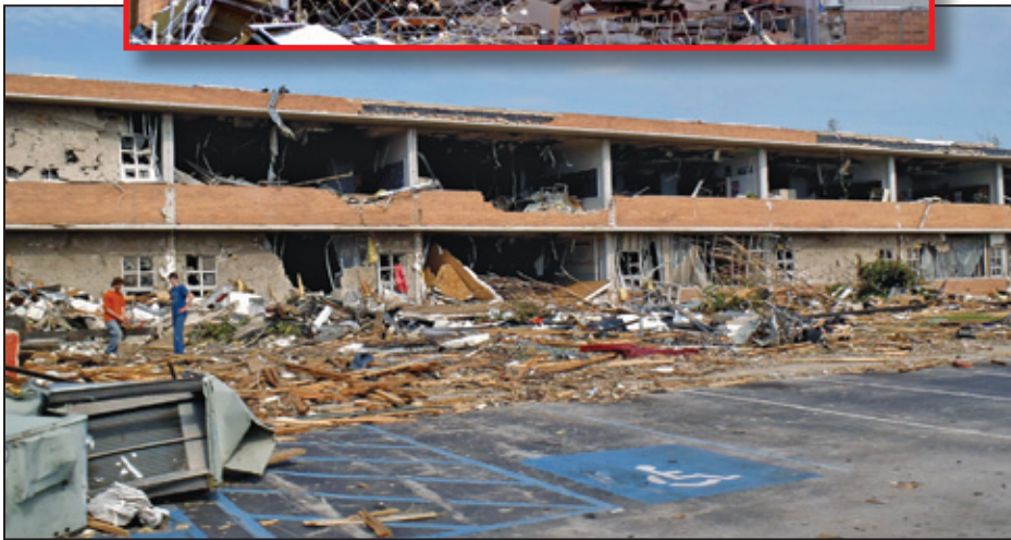
Figure 6-51: North classroom wing. The inset shows a close-up of the opposite side of the wing (Joplin, MO).
