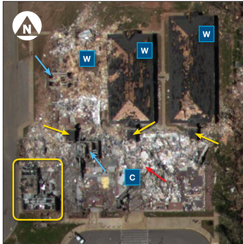
Figure 6-4: Area shown in yellow circle of Figure 6-3. The classroom wings are indicated by “W” and the core area by “C.” The general location of the tornado refuge areas for the two surviving wings is shown by the red arrow. Yellow arrows indicate remnants of corridors between the core and wings. The blue arrows indicate restroom remnants. The yellow box indicates kitchen remnants (Tuscaloosa, AL).
