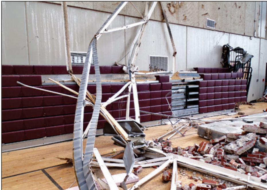
Figure 6-45: Roof truss and wall debris on the gymnasium floor (Joplin, MO)
