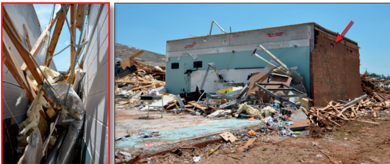
Figure 6-10: The reinforced CMU walls around the restroom were left standing, but the rooms were littered with debris (as shown in the inset). The wall with the brick veneer (red arrow) was an exterior wall (Tuscaloosa, AL).
