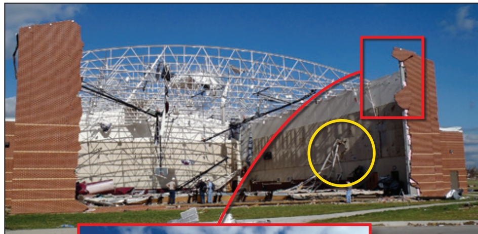
Figure 6-43: View of the gymnasium. The red box in the inset shows where the truss was attached to the wall. The yellow circle indicates the end of the collapsed truss shown in Figure 6-45 (Joplin, MO).
