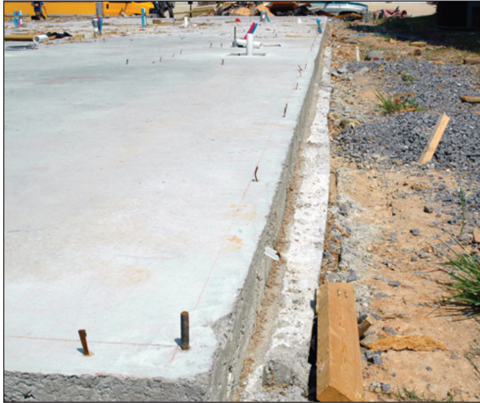
Figure 10-2: Lack of anchor bolts on recently constructed slab foundation in Jefferson County, AL. Note that an anchor bolt is installed at the corner, but cut nails are installed elsewhere.
