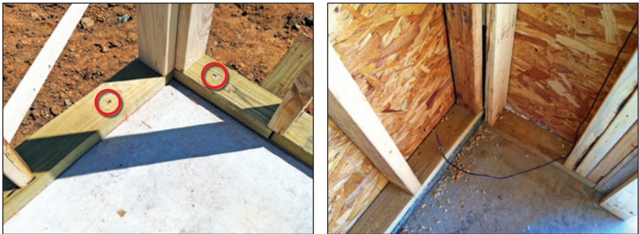
Figure 10-1: Concrete nails (red circles in left photograph) used in lieu of anchor bolts (absent in both photographs) on residential buildings under construction in the City of Tuscaloosa, AL, after the 2011 tornadoes
